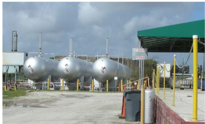
Current propane retail facility
