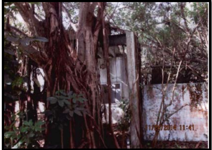
Structures of the old treatment plant overtaken by vegetation
