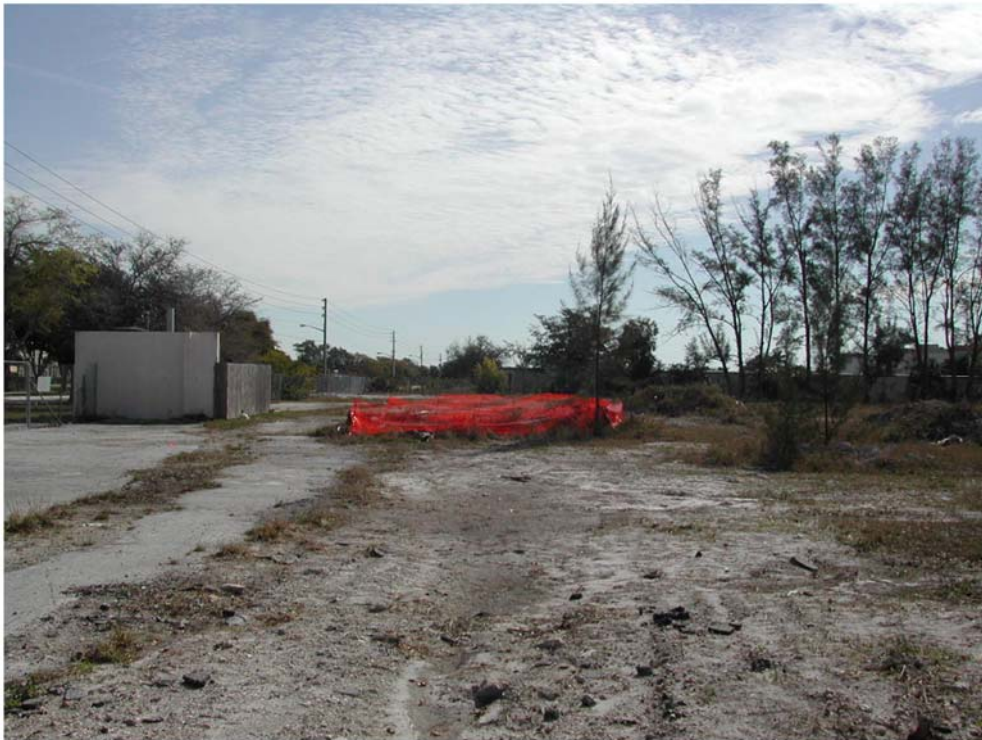
Above: The Pan American Brownfield Site in Coral Springs. The compound for the pump-and-treat remediation system is seen on the left.
