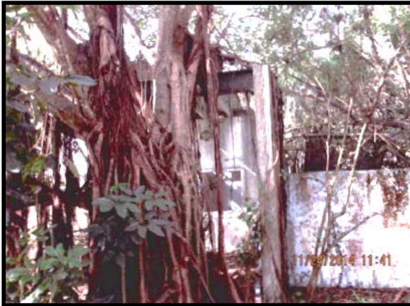
Structures of the old treatment plant overtaken by vegetation
