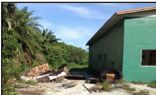
Dumping near former maintenance building
