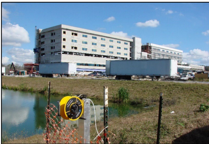
Left: Monitoring groundwater levels after soil removal and groundwater treatment. Below: Current hospital construction
