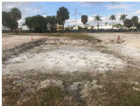
Photograph 2. View towards the north showing the SS-1 Excavation (still opened) in the northern portion of the subject site.
