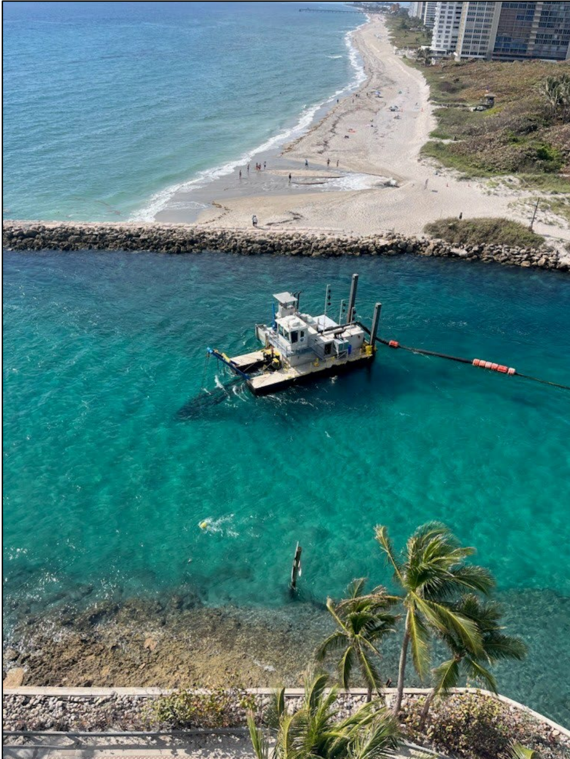
Figure 13: Boca Raton Inlet with City dredge bypassing sand south of the inlet. Photo courtesy of the City of Boca Raton - Zach Bihr, March 2024.
