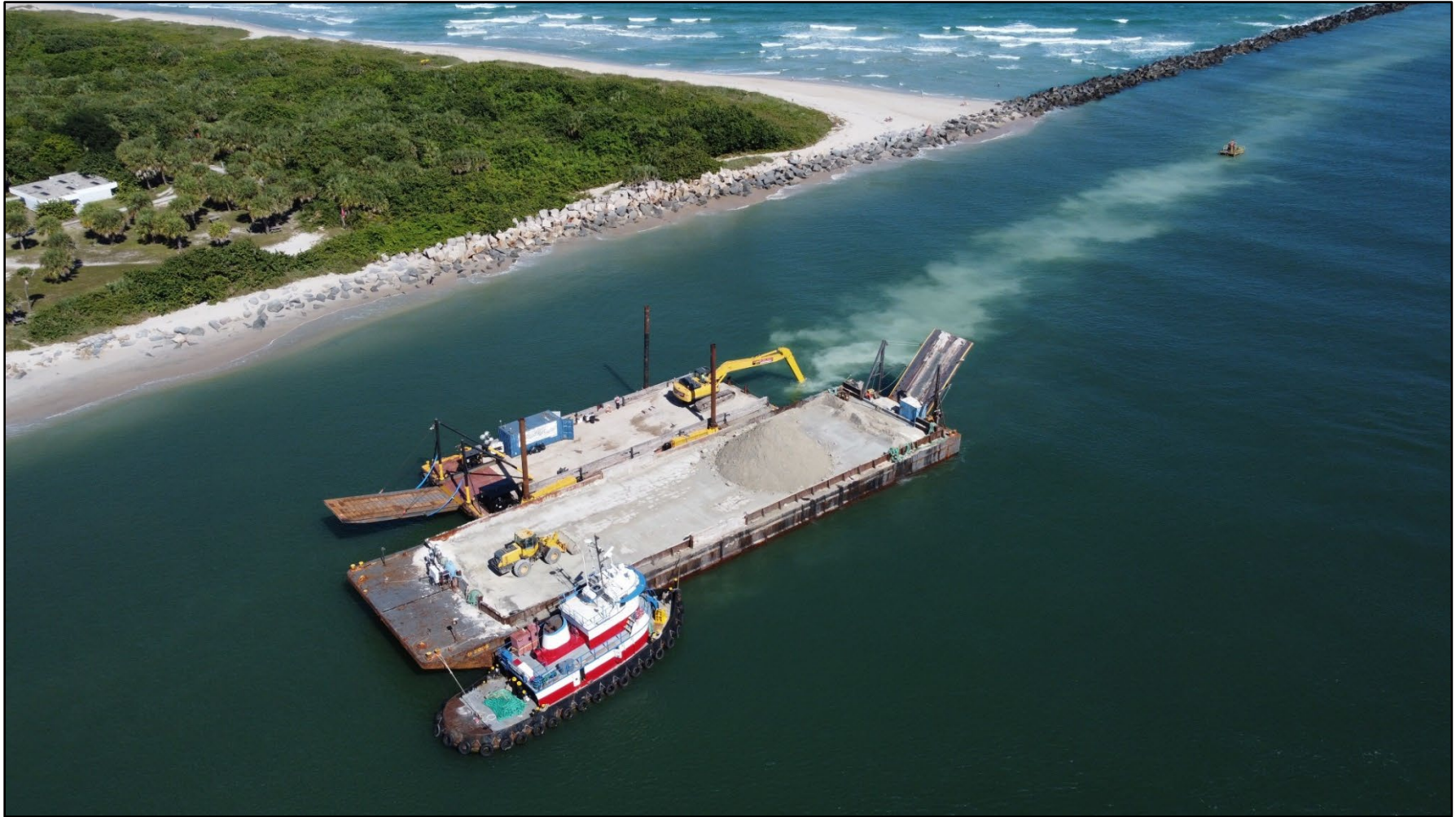
Figure 7: Ahtna Marine and Construction with a barge and backhoe within Ft. Pierce Inlet constructing the inlet sand trap. Photo courtesy of Joshua Revord project manager with St. Lucie County, November 2021.
