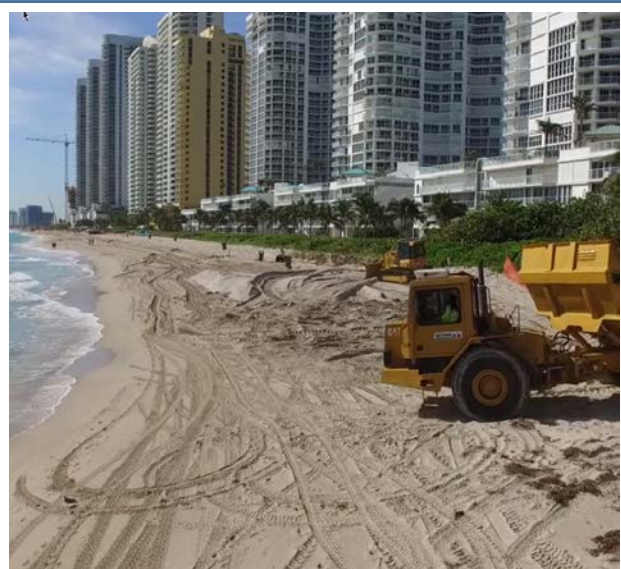
Construction of the 2017 Sunny Isles - Dade County Shore Protection Project. Photo courtesy of the U.S. Army Corps of Engineers.
