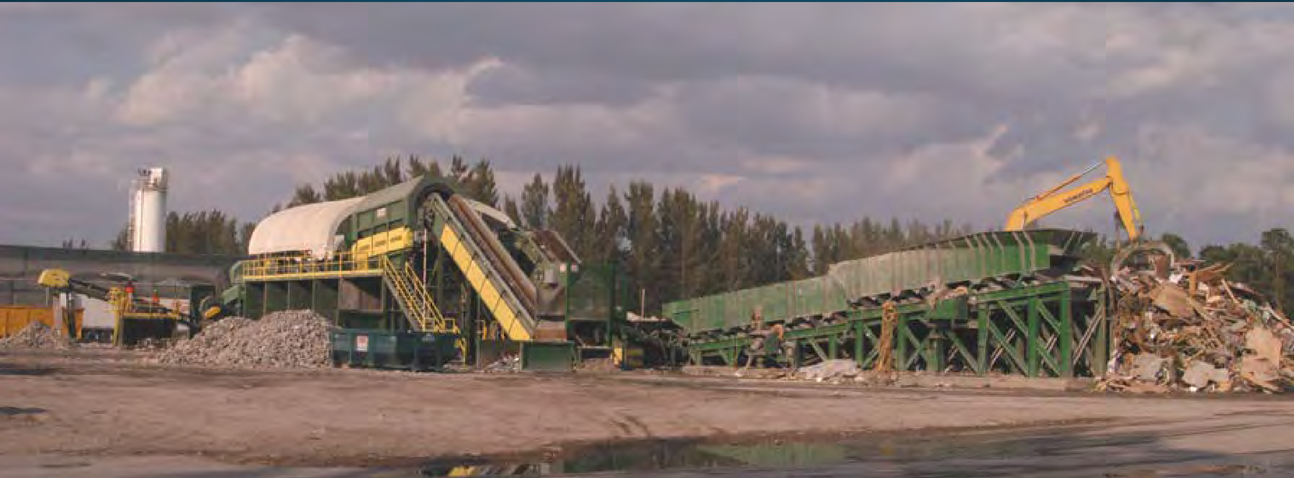
Mixed C&D Processing Facility
