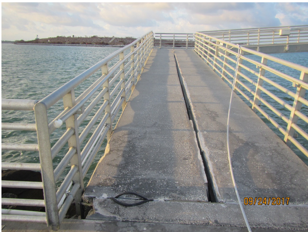
Figure 35. Jetty Park fishing pier damage where concrete deck slabs were separated, R1.
