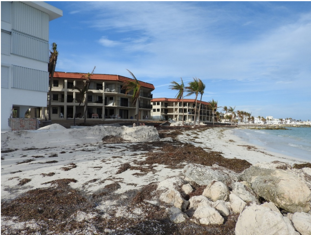
Figure 69. Major beach erosion, Key Colony Beach.
