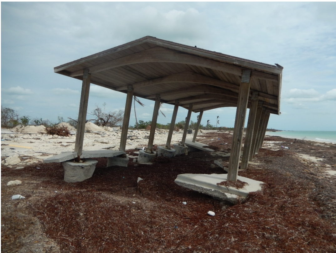
Figure 87. Middle beach pavilion and parking lot destroyed, Sandspur Beach.
