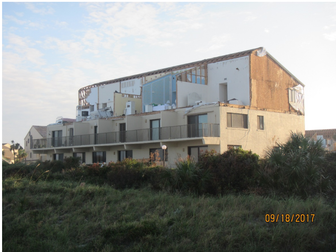
Figure 18. One of four condominiums destroyed by rain band tornado, Matanzas Shores, R192.4.
