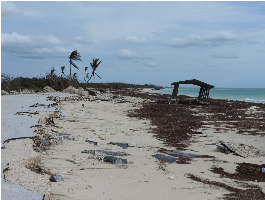
Figure 86. Sandspur Beach parking lot destroyed.
