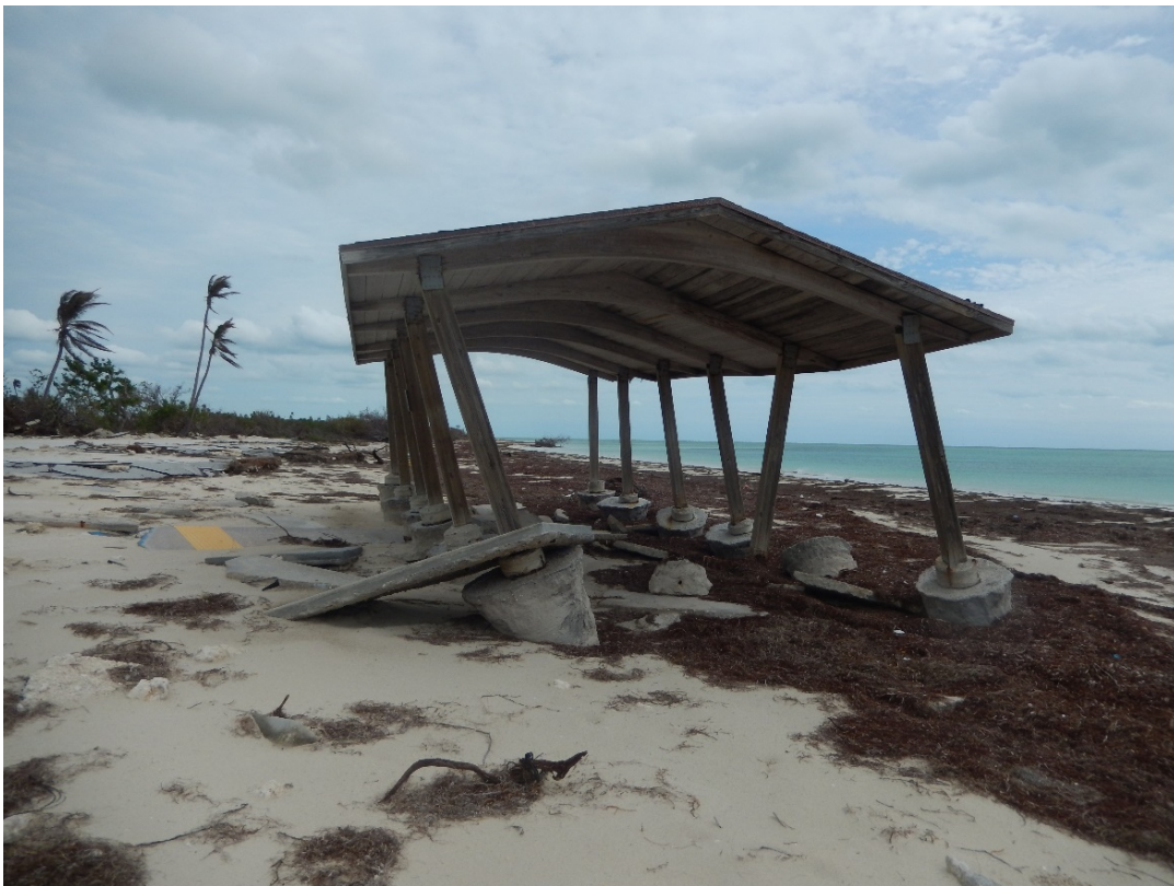
Figure 89. Eastern pavilion structure and parking lot destroyed, Sandspur Beach.
