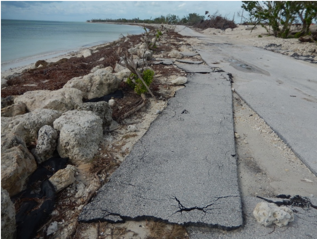
Figure 83. Bahia Honda State Park road and revetment damage.
