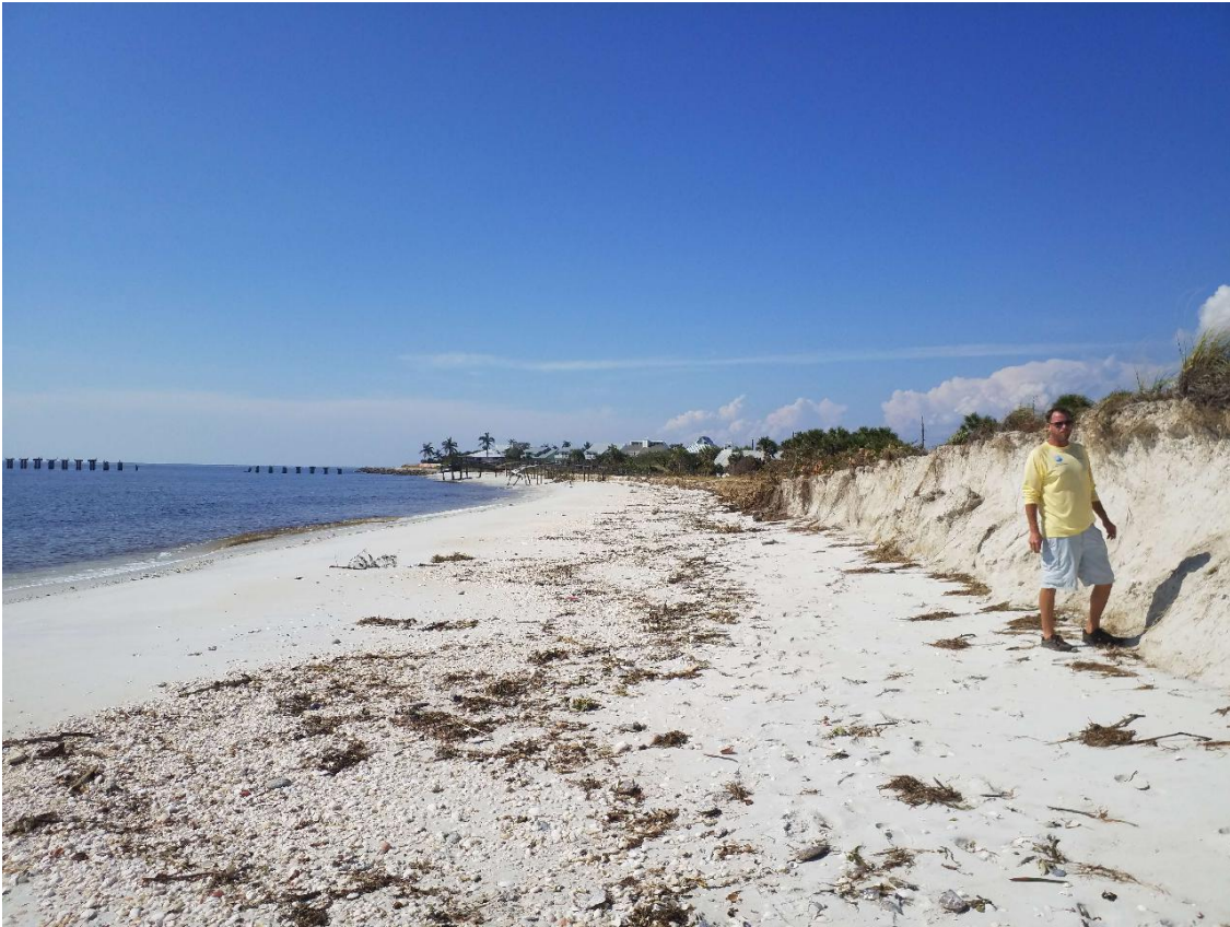
Figure 44. Erosion and damage to dune walkovers at the southern end of Gasparilla Island State Park, R26.
