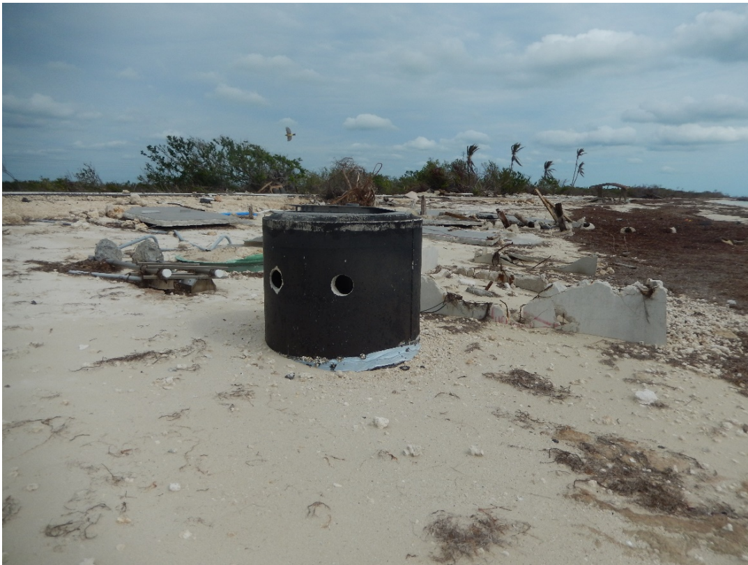
Figure 88. Bathhouse structure totally destroyed, Sandspur Beach.
