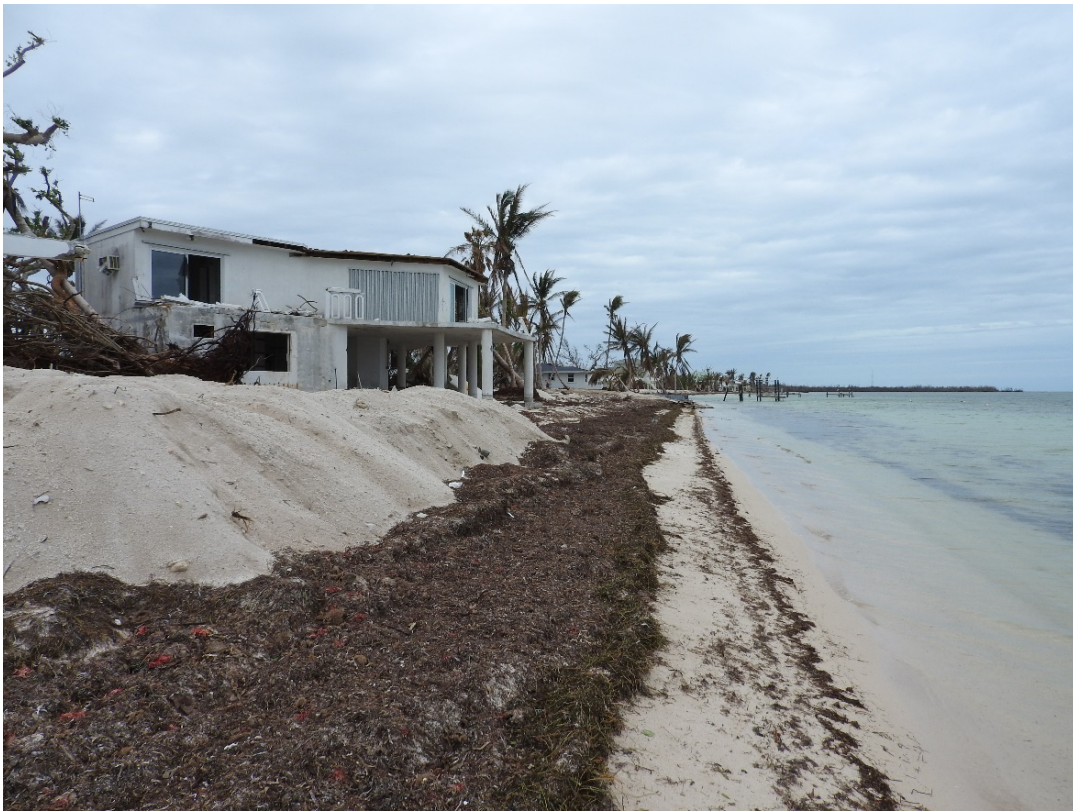
Figure 90. Major erosion and structural damage along Long Beach, Big Pine Key.
