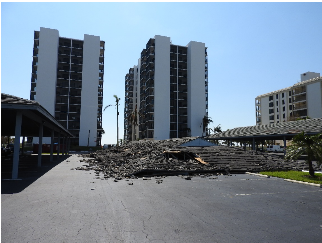
Figure 50. Collapsed parking garage structure at Fort Myers Beach near R201.
