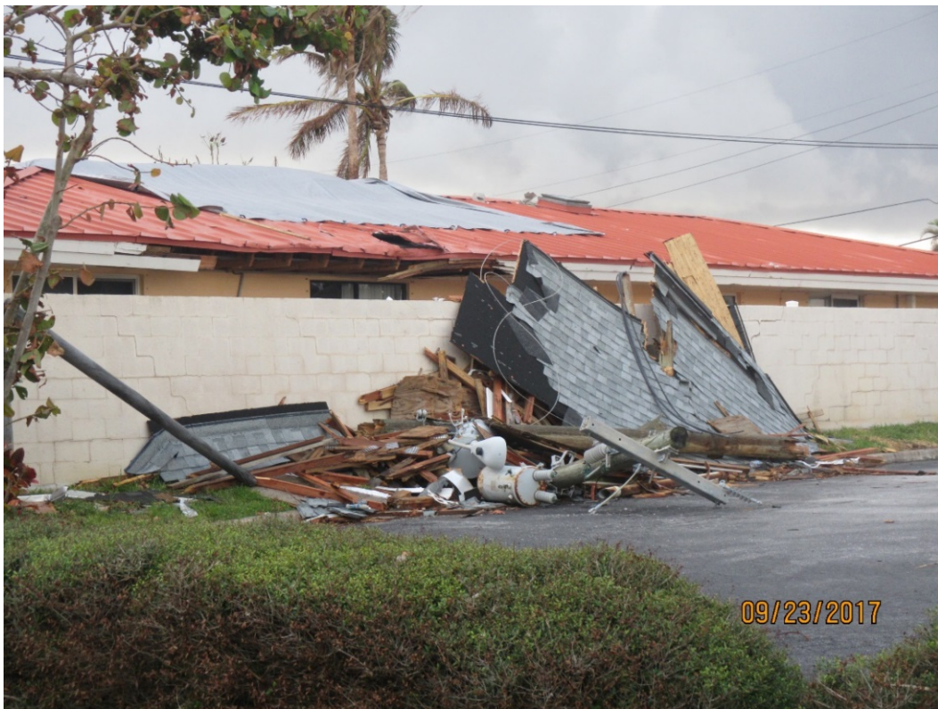
Figure 33. Condominium roof section blown across State Road A1A onto single-family dwelling by tornado at R122, Indialantic.
