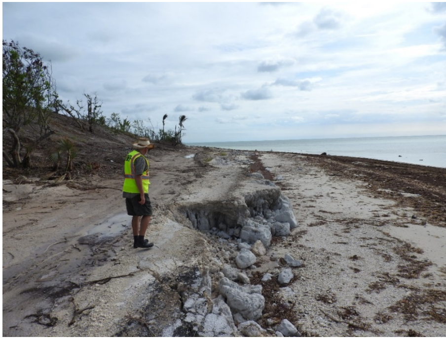
Figure 81. Severe beach erosion and road destroyed at west end of Bahia Honda Key.
