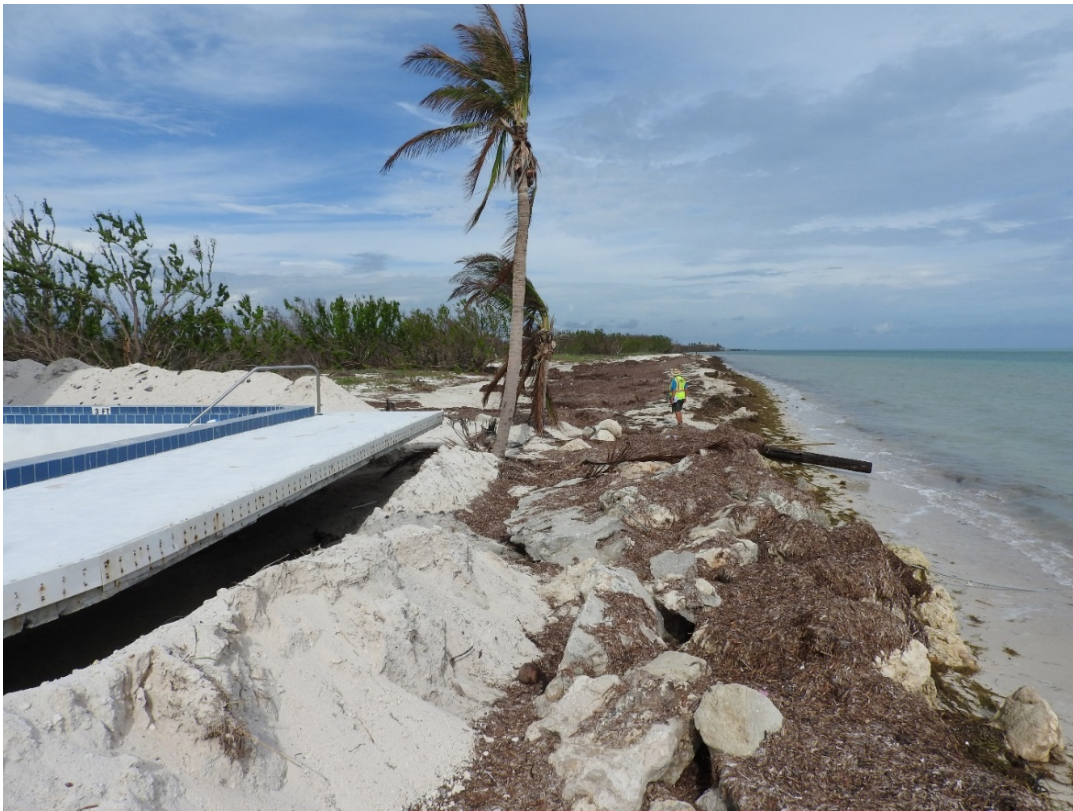
Figure 68. Damaged revetment and undermined pool at Coco Plum Beach.
