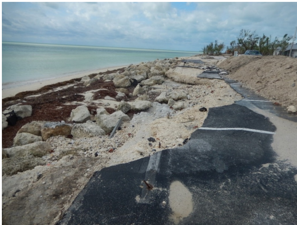
Figure 82. Revetment, access walkways, parking lot and all infrastructure for Loggerhead Beach was destroyed.
