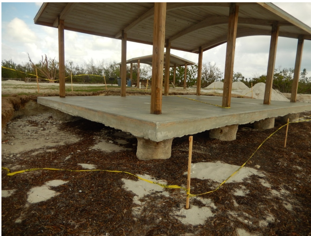
Figure 66. Undermined pavilion at Curry Hammock State Park.
