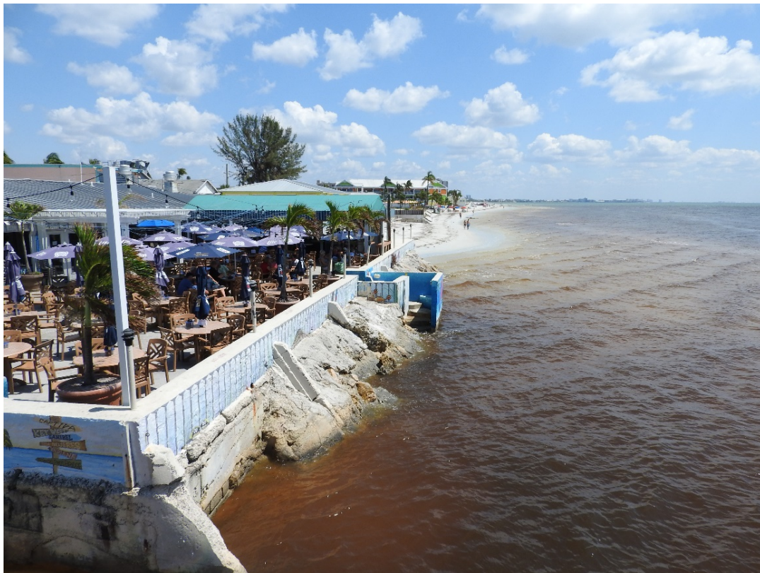
Figure 48. Erosion south of the Fort Myers Beach Pier near R180.
