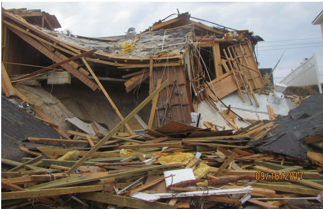
Figure 17. Seawall failure and single-family dwelling destroyed at R89.4, South Ponte Vedra.
