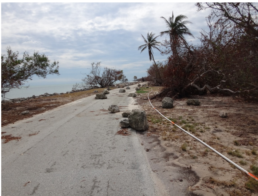
Figure 63. The park road in Long Key State Park with overwash of revetment boulders.
