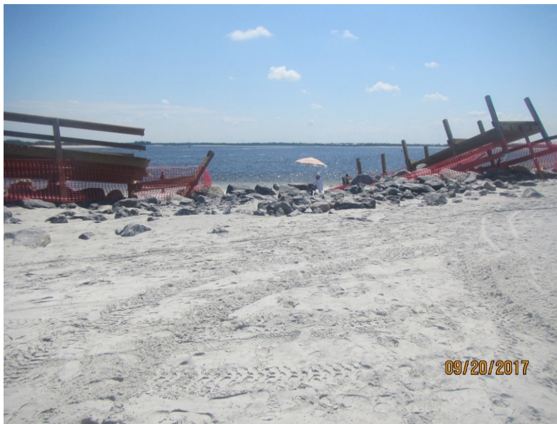
Figure 28. Major damage to north jetty and boardwalk at Ponce de Leon Inlet, R148.
