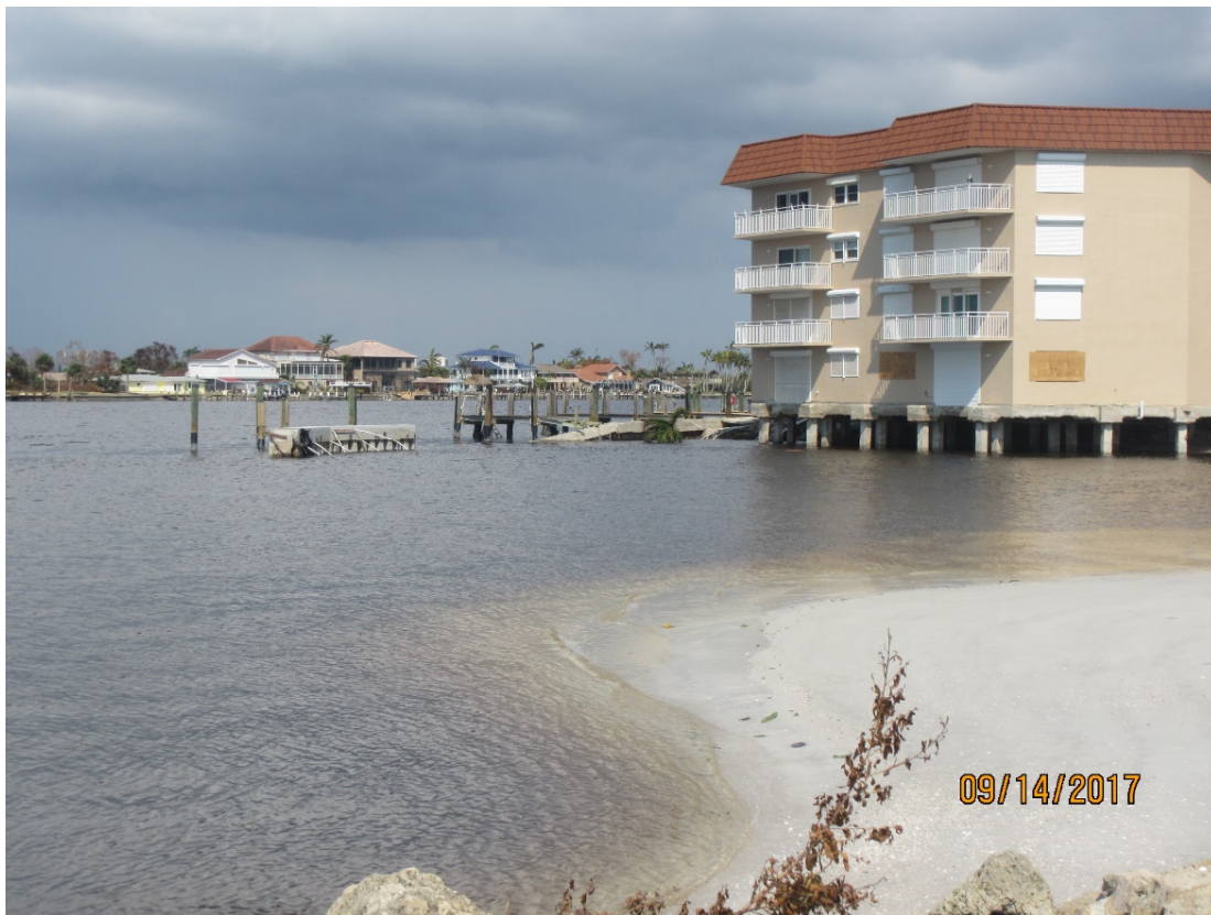
Figure 42. Seawall destroyed and condominium undermined in Big Marco Pass near V310.
