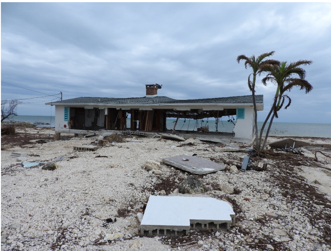
Figure 93. Single-family dwelling destroyed, Long Beach, Big Pine Key.
