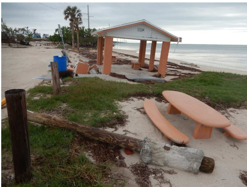
Figure 77. Monroe County park damages on Little Duck Key.
