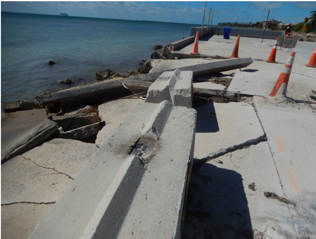
Figure 97. Bertha Street end seawall damage, Key West.
