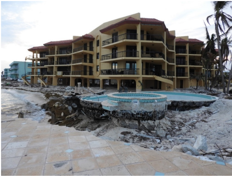
Figure 71. Major damage to shoreline development, Key Colony Beach.
