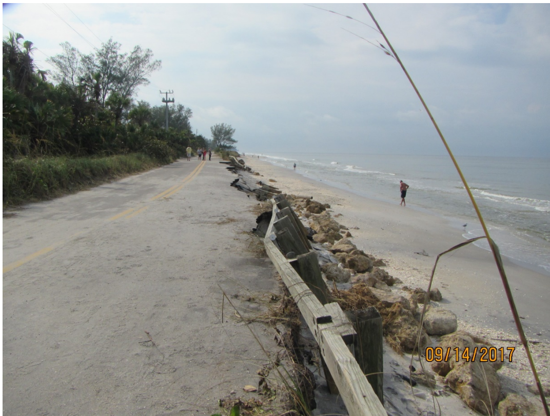
Figure 55. Dune erosion that damaged Manasota Key Road near R175.
