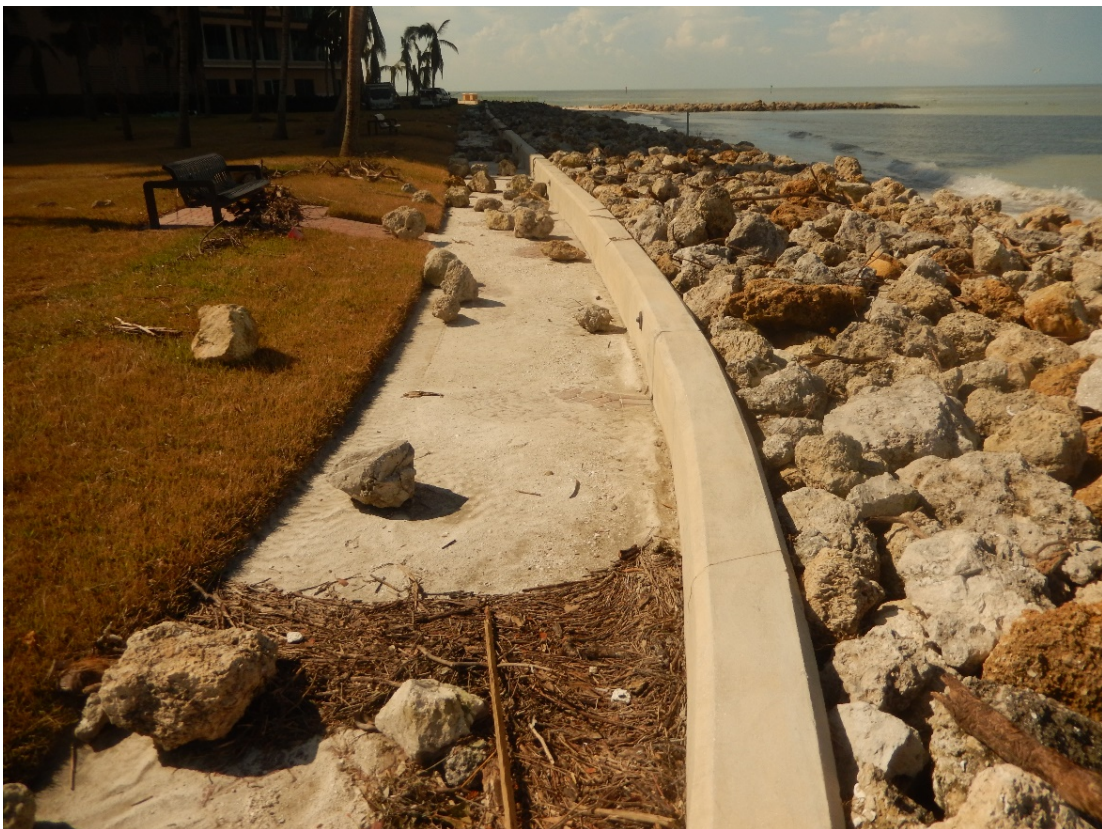
Figure 41. South Marco Island revetment damage near R148.
