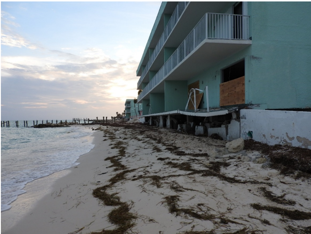
Figure 70. Building damage, Key Colony Beach.
