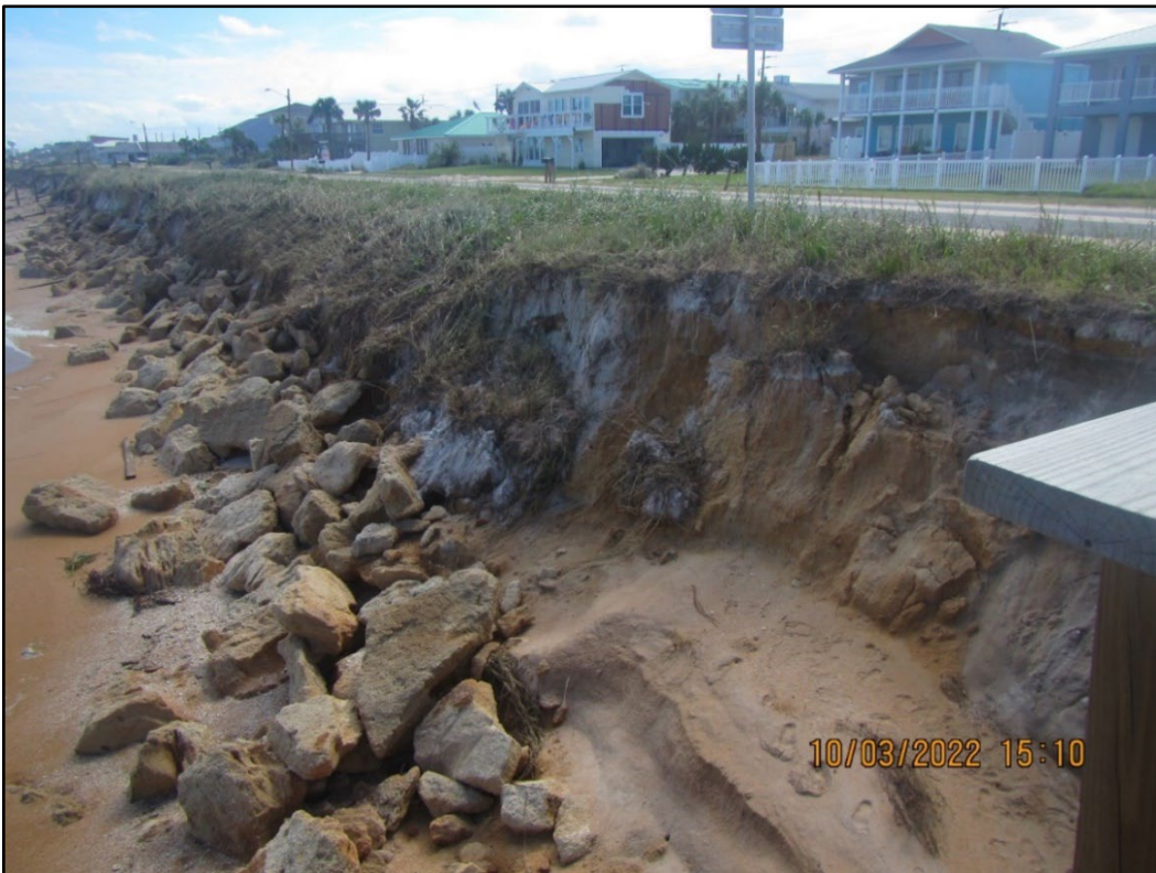
Figure 78. Major revetment damage due to Hurricane Ian south of the pier (R-80).
