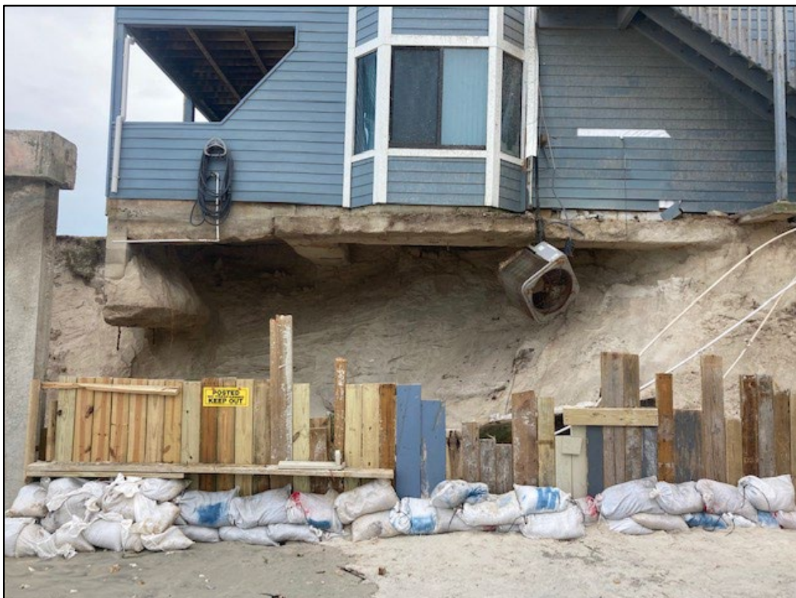
Figure 112. Multifamily dwelling in imminent danger of collapse (R131).
