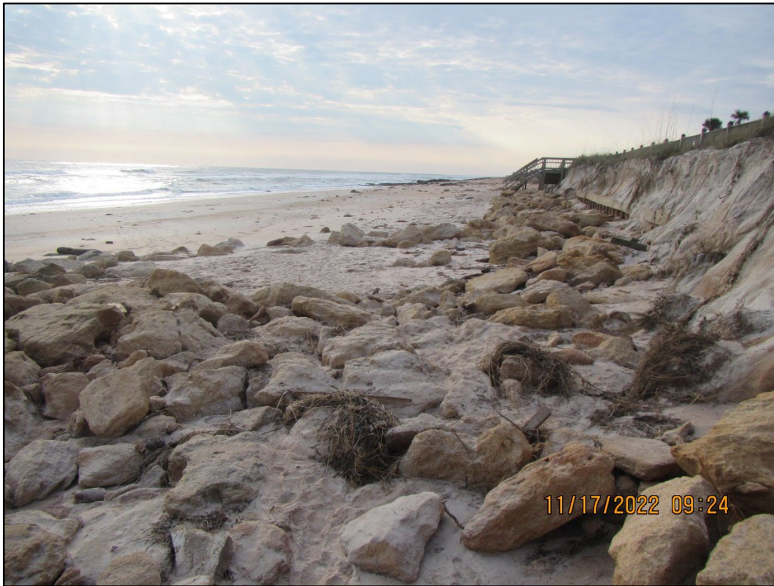
Figure 70. Major beach and dune erosion at Marineland's River to Sea Preserve (R3).
