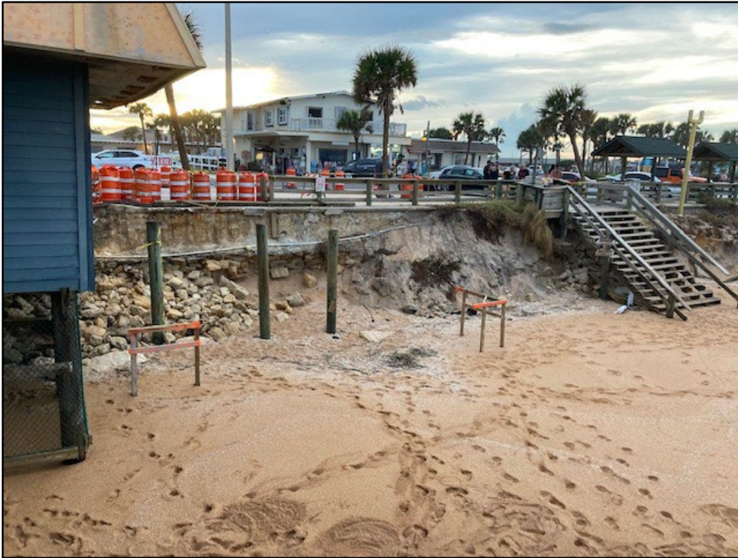
Figure 77. Major beach and dune erosion from Ian north of the Flagler Beach Pier (R-79).
