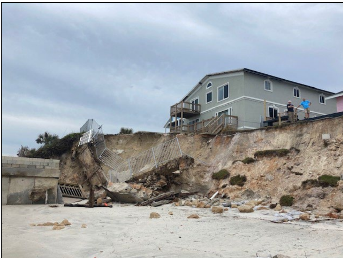
Figure 116. Multifamily dwelling in imminent danger following severe dune erosion.
