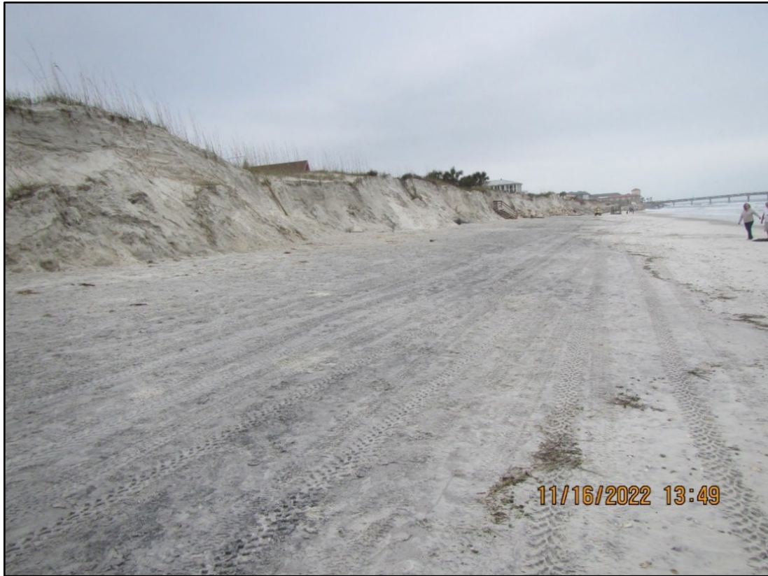
Figure 62. Major beach and upland erosion at St. Augustine Beach, looking north to pier (R-144).
