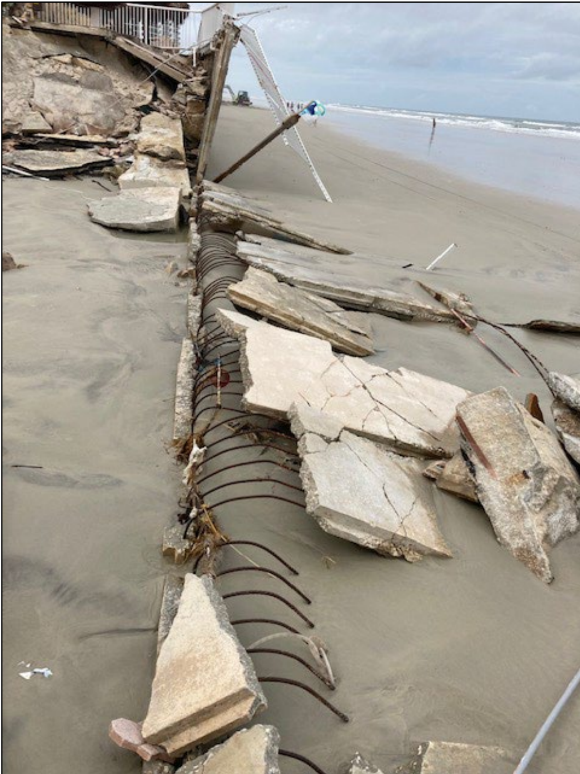
Figure 87. Seawall failure due to inadequate panel thickness of only 4 inches.
