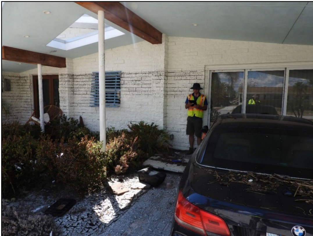
Figure 46. High-water mark on a bay-side single-family dwelling on Clearview Blvd. (R-201).
