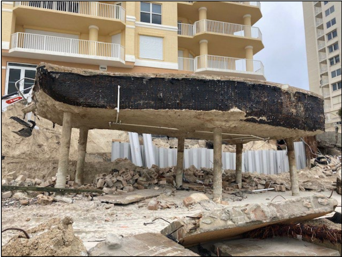
Figure 117. Undermined pile-supported pool in Volusia County.
