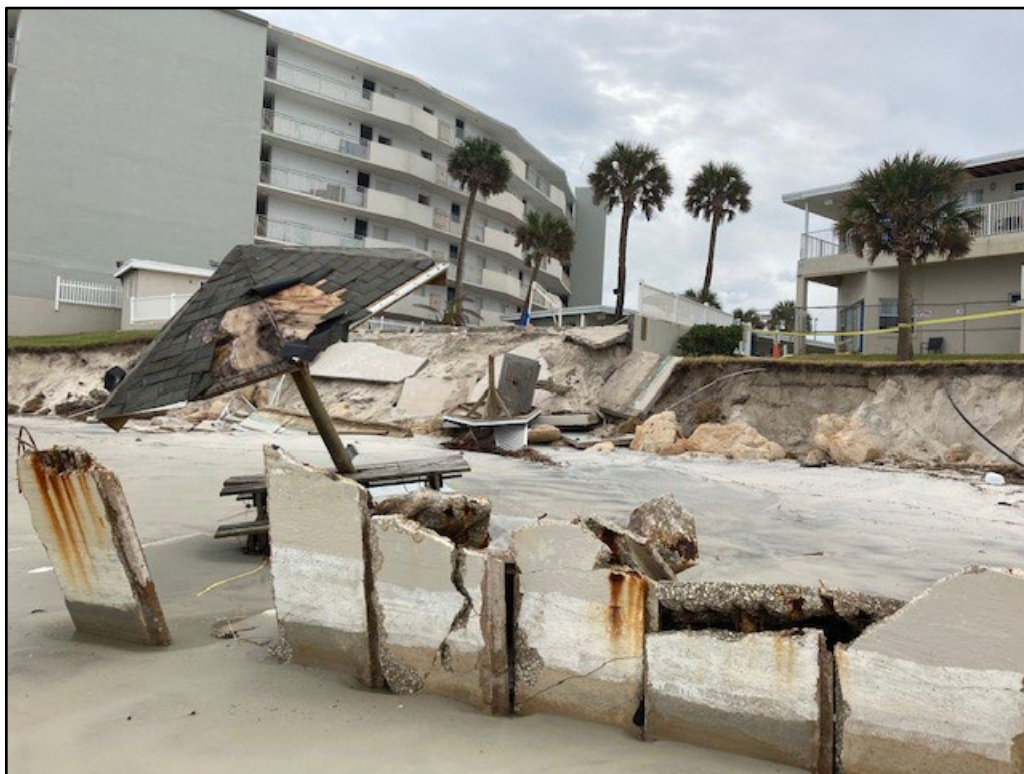
Figure 91. Old seawall destroyed by wave impact loads resulting in substantial loss of property in Daytona Beach Shores (R99).
