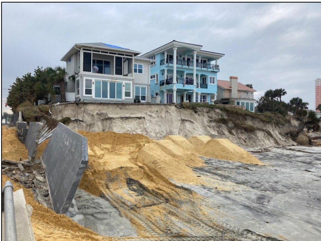
Figure 120. More threatened houses following severe erosion in Daytona Beach Shores (R-103).
