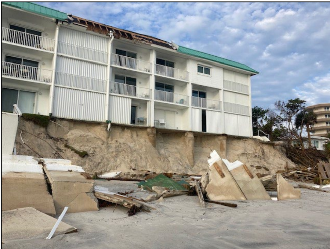
Figure 106. Condominium in imminent danger with roofing and siding damages.
