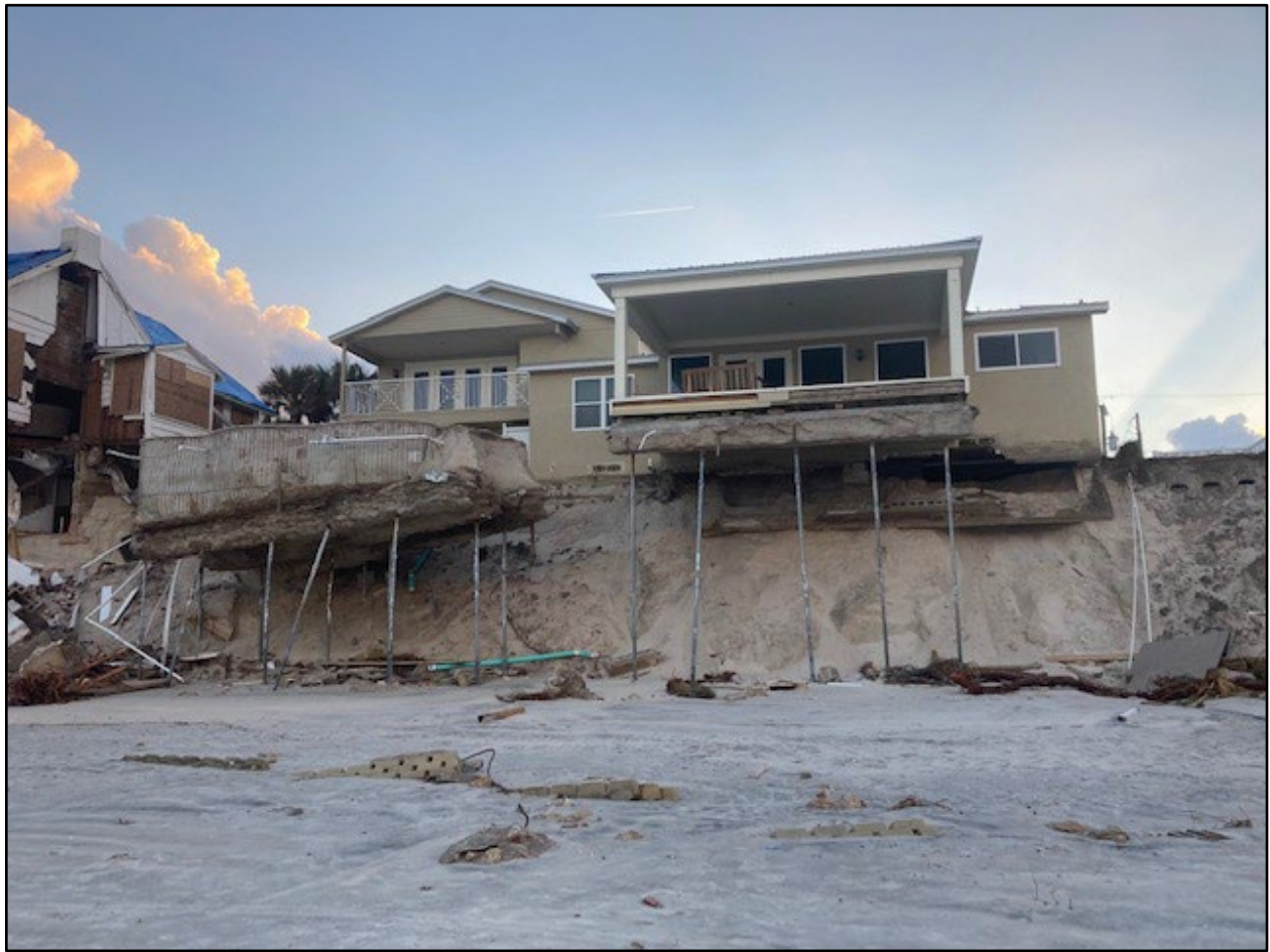
Figure 103. House and pool in imminent danger from major beach and dune erosion .
