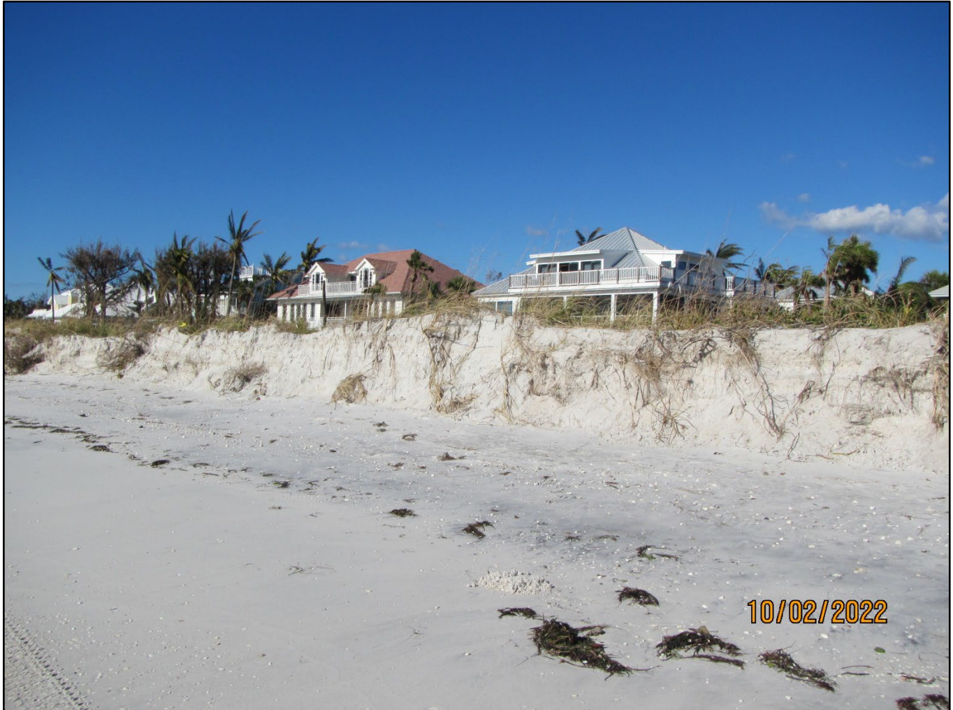
Figure 30. Condition II erosion at R-2 in Lee County near the county line between Charlotte and Lee Counties.
