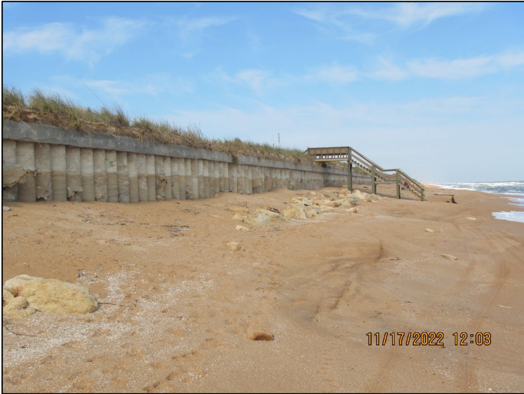
Figure 75. Major beach and dune erosion exposed the new secant wall constructed by the Florida Department of Transportation (R-66).
