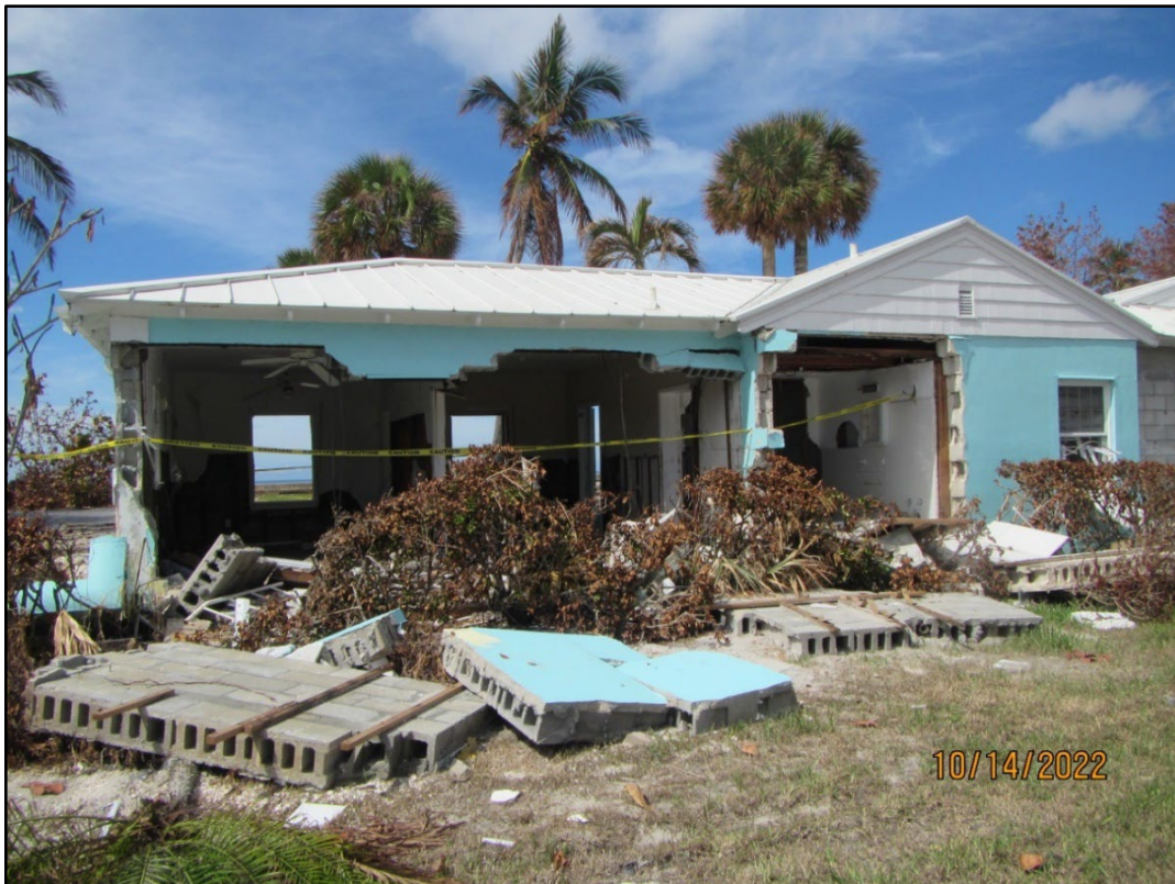
Figure 53. Single-family dwelling with storm surge damage, Naples (R-85).
