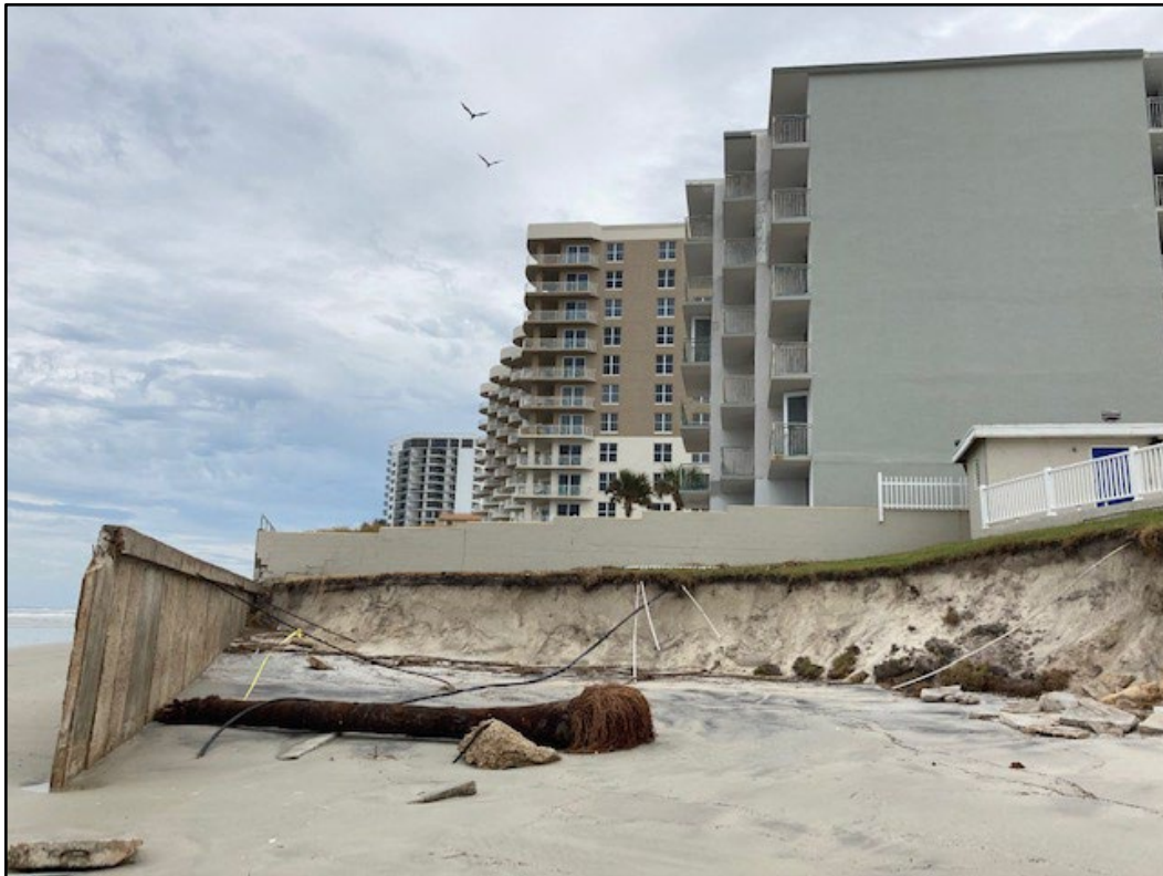
Figure 97. Substantial loss of property with seawall failure.
