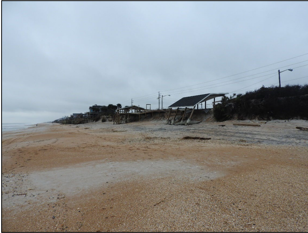
Figure 58. Major damage to a pavilion due to erosion in a county park in South Ponte Vedra (R-95).
