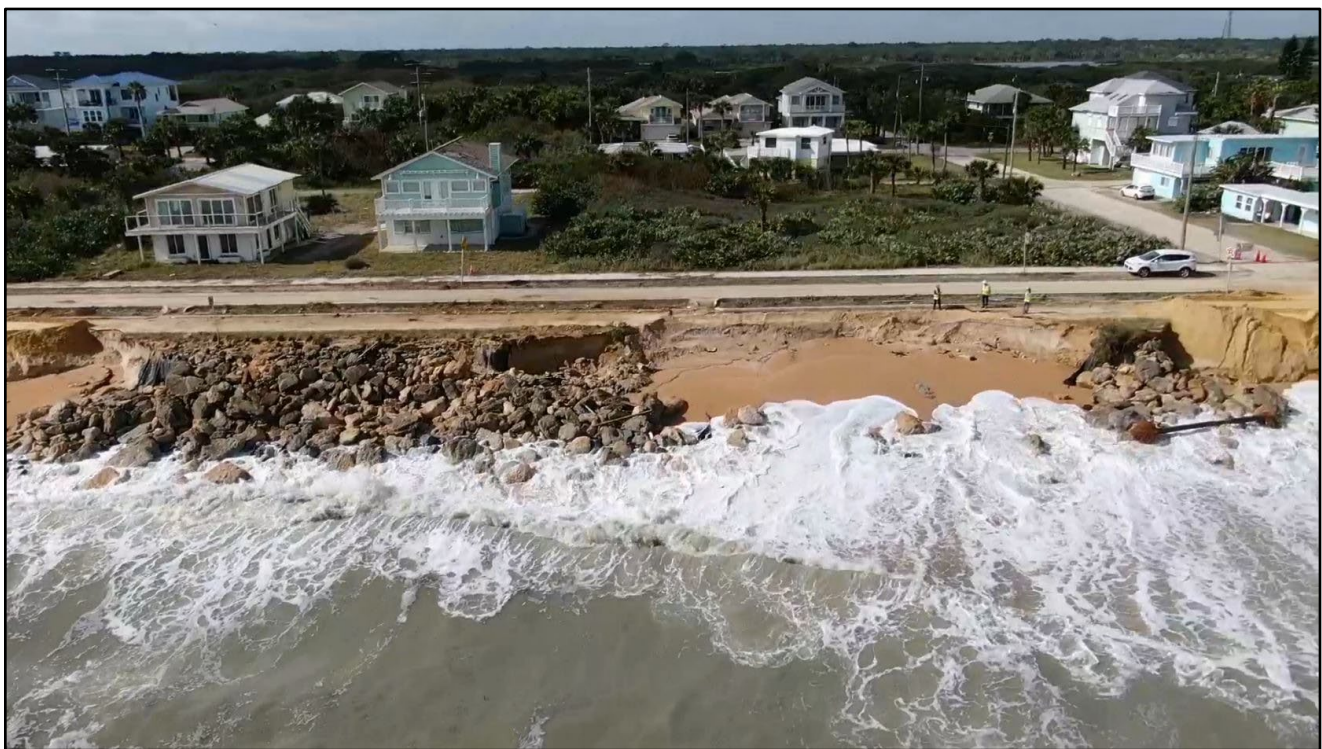
Figure 80. A1A revetment and road damage after Hurricane Nicole in Flagler Beach at 17 th Street South (R-88) [Drone footage courtesy of Olsen Associates and Flagler County].
