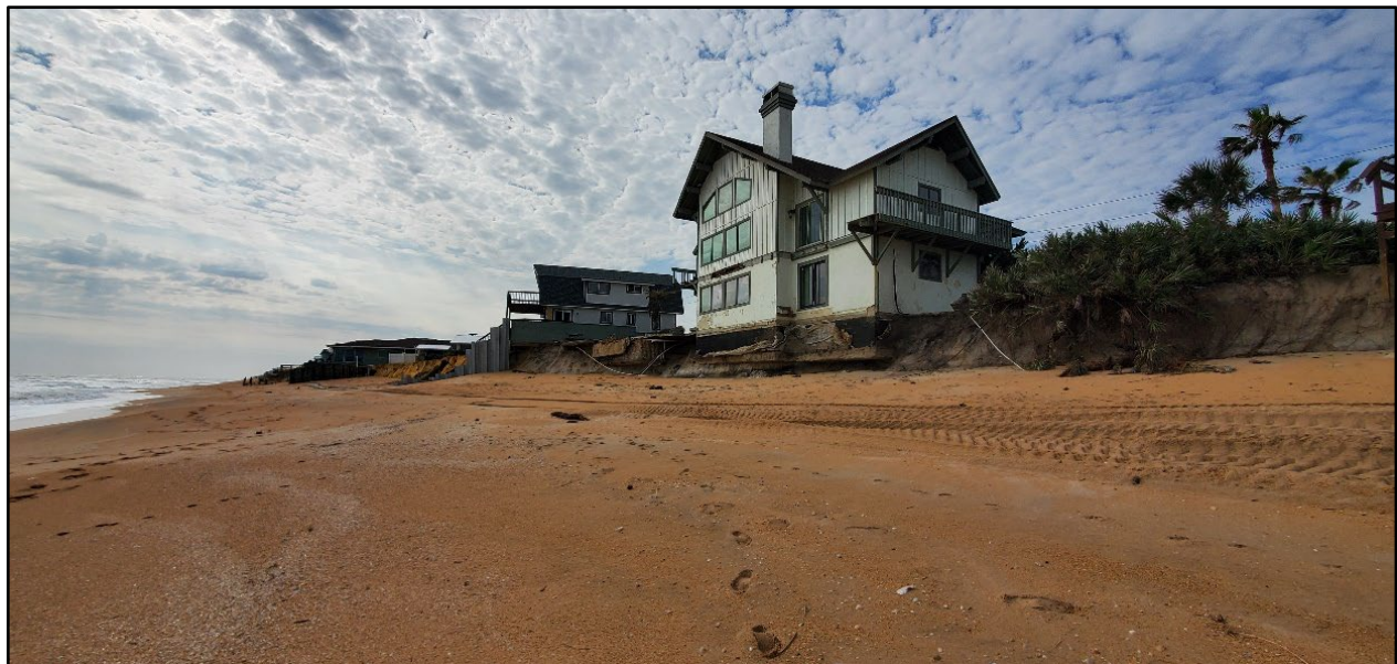
Figure 74. Single-family dwelling with first floor damage and major pool damage in Beverly Beach (R-53).
