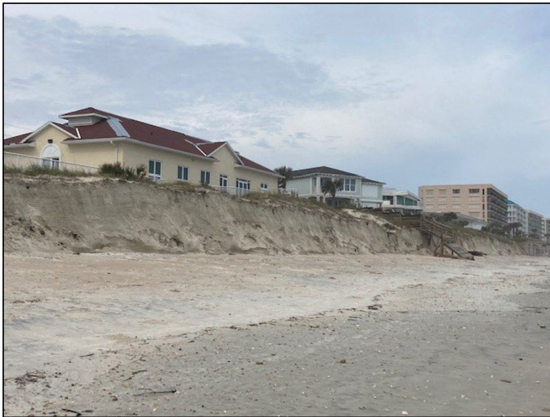
Figure 83. Severe dune erosion threatening upland properties in the Town of Ponce Inlet (R138).
