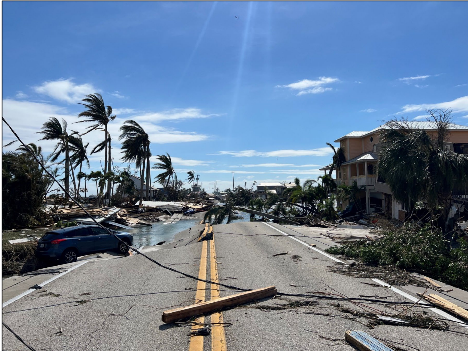
Figure 37. Pine Island causeway destroyed. Photo courtesy of Florida State University - Emergency Management and Homeland Security Program/ Florida UAS-1. Photo taken on September 29 th , 2022.
