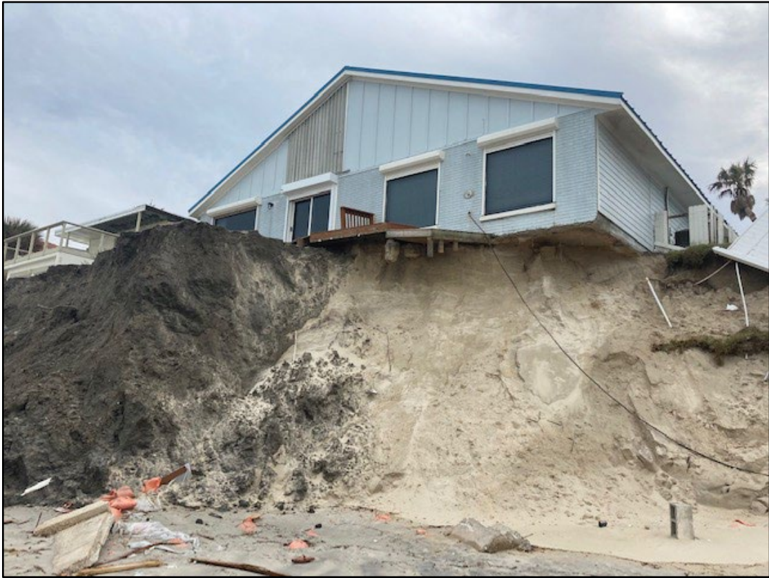
Figure 113. House in imminent danger of collapse, Wilbur-by-the-Sea, (R126).
