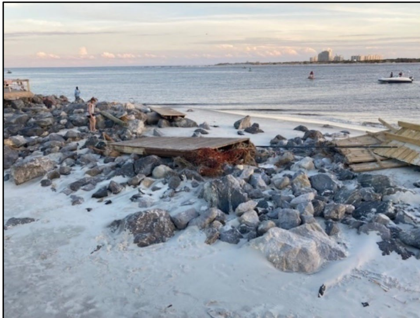
Figure 100. Damaged north jetty to Ponce de Leon Inlet (R-148).
