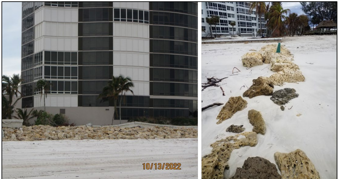
Figure 54. Concrete seawall collapsed in Naples at R-47 (left) and buried groin exposed at R-58 (right).
