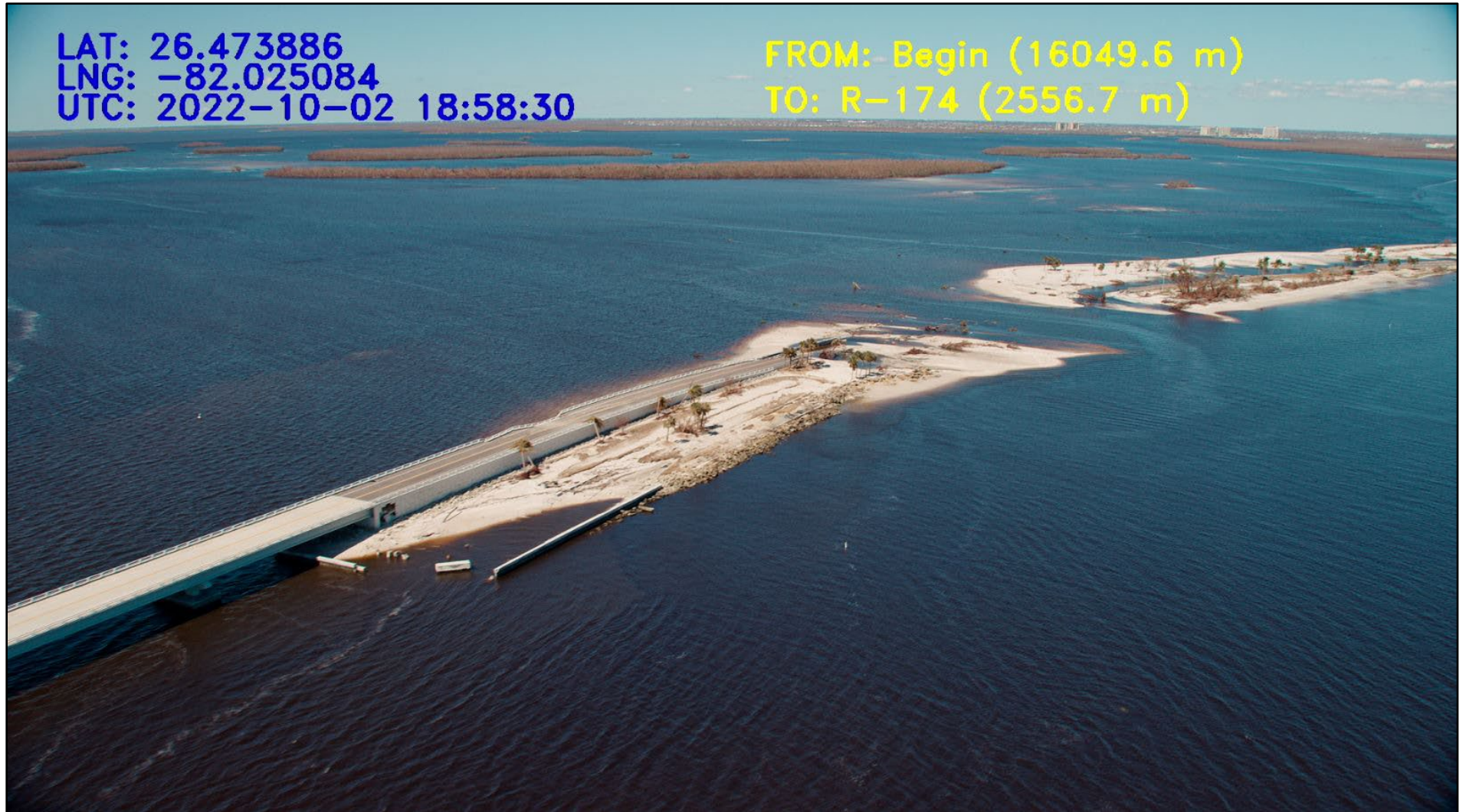
Figure 34. Sanibel Island bridge and causeway destroyed. (Image source: Active Camera Systems and Camera Copters).
