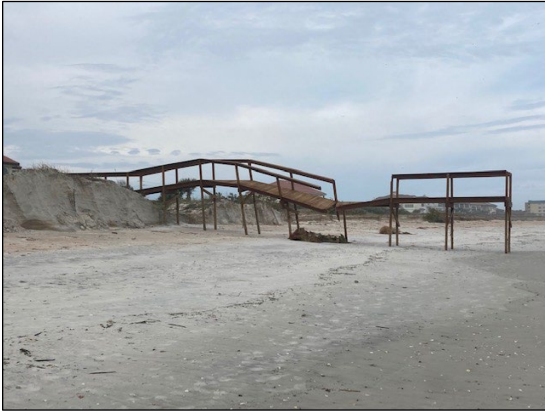
Figure 82. Major beach and dune erosion in the Town of Ponce Inlet (R147).
