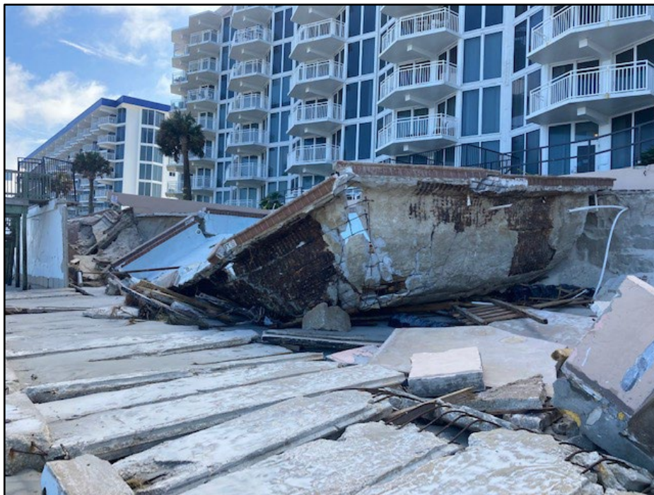
Figure 89. Seawall destroyed with inadequate pile penetration resulting in a destroyed swimming pool (R116).
