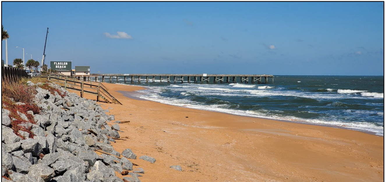
Figure 79. Flagler Beach Fishing Pier with 165 ft. of the seaward end destroyed (R-79).
