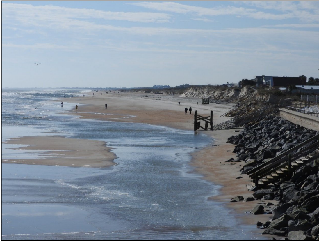
Figure 61. Major beach and upland erosion at St. Augustine Beach, looking south from pier (R-142).
