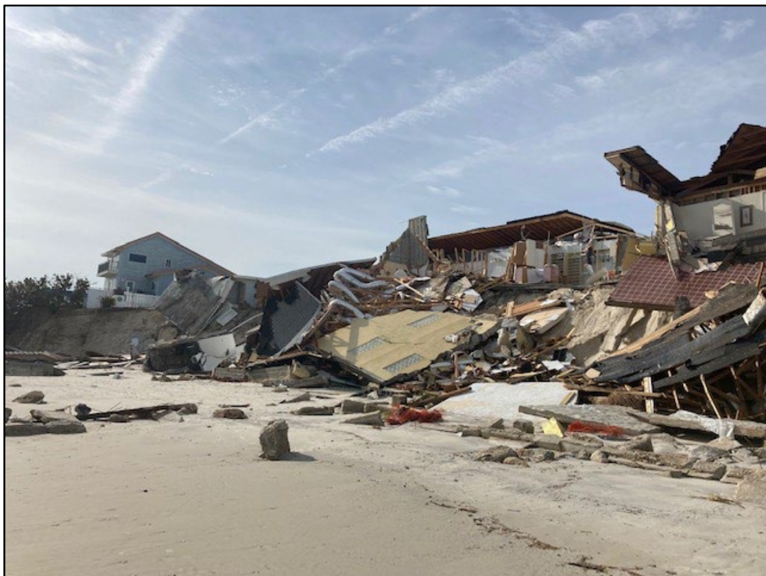
Figure 110. Homes destroyed, Wilbur-by-the-Sea (R125).
