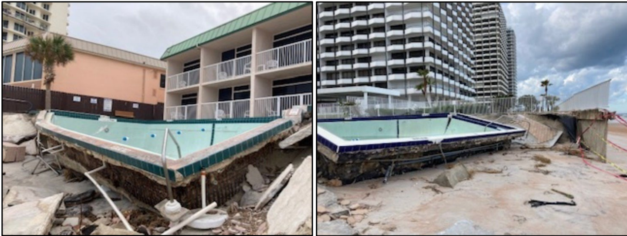
Figure 85. Swimming pools destroyed with seawall failure (R101).
