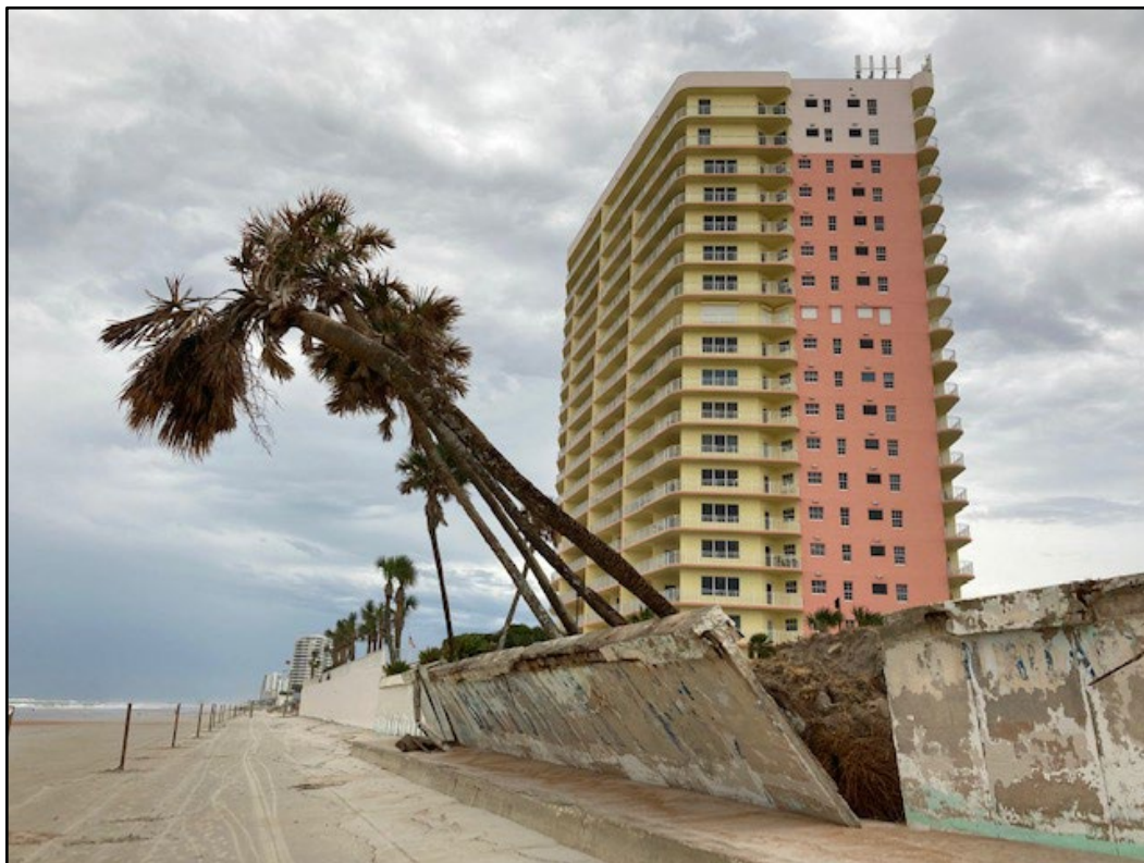
Figure 99. Inadequate seawall tie-backs, wall thickness and pile penetration (R-71.5).
