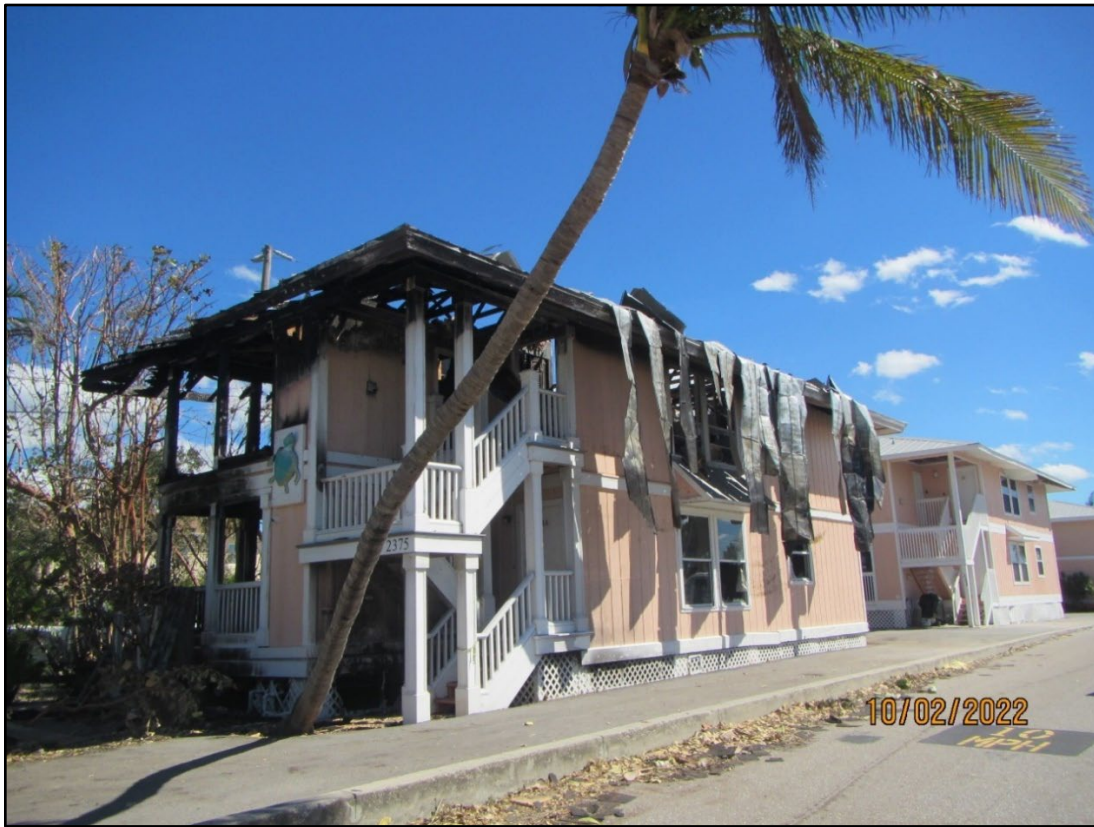
Figure 22. Multi-family dwelling destroyed by fire off Estada Street (R-8).
