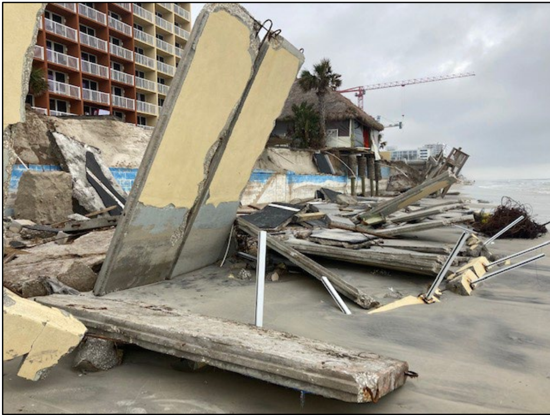
Figure 119. More seawall damage by Hurricane Nicole.
