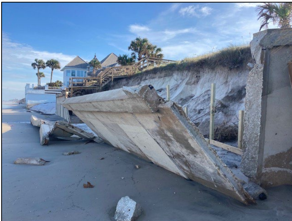
Figure 93. Seawall failure due to beach profile lowering and lack of tie-backs in Wilbur by the Sea (R124).
