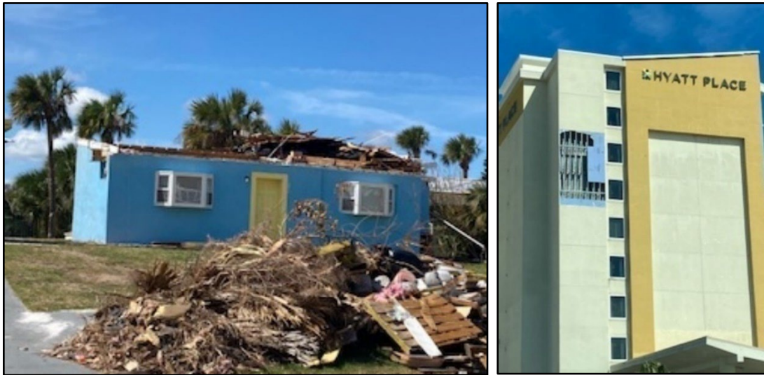
Figure 84. Roof blown off dwelling (left, R94); siding damage on hotel (right, R111).
