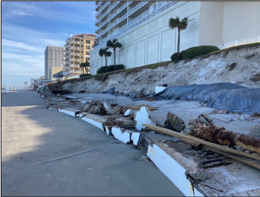
Figure 96. Catastrophic seawall failure threatens condominium in Daytona Beach Shores (R114).
