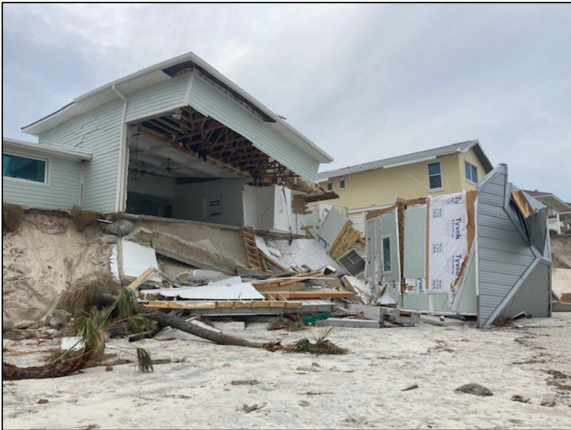
Figure 115. Partial collapse of house.
