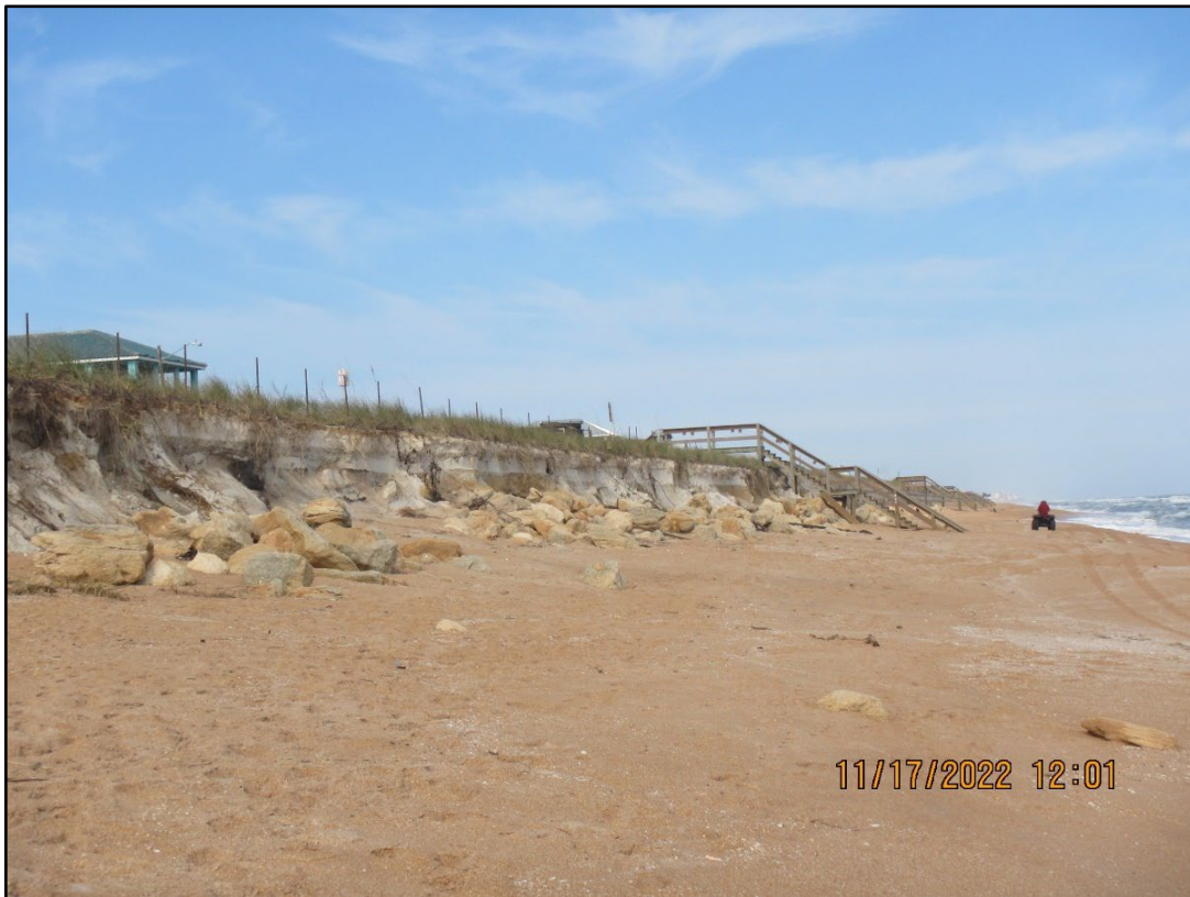
Figure 76. Flagler Beach after Hurricane Nicole (R-69).
