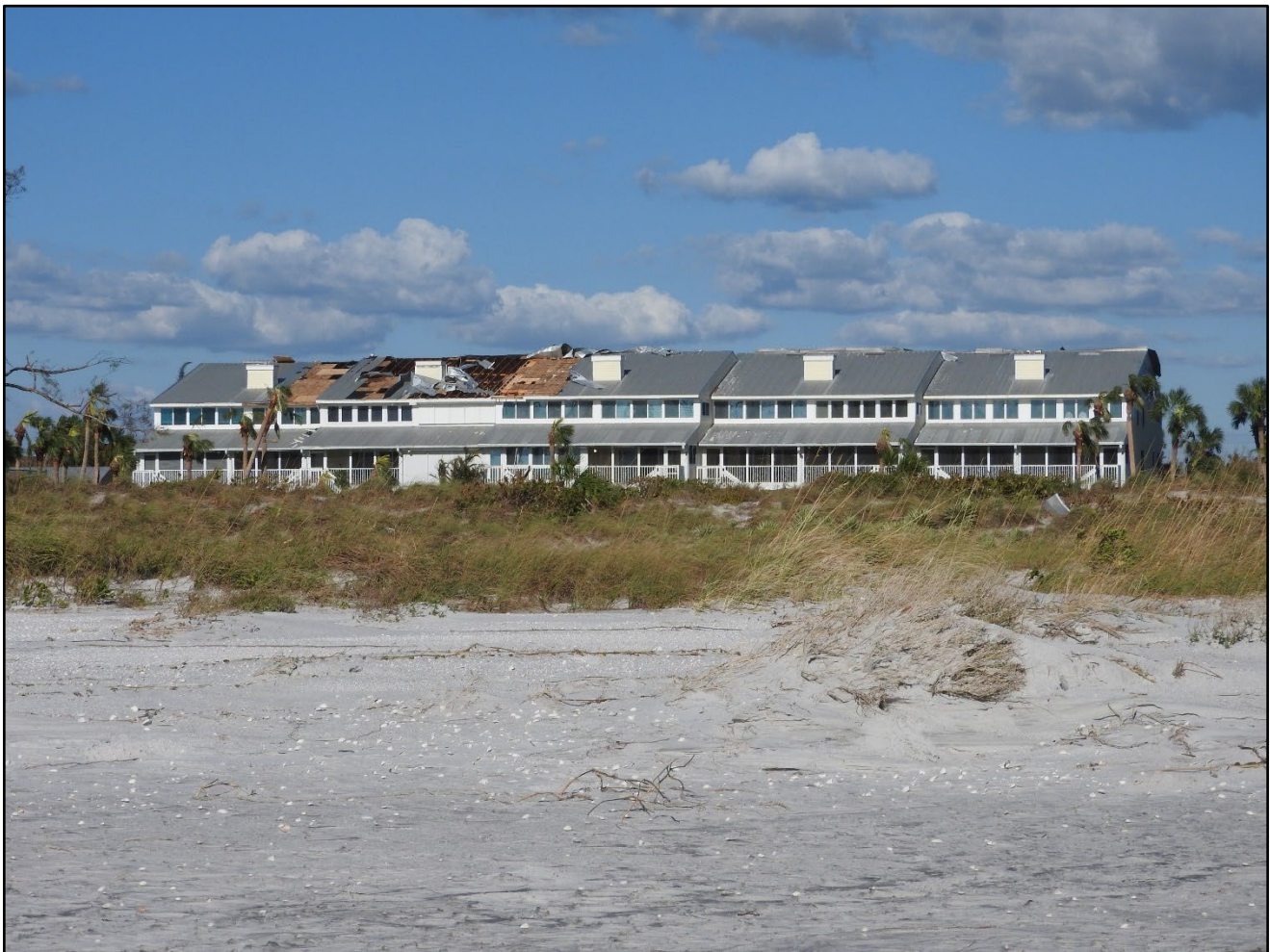
Figure 25. Major roofing damage on condominiums on northern Gasparilla Island (R-64).
