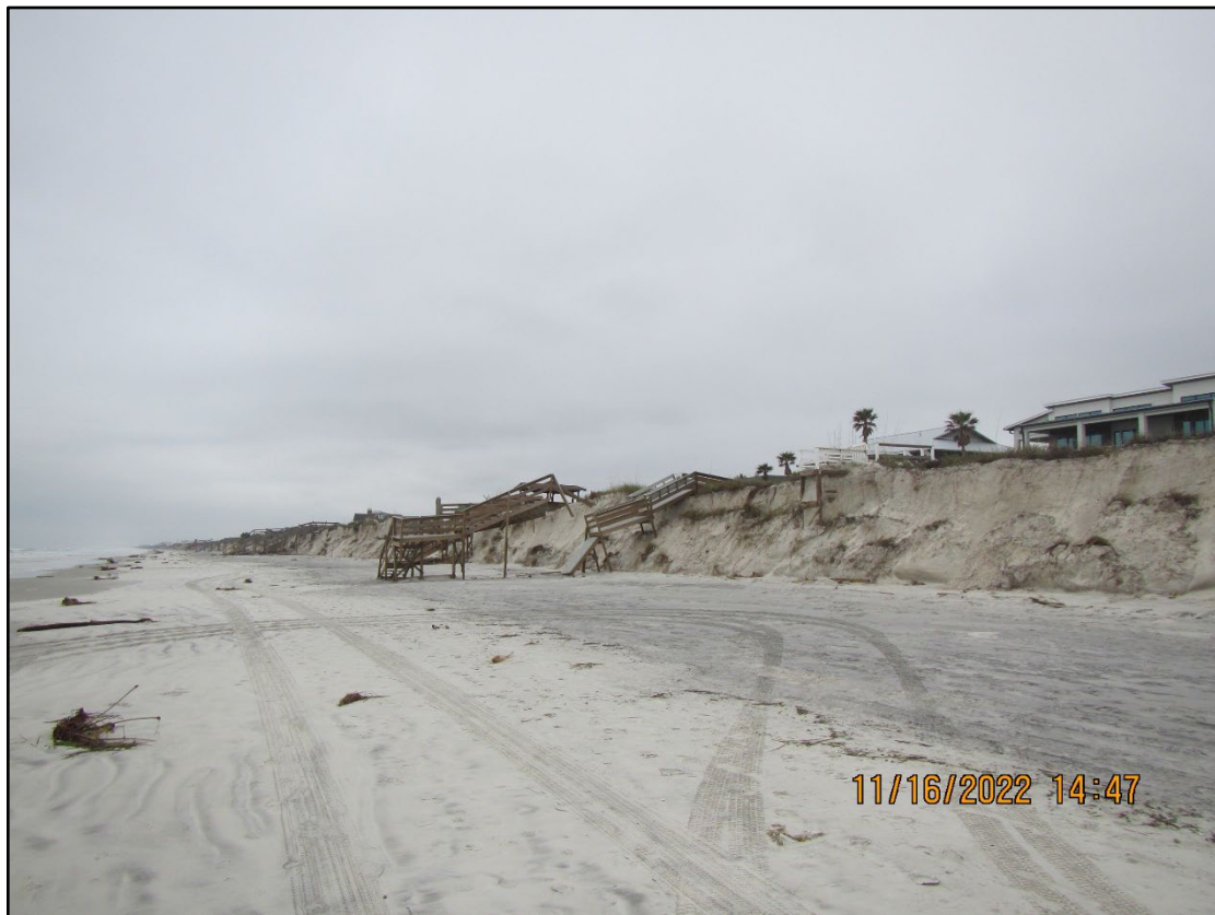
Figure 63. Major beach and dune erosion at Crescent Beach (R-172).
