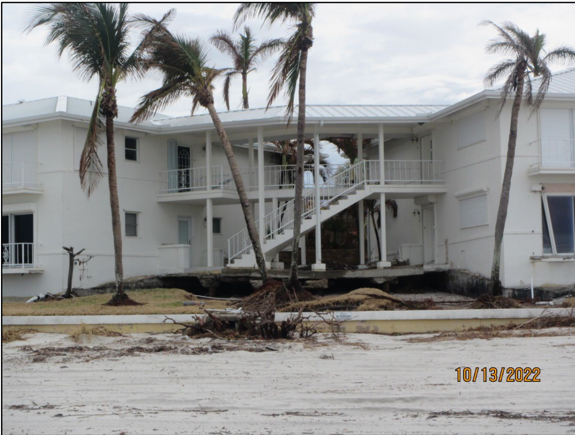
Figure 50. Understructure damage in Naples (R-60).
