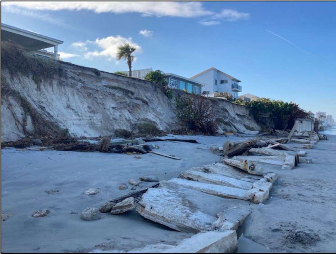
Figure 94. Catastrophic seawall collapse with loss of upland property in Wilbur by the Sea (R125).
