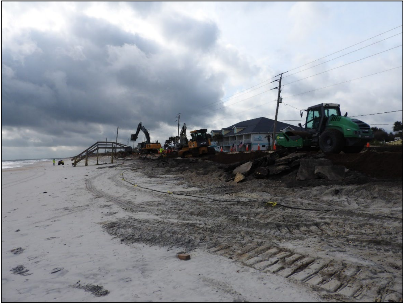
Figure 60. Major beach and dune erosion and road damage at Vilano Beach (R-115).
