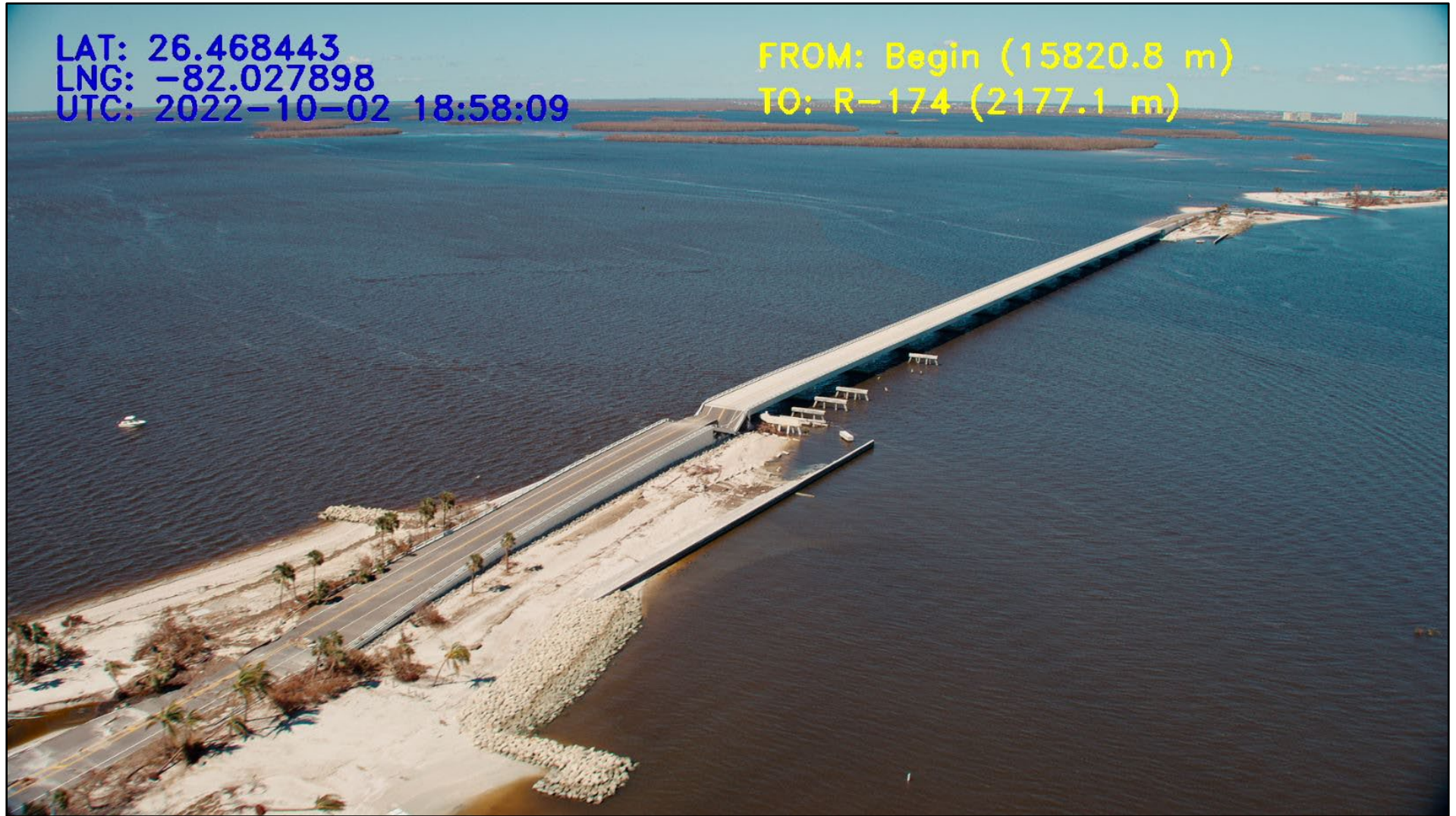
Figure 35. Sanibel Island bridge and causeway destroyed. (Image source: Active Camera Systems and Camera Copters).
