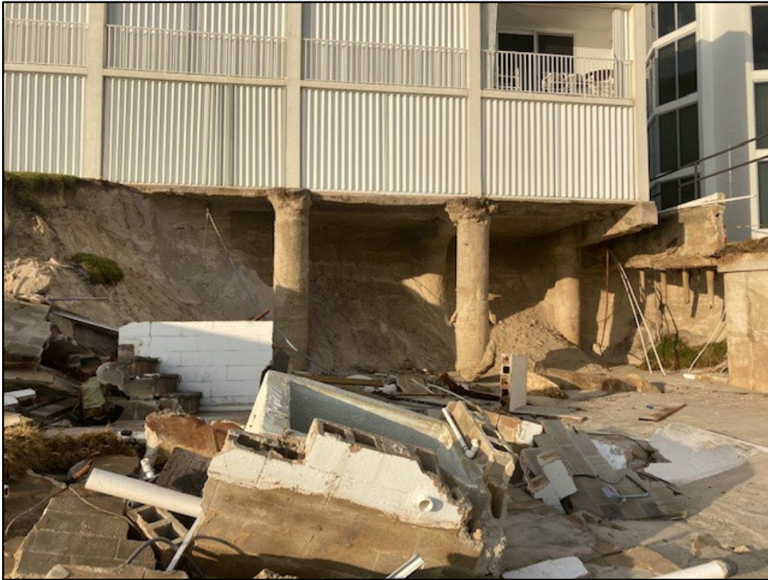
Figure 105. Threatened multifamily dwelling with foundation piles suspended (R117).
