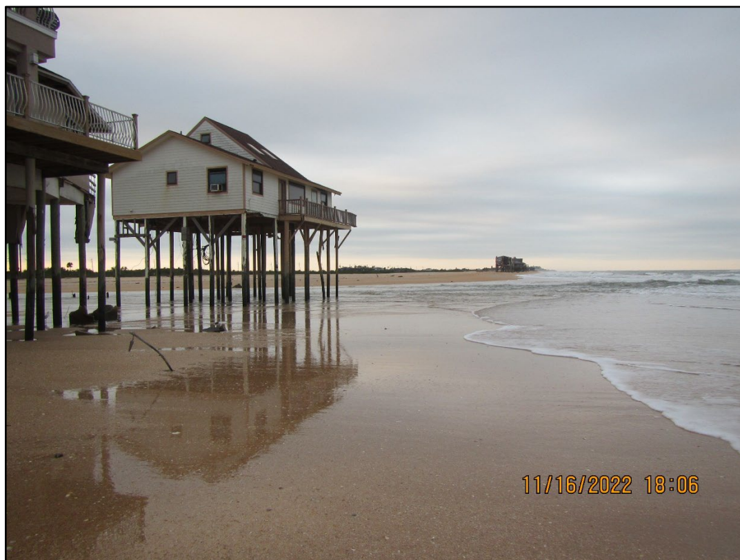
Figure 66. Coastal barrier breach at Summer Haven (R204.9).
