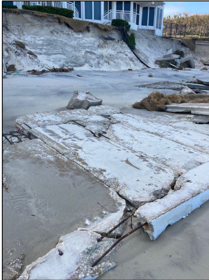
Figure 88. Old seawall with corroded reinforcing steel in Daytona Beach Shores (R116).
