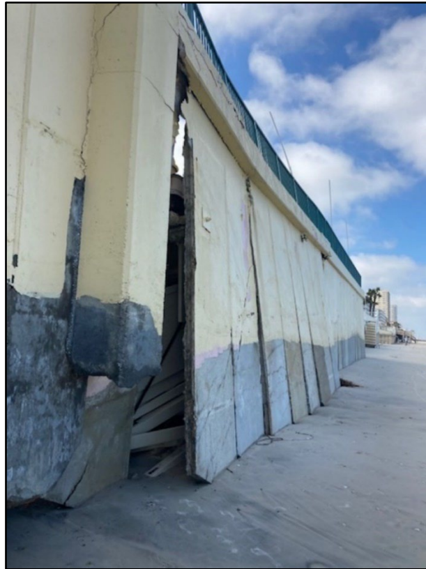
Figure 90. Inadequate sheet pile penetration.
