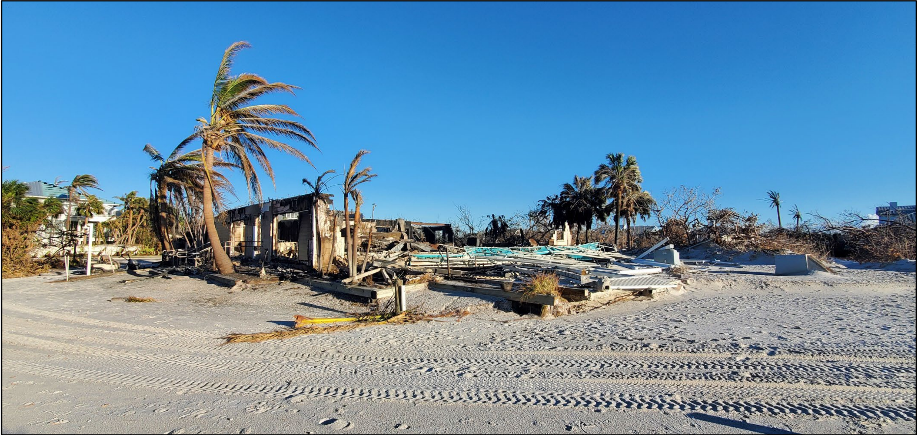
Figure 32. South Beach Bar and Grill Restaurant on Gasparilla Island near R-25 that caught fire during Hurricane Ian.
