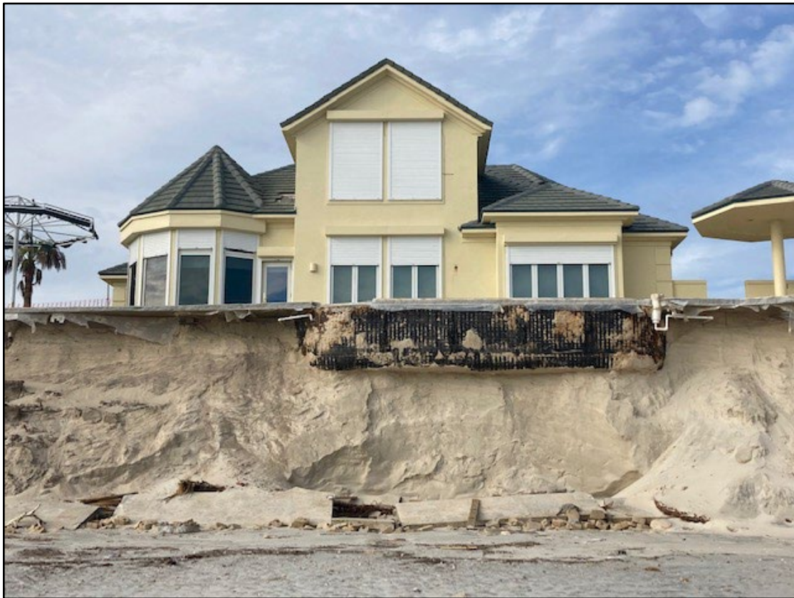
Figure 107. House and pool in imminent danger, Wilbur-by-the-Sea (R122).
