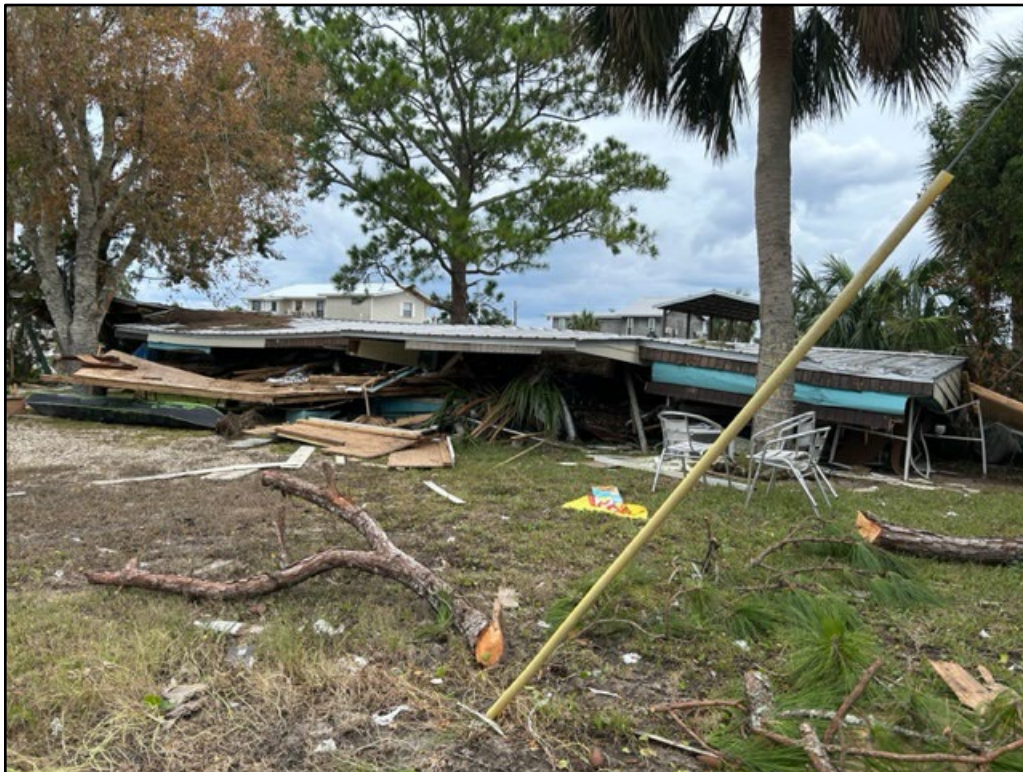
Figure 30. Dwelling destroyed in Horseshoe Beach.
