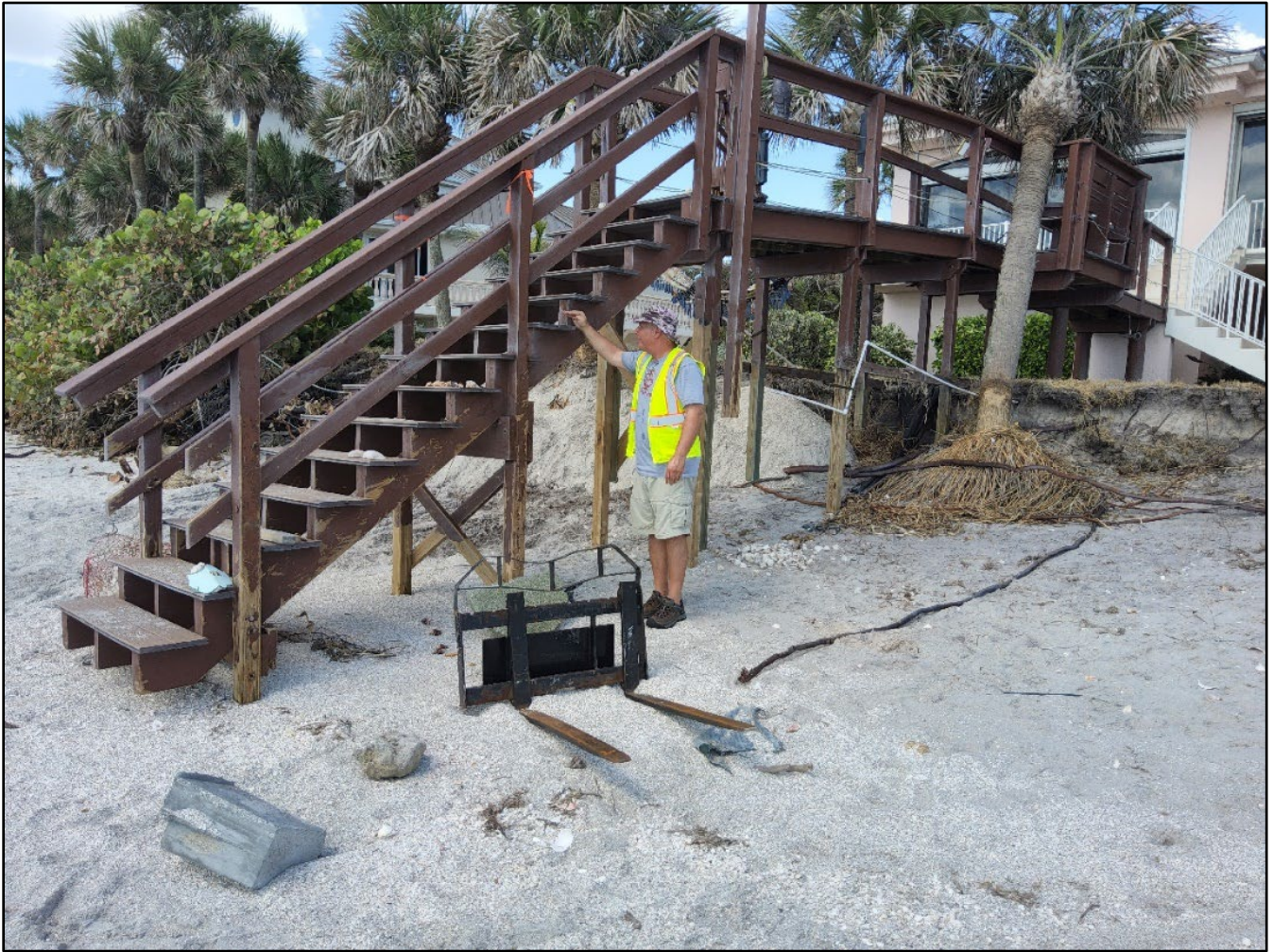
Figure 58. Erosional losses demonstrated by the mark on the stairs of the dune walkover at Manasota Key, near R174, just north of Blind Pass Park.
