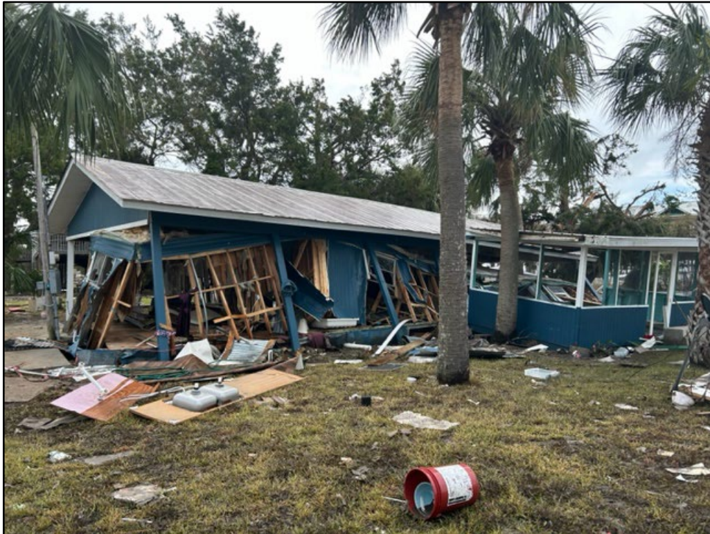
Figure 36. On-grade dwelling destroyed, Horseshoe Beach.
