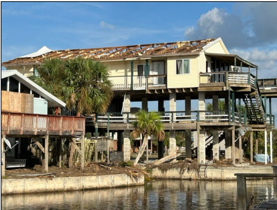
Figure 14. Major roof damage in Dekle Beach.
