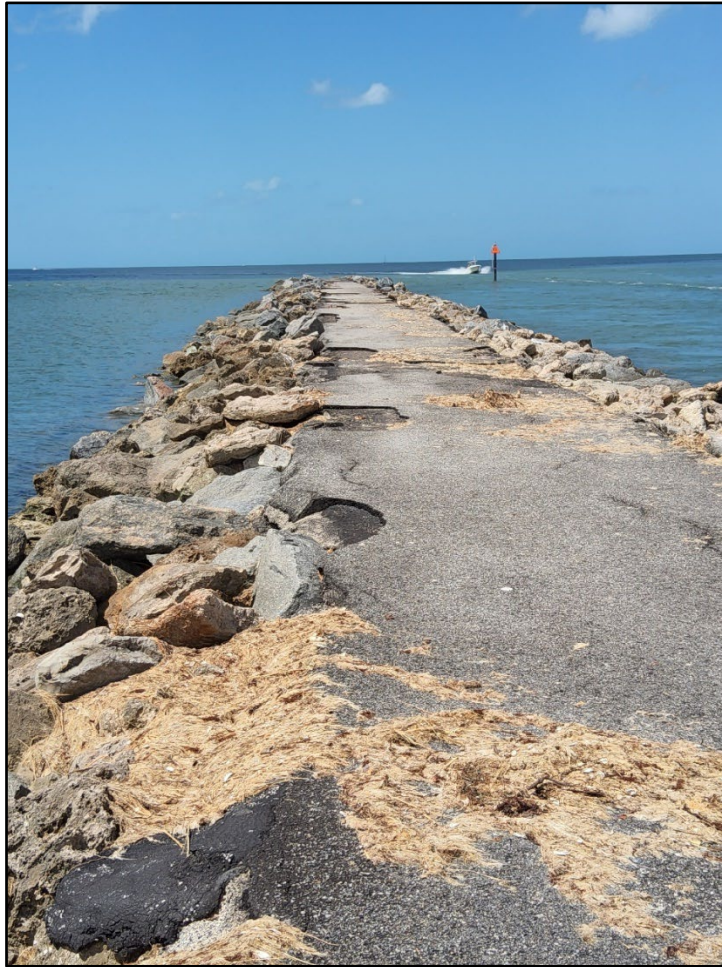
Figure 63. Damage to the south jetty at Venice Inlet, R115.
