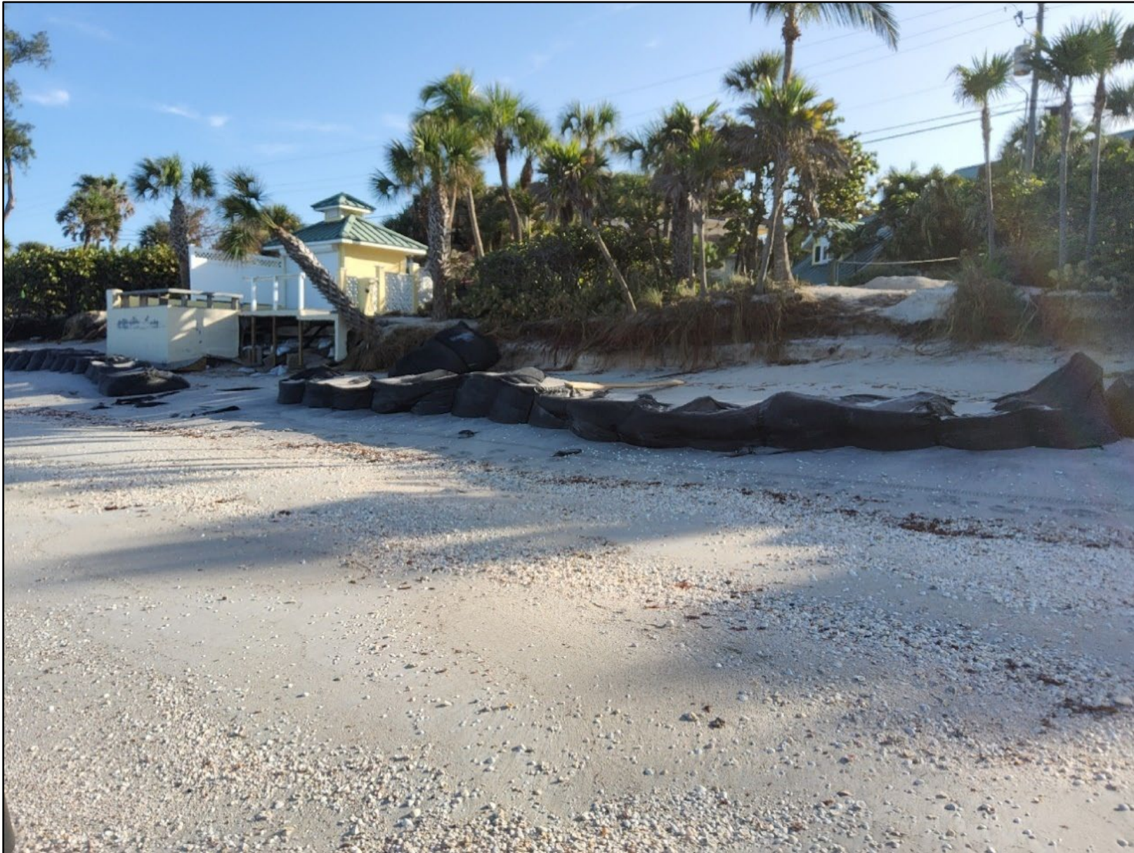
Figure 62. Moderate beach and dune erosion (condition III) damaged geotextile sandbags on Casey Key near R100.
