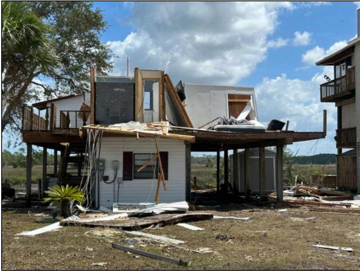
Figure 15. House destroyed by wind in Keaton Beach.
