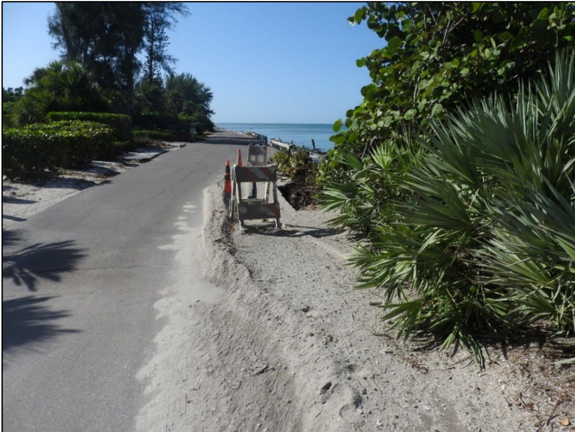
Figure 61. Damage to road on Casey Key, near R84.5.
