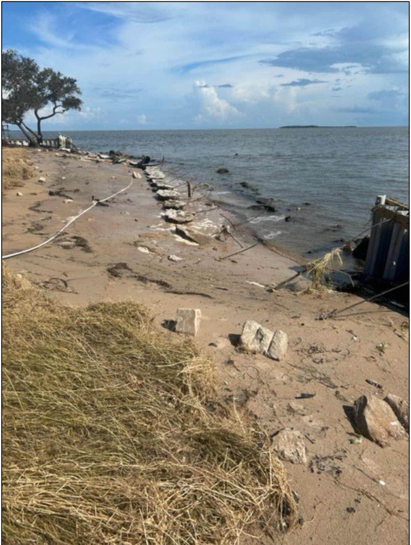
Figure 44. Composite seawall destroyed at Piney Point, Cedar Key.
