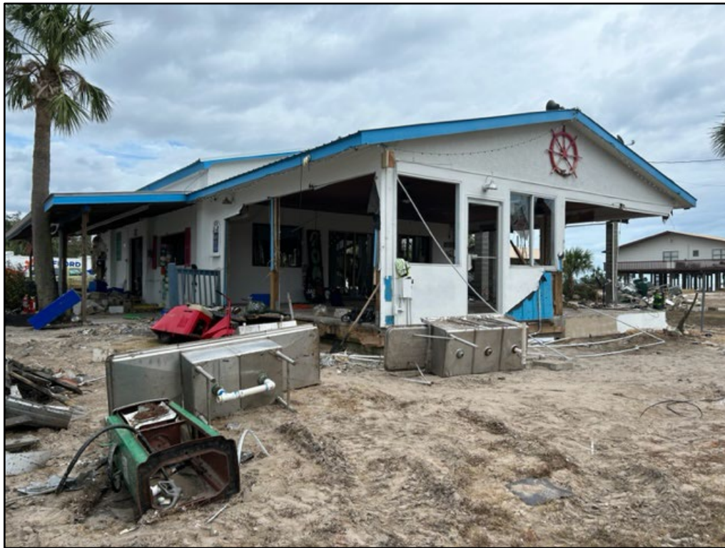
Figure 28. Major damage to the marina building, Horseshoe Beach.
