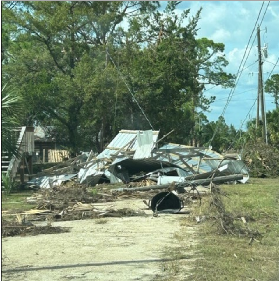
Figure 16. Wind damaged structure on Cedar Island.
