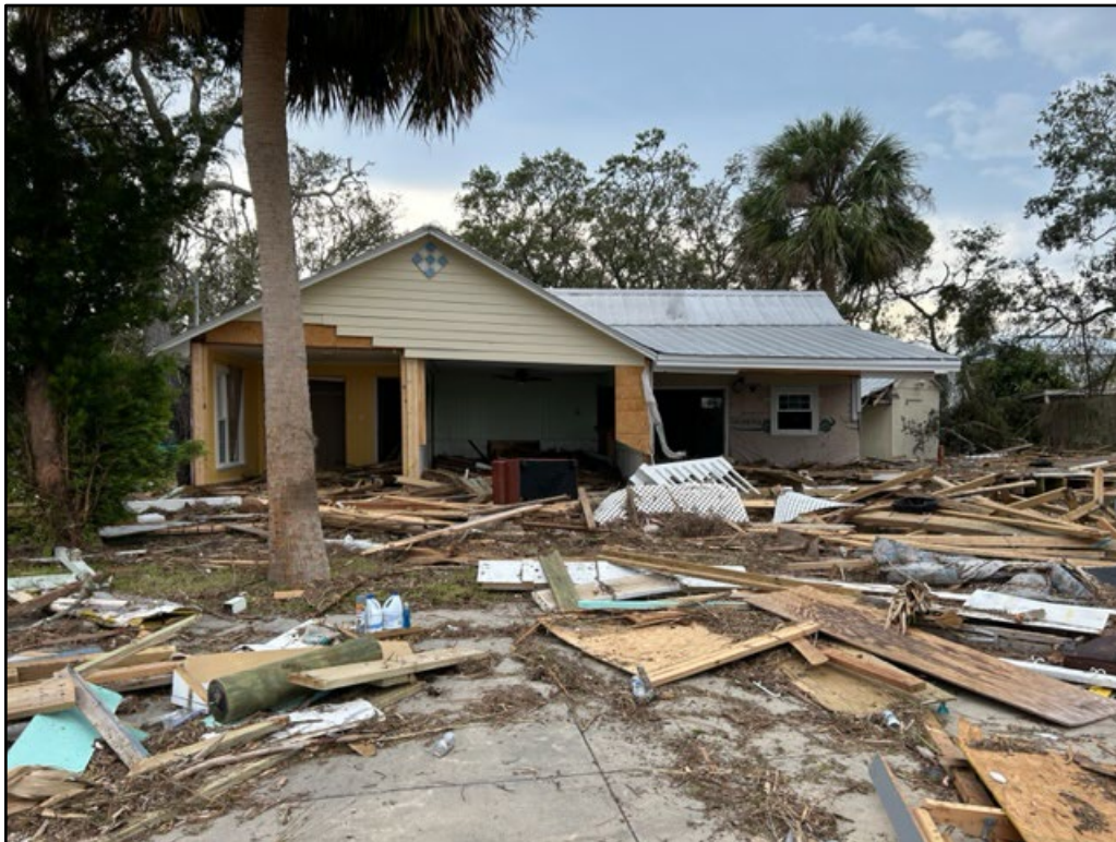
Figure 32. Dwelling destroyed in Horseshoe Beach.
