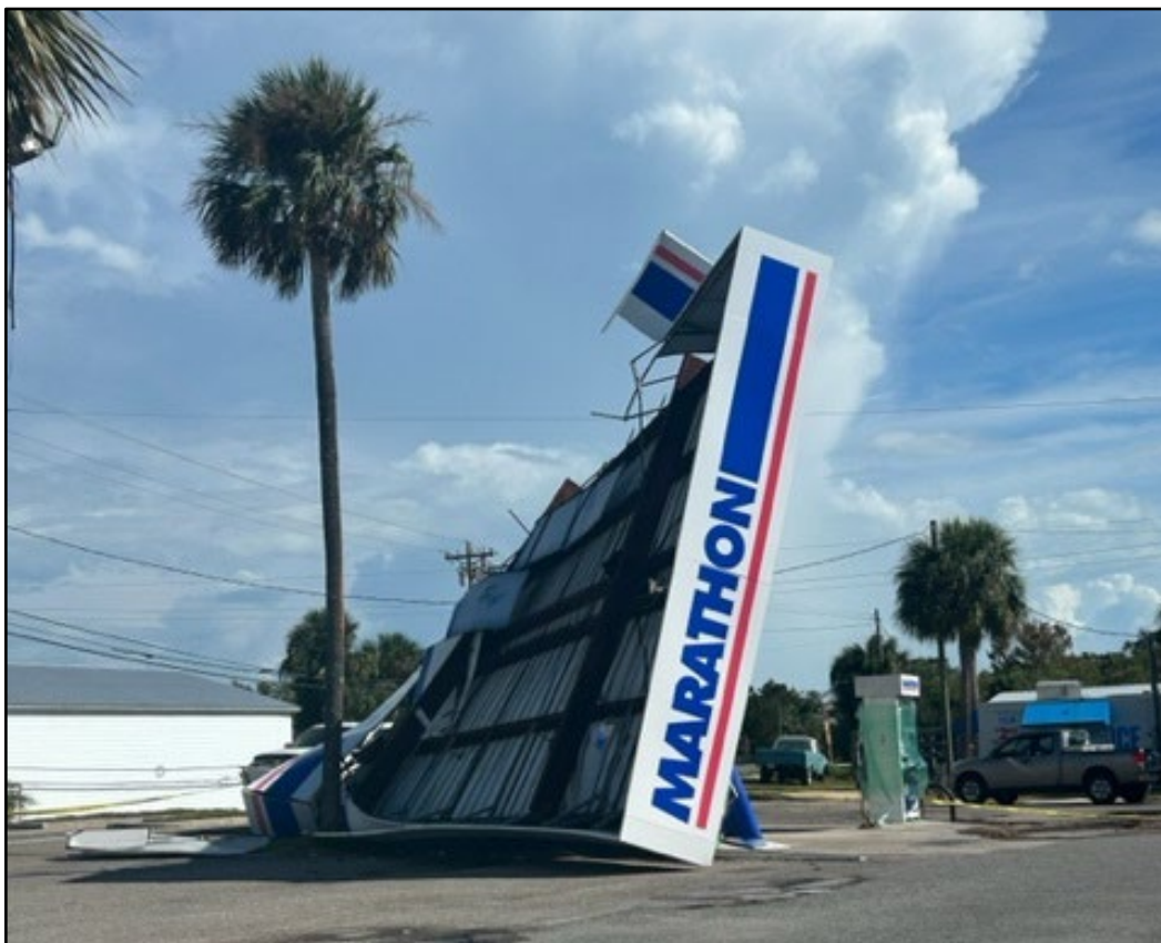
Figure 43. Wind damage in Cedar Key.
