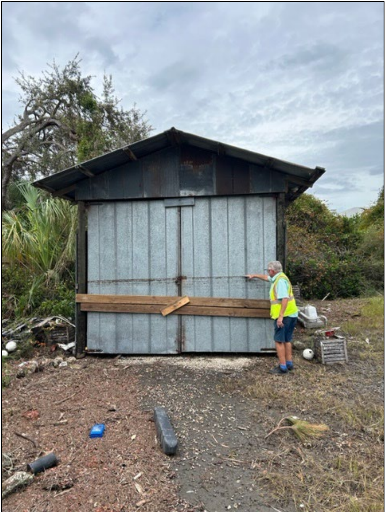
Figure 27. Mud line on interior Horseshoe Beach shed indicating storm surge elevation.
