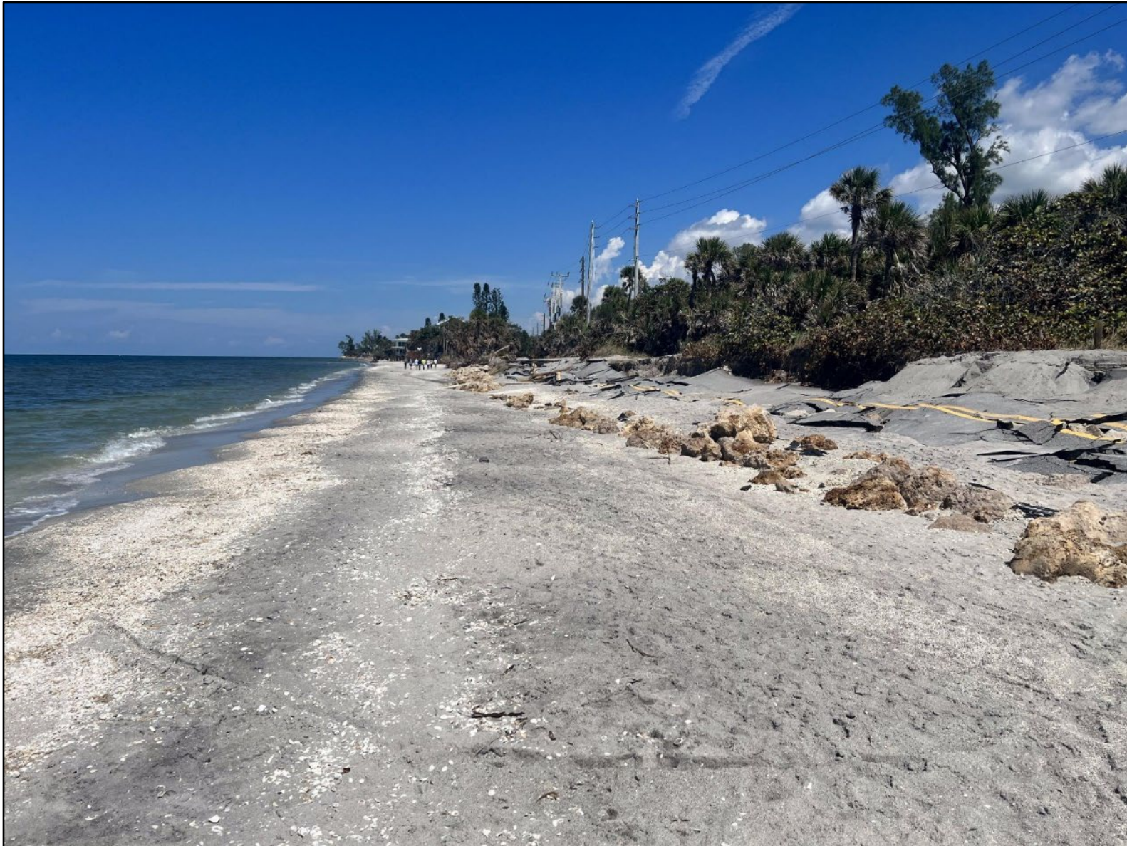
Figure 65. Major damage to Manasota Key Road at R175 north of Blind Pass Park (photo courtesy of Vadim Alymov with Coastal Engineering Consultants Inc.).
