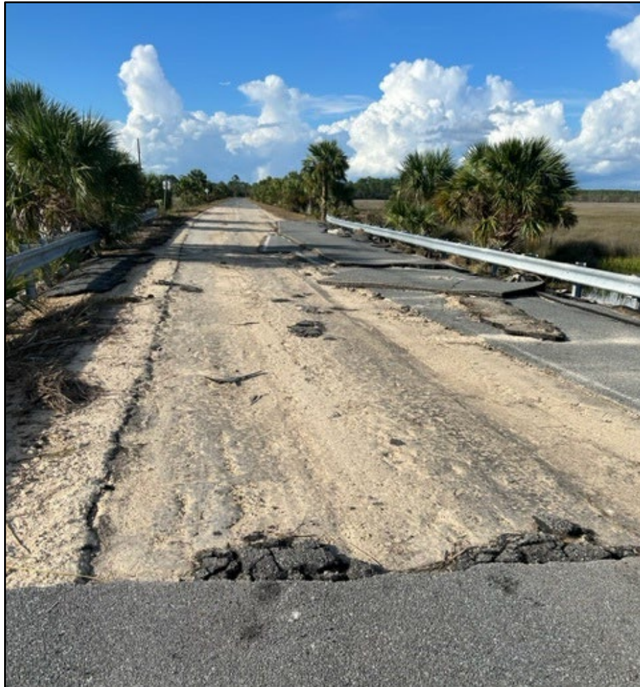
Figure 26. Road damage at Shired Island.
