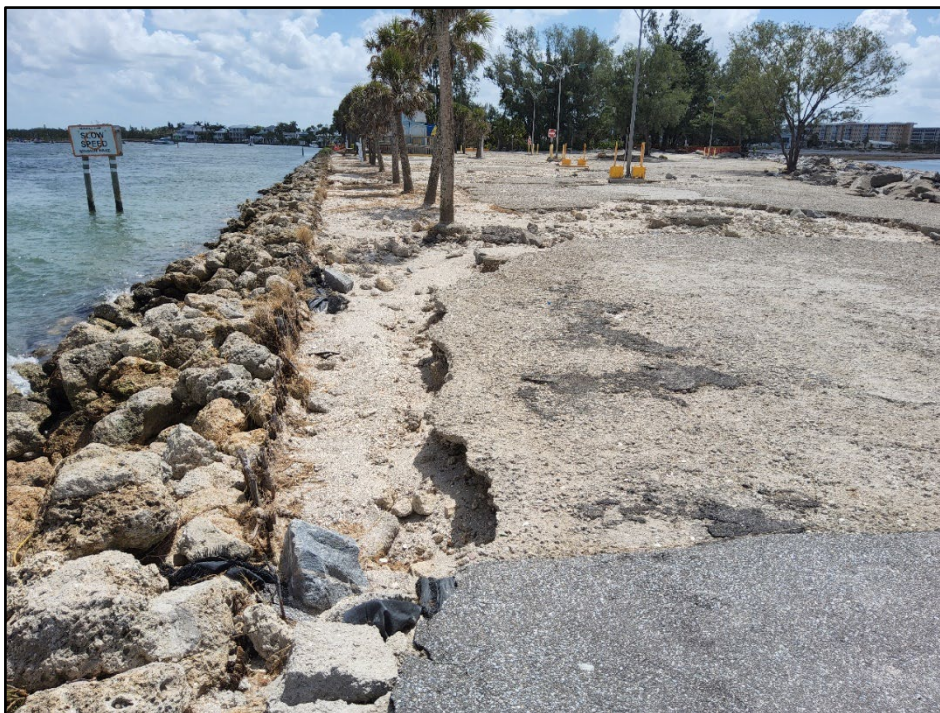
Figure 64. Damage to the south jetty at Venice Inlet, R115.
