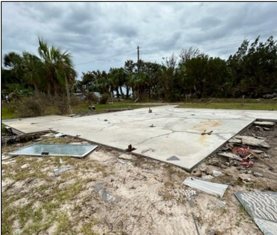
Figure 39. Pile supported dwelling destroyed, Horseshoe Beach.
