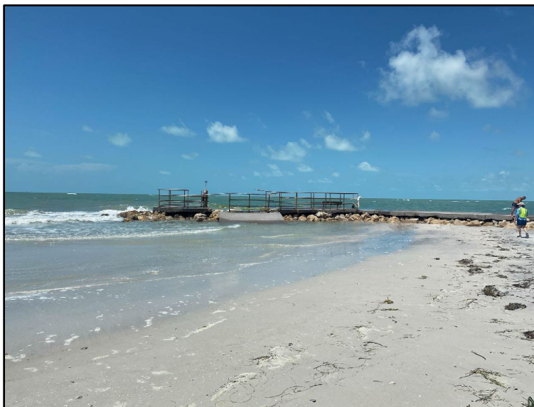
Figure 53. Major damage to the John's Pass south jetty near R126 (photo courtesy of Zach Westfall with Pinellas County).
