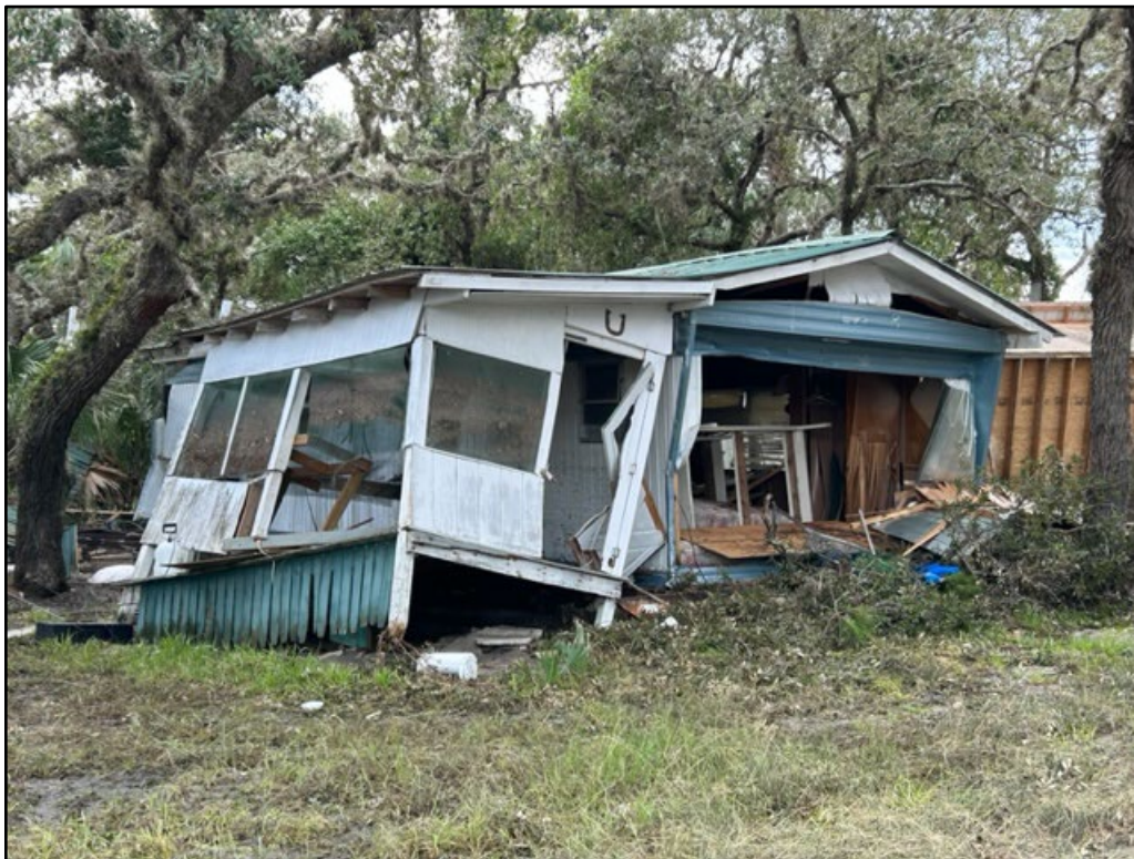
Figure 31. Dwelling destroyed in Horseshoe Beach.
