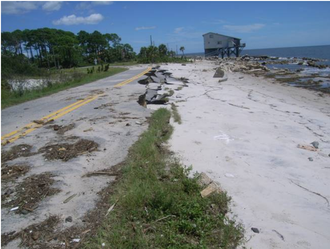
Figure 3. Damage to Chip Morrison Drive at the Southwest Cape, Alligator Point.
