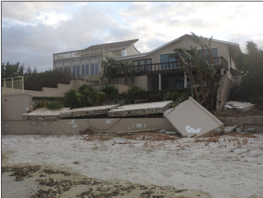
Figure 19b. Failure of a concrete seawall in Wilbur-By-The-Sea, Volusia County (R123.4).
