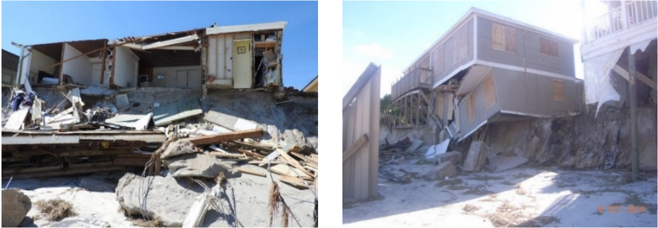
Figure 8. Examples of structural damages to major structures in St. Johns County.
