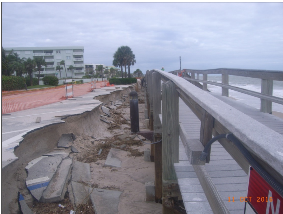
Figure 21a. Major beach and dune erosion undermining parking area along Ocean Drive at Conn Park in Vero Beach, Indian River County (R79).
