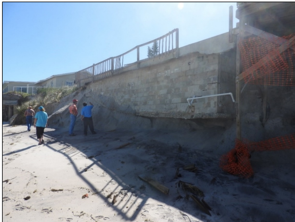
Figure 20b. Major beach and dune erosion undermining a swimming pool in south Brevard County (R158.7).
