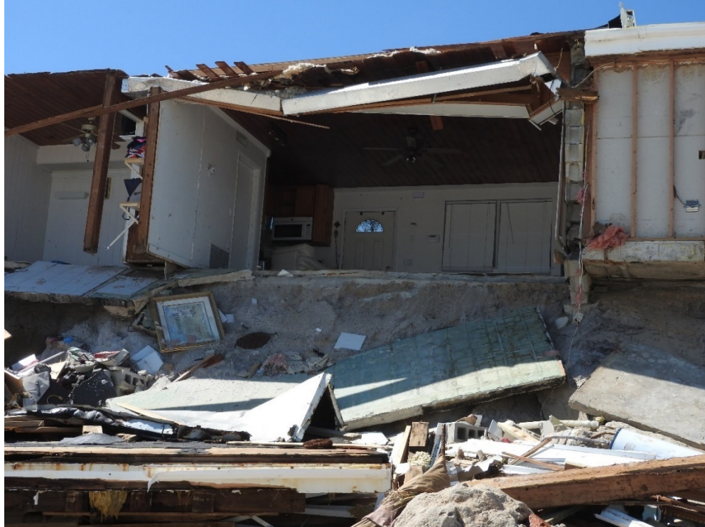
Figure 17a. Timber seawall and single-family dwelling destroyed in South Ponte Vedra, St. Johns County (R088+250').
