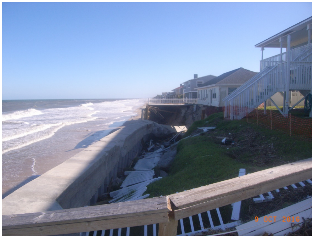
Figure 17b. Composite seawall with concrete cap destroyed in South Ponte Vedra, St. Johns County (R089+300').
