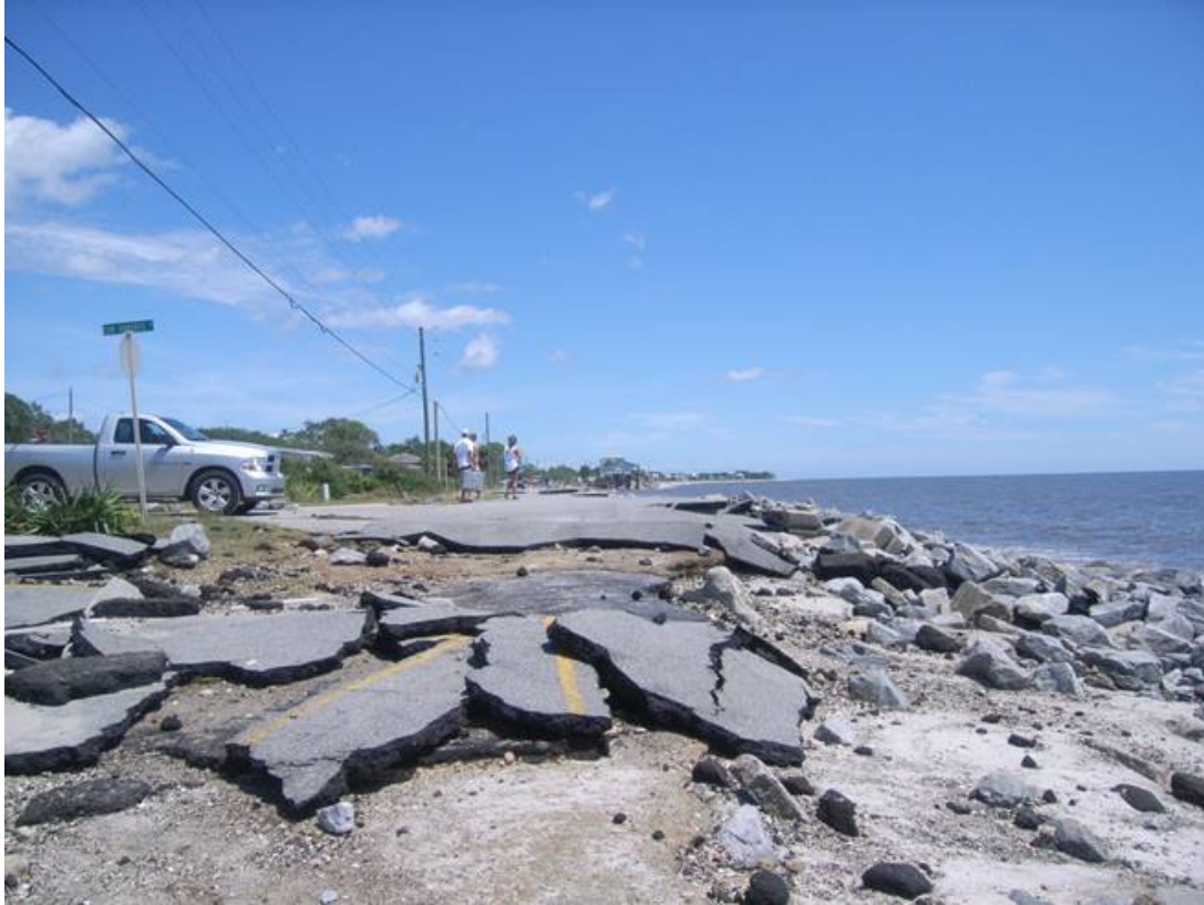
Figure 4. Alligator Point Road and revetment damage, Alligator Point.
