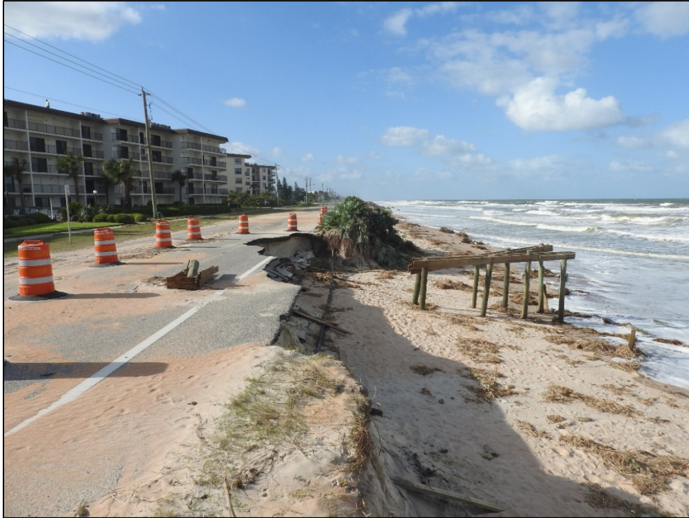
Figure 19a. Major beach and dune erosion and damage to State Road A1A in northern Volusia County (R29.5).
