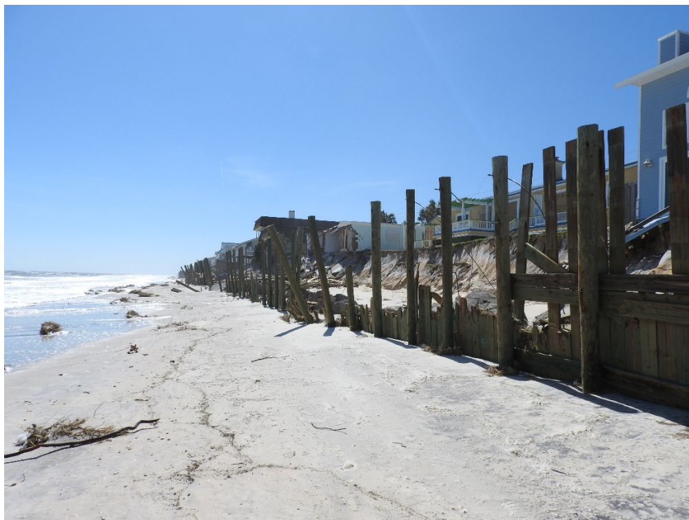
Figure 17d. Major dune erosion and major structural damage to single-family dwellings in South Ponte Vedra, St. Johns County (R87).
