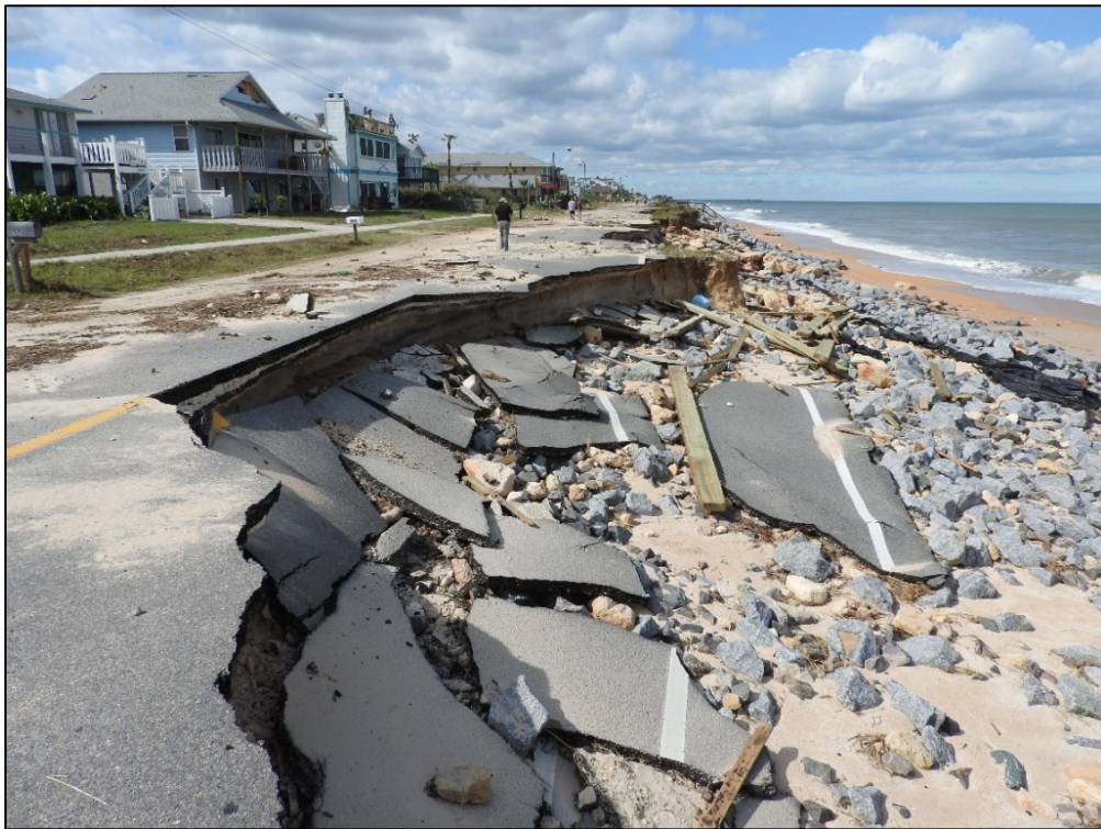
Figure 18b. Rock revetment and State Road A1A destroyed in Flagler Beach (R84.5).
