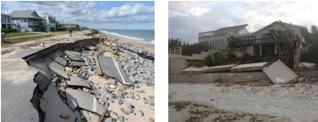
Figure 9. Examples of damages to paved roads and coastal armoring.
