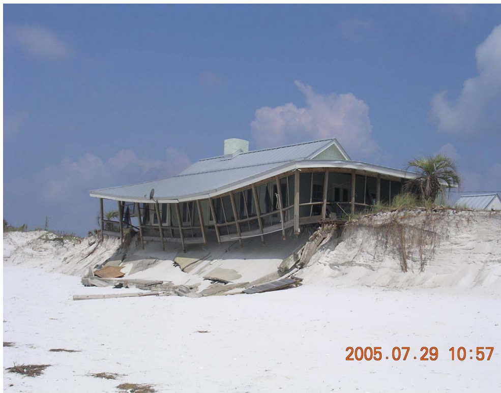
Photo 2. Dwelling undermined and damaged (R176.2)
