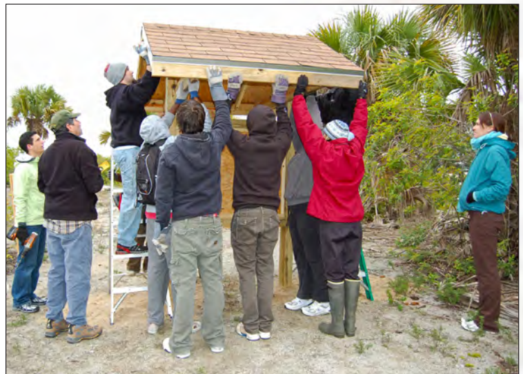
Outreach displays, like this kiosk being built by volunteers, help educate visitors about the importance of the IRLAP System.
