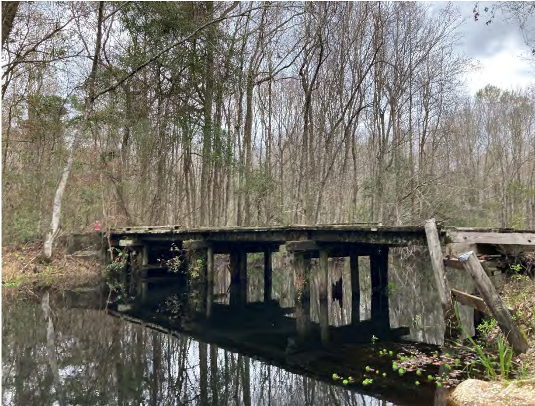
10. One of seven bridges recorded within the project along the historic Seven Bridges Road.
