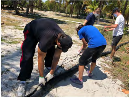
University of Miami students and technicians placing WERA HFR cables inside of 4" corrugated pipe. The conduit with the HFR cables inside was placed within the vegetation at the HFR site at Crandon Park, Miami, FL.
