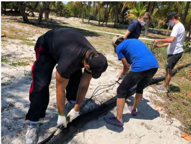
University of Miami students and technicians placing WERA HFR cables inside of 4" corrugated pipe. The conduit with the HFR cables inside was placed within the vegetation at the HFR site at Crandon Park, Miami, FL.
