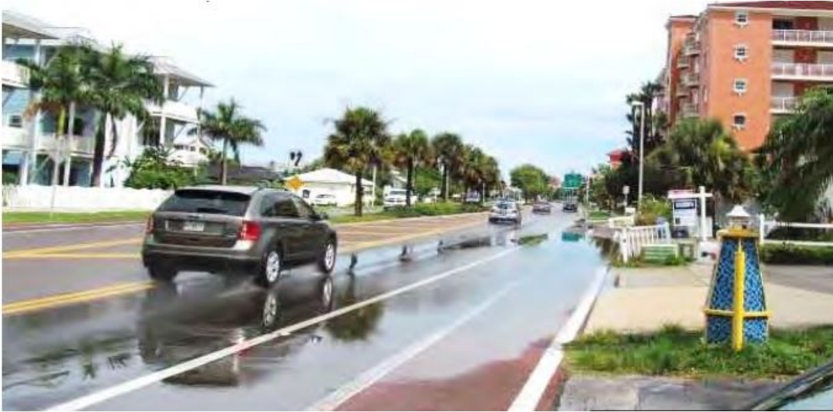
Figure 7-3. Failure of permeable pavement. (Photo: Tim Kelly, Wood Environment & Infrastructure Solutions)
