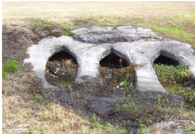
Figure 7-2. Sedimentation in inlet pipes. (Photo: Tim Kelly Wood Environment & Infrastructure Solutions, Inc.)
