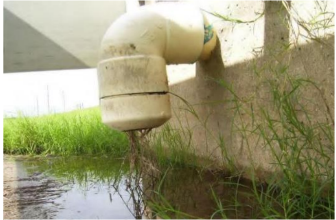
Figure 7-1. Clogged drawdown orifice. (Photo: Tim Kelly Wood Environment & Infrastructure Solutions, Inc.)
