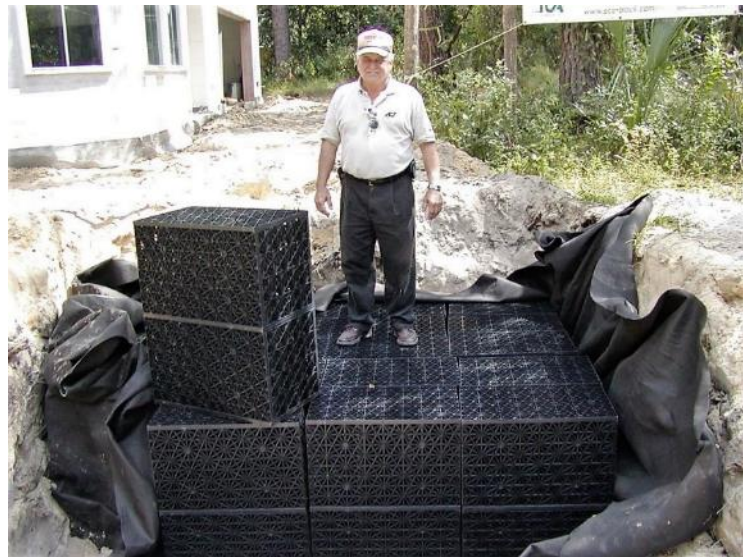
Figure 5-8. Installation of underground exfiltration media, Madera subdivision, Alachua County, Florida. [Photo, UF-PREC]
