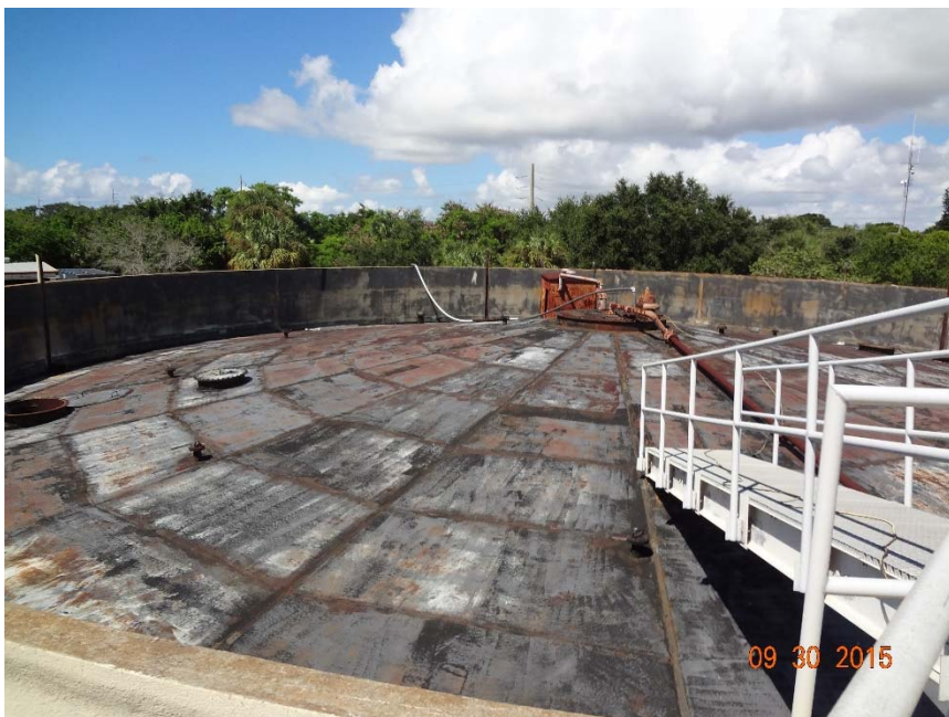
Figure SWWRF-4. Anaerobic Digester No. 2 Floating Cover Southwest WRF
