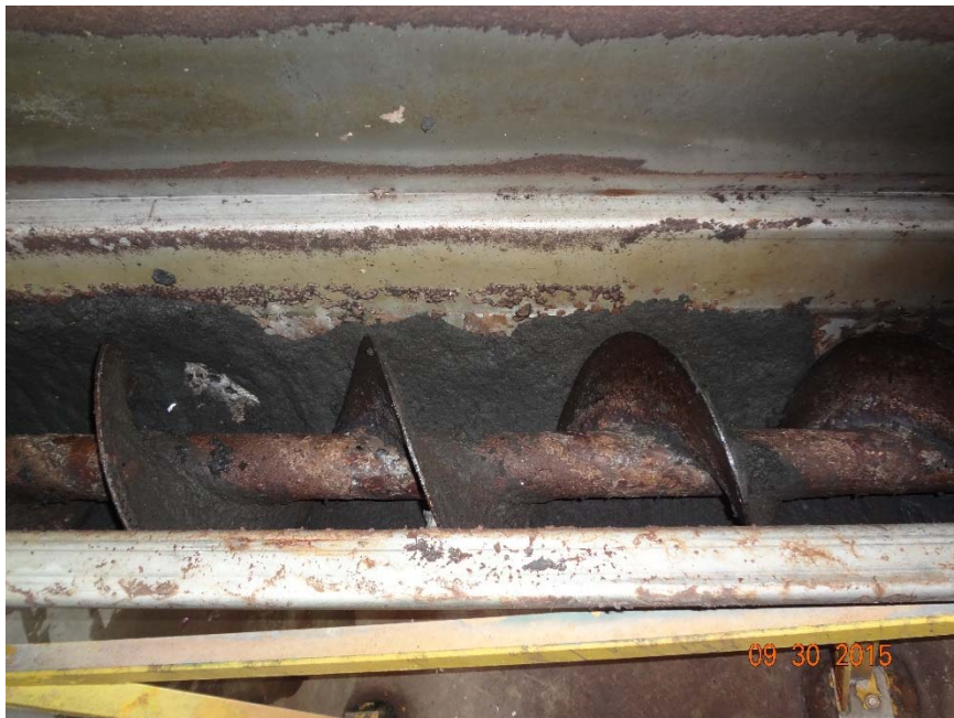
Figure NWWRF-16. Dewatered Sludge Conveyor Northwest WRF
