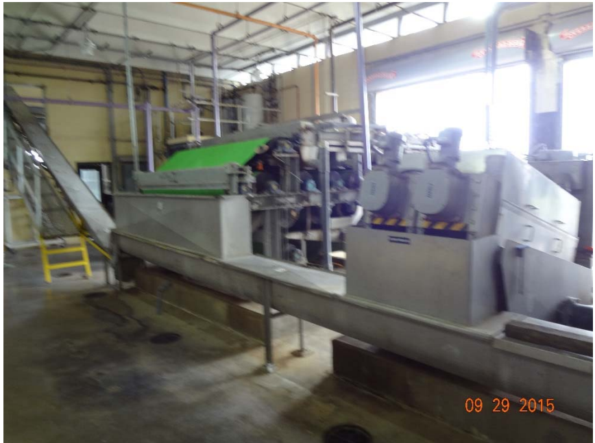
Figure NEWRF-8. Dewatering Building Northeast WRF
