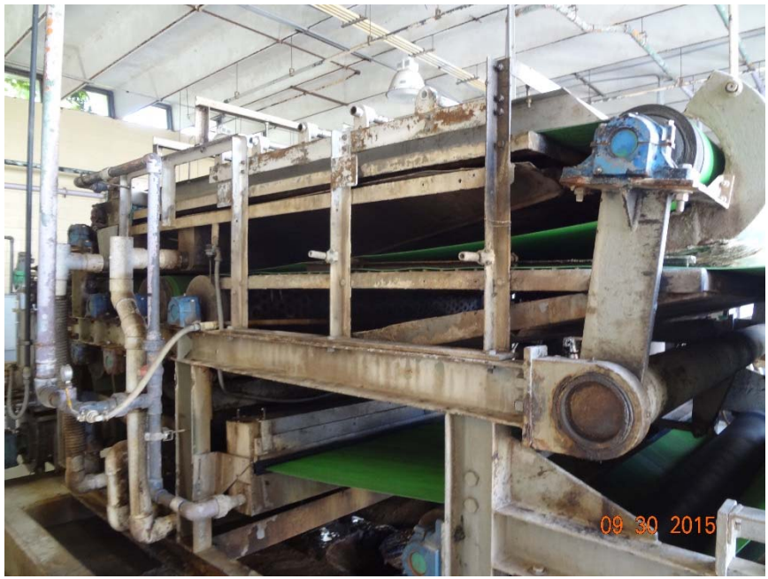
Figure NWWRF-11. Belt Filter Press Northwest WRF
