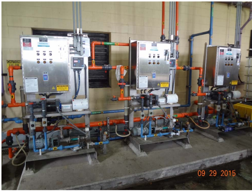
Figure NEWRF-9. Dewatering Polymer Blending Units Northeast WRF
