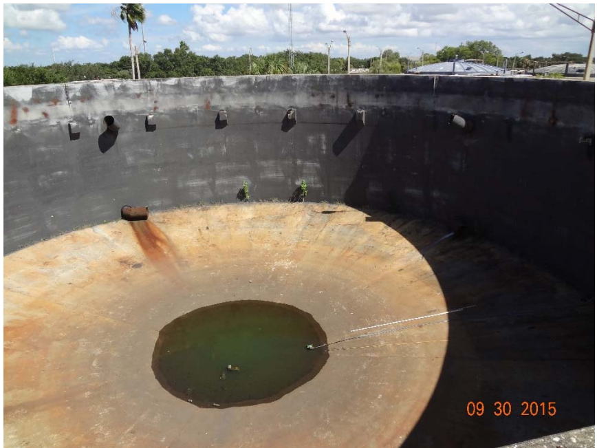
Figure NWWRF-6. Anaerobic Digester No. 4 Northwest WRF
