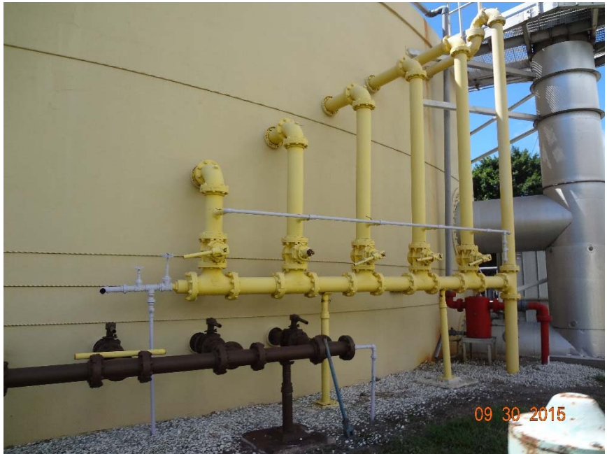
Figure SWWRF-6. Anaerobic Digester Decant No. 3 Piping and Draft Tube Mixer Southwest WRF
