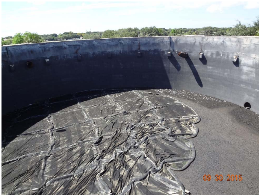
Figure NWWRF-5. Anaerobic Digester No. 3 Northwest WRF
