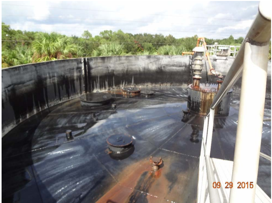
Figure NEWRF-6. Anaerobic Digester No. 2 Floating Cover Northeast WRF
