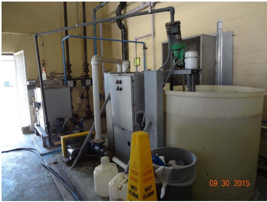
Figure NWWRF-15. Dewatering Polymer Storage and Feed Northwest WRF
