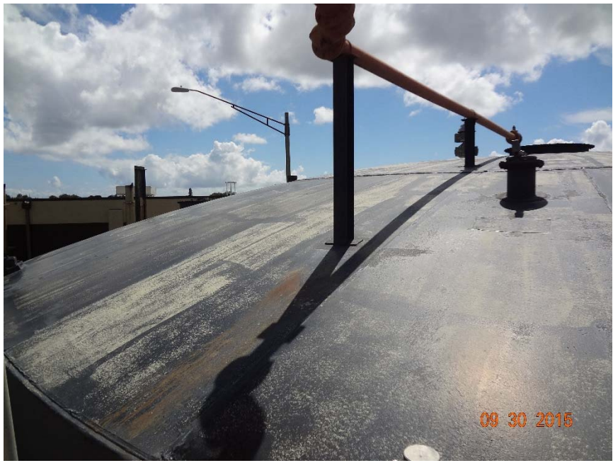
Figure NWWRF-3. Anaerobic Digester No. 1 Northwest WRF
