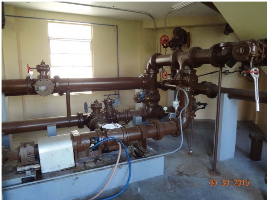
Figure NWWRF-4. Anaerobic Digester No. 1 and No. 2 Pumping Northwest WRF
