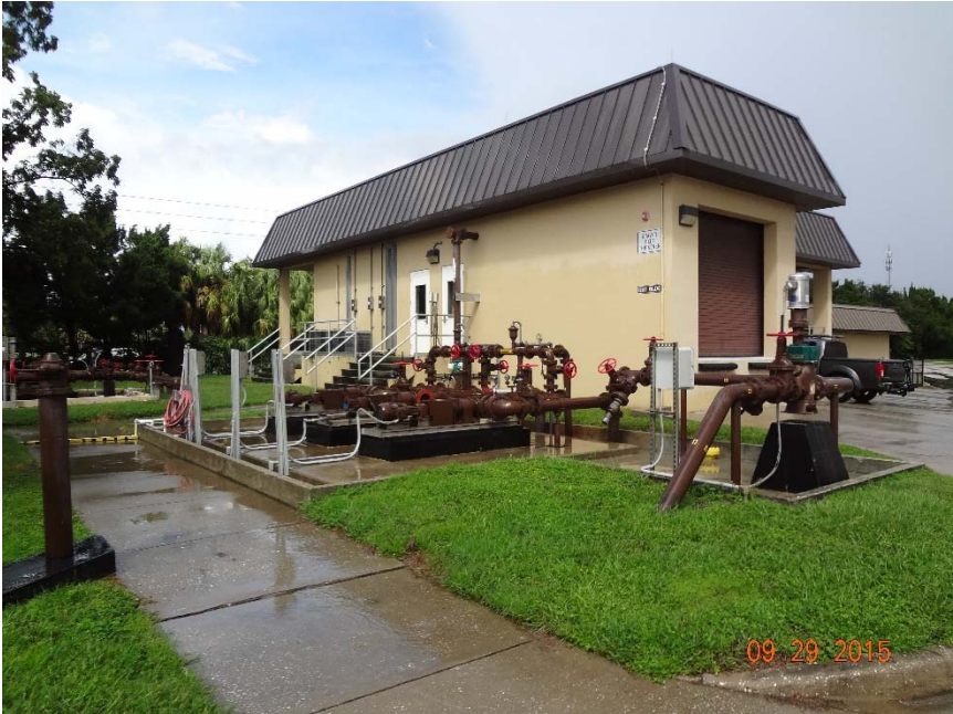
Figure NEWRF-2. Sludge Transfer Pump Station Northeast WRF
