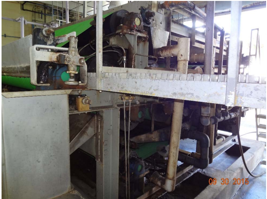
Figure NWWRF-12. Belt Filter Press Northwest WRF
