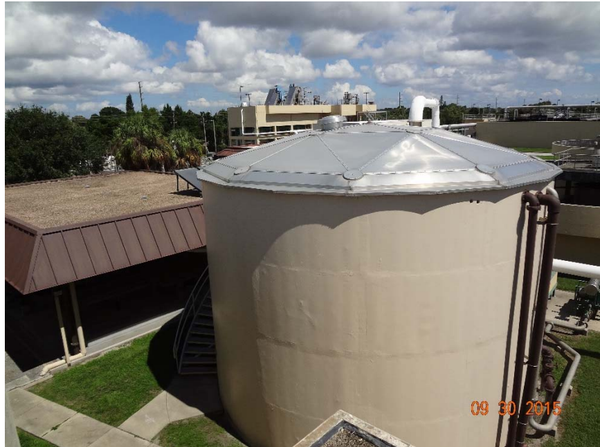
Figure SWWRF-1. Sludge Storage Tank Southwest WRF
