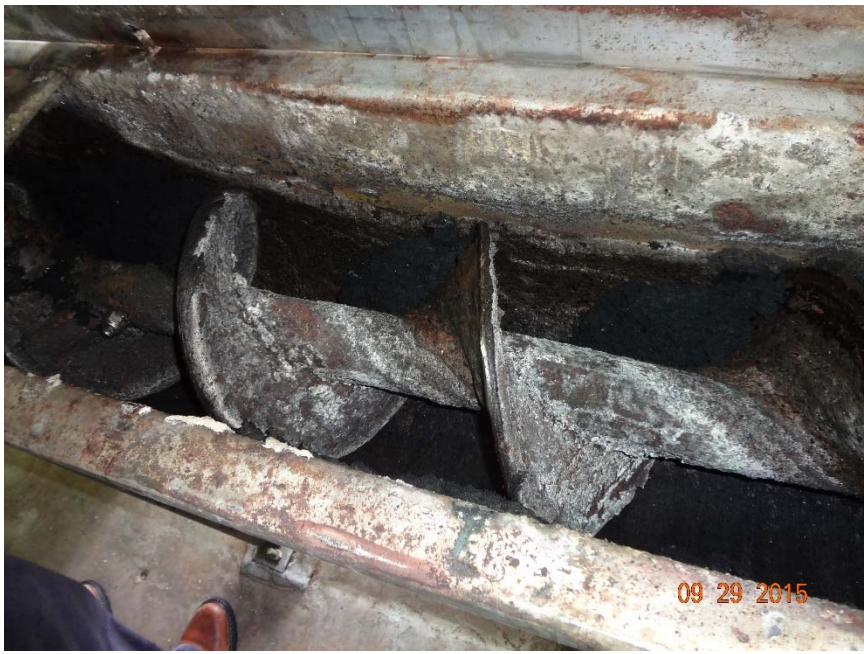
Figure NEWRF-11. Screw Conveyor Northeast WRF
