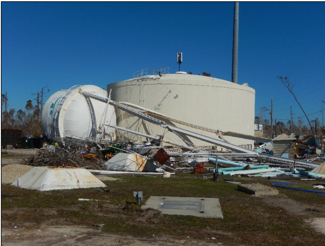
Figure 37. City water tower collapsed under high winds near R134, Mexico Beach.
