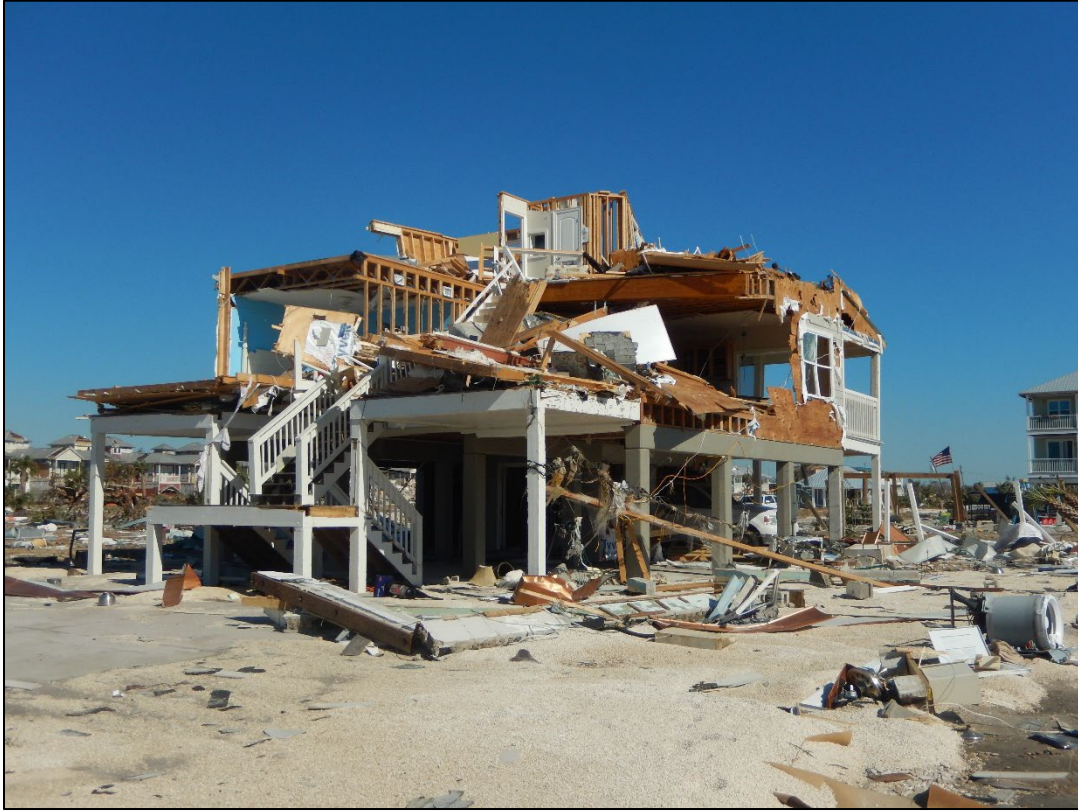
Figure 32. Pile-supported dwelling destroyed near R129, Mexico Beach.
