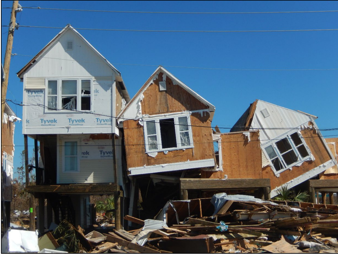
Figure 28. Beach dwellings north of U.S. 98 lifted off their foundations, R128, Mexico Beach.
