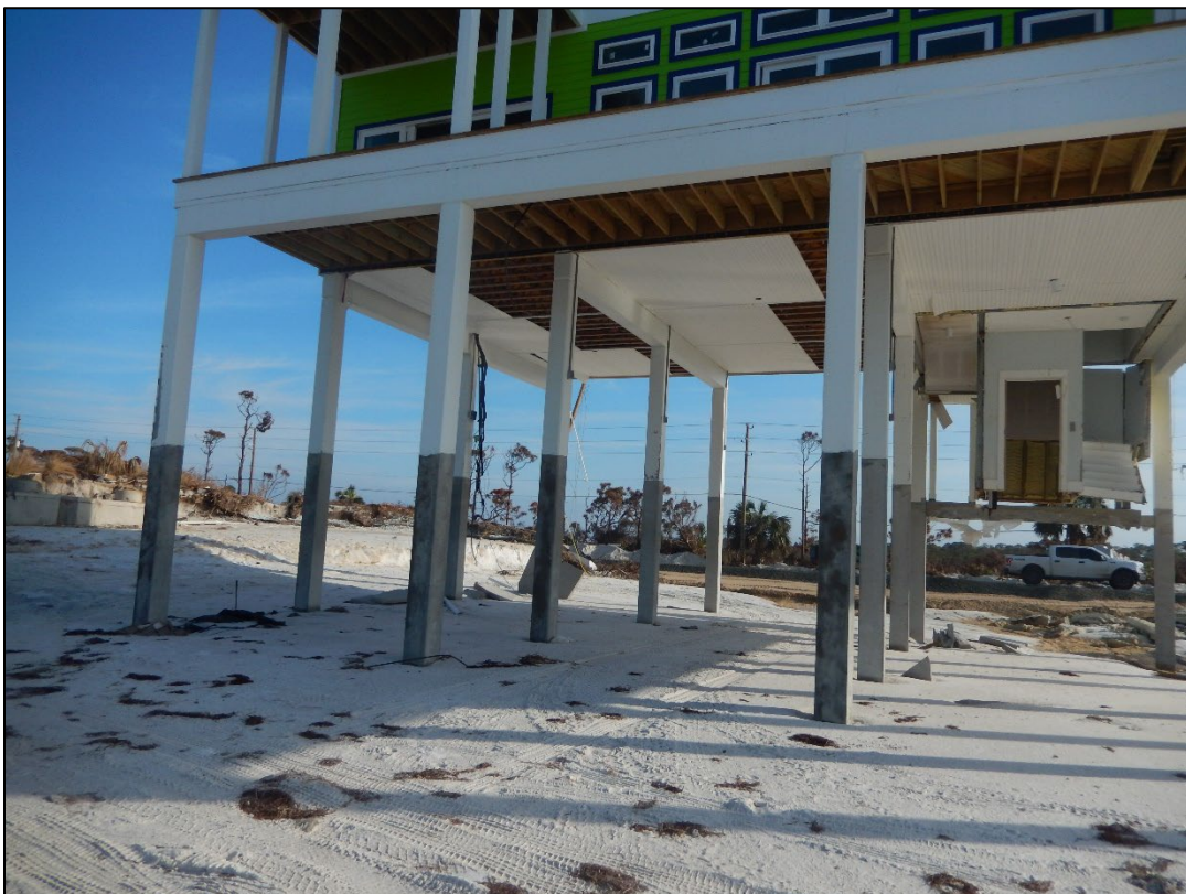
Figure 72. Over six feet of vertical loss of grade beneath structure near R104.
