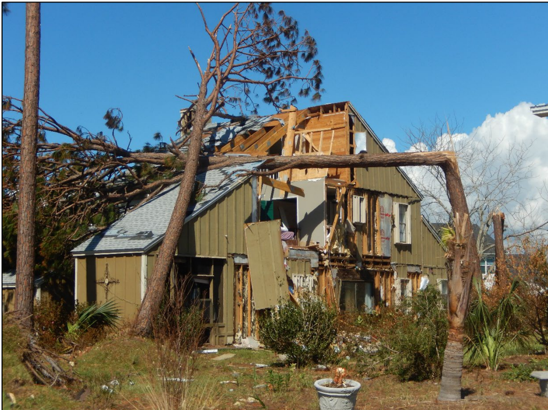
Figure 62. Major damage to dwelling due to high winds and fallen trees, Beacon Hill.
