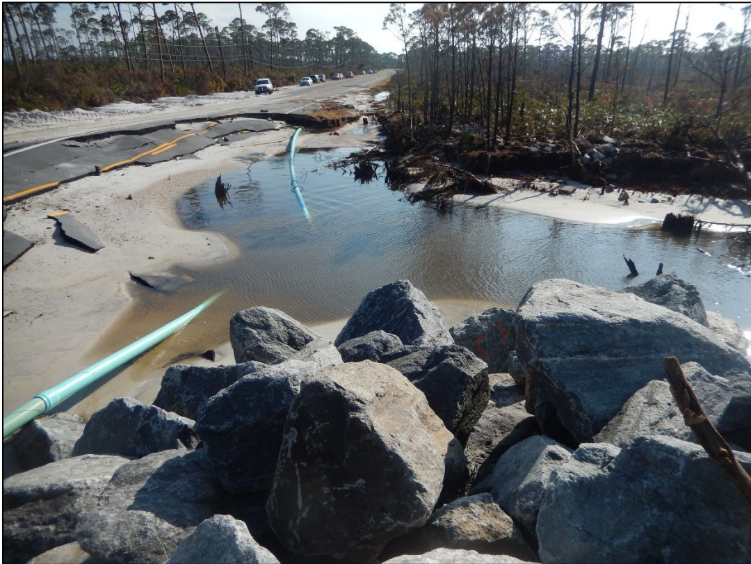
Figure 75. County Road 30E destroyed south of the Stump Hole boulder mound, R107.
