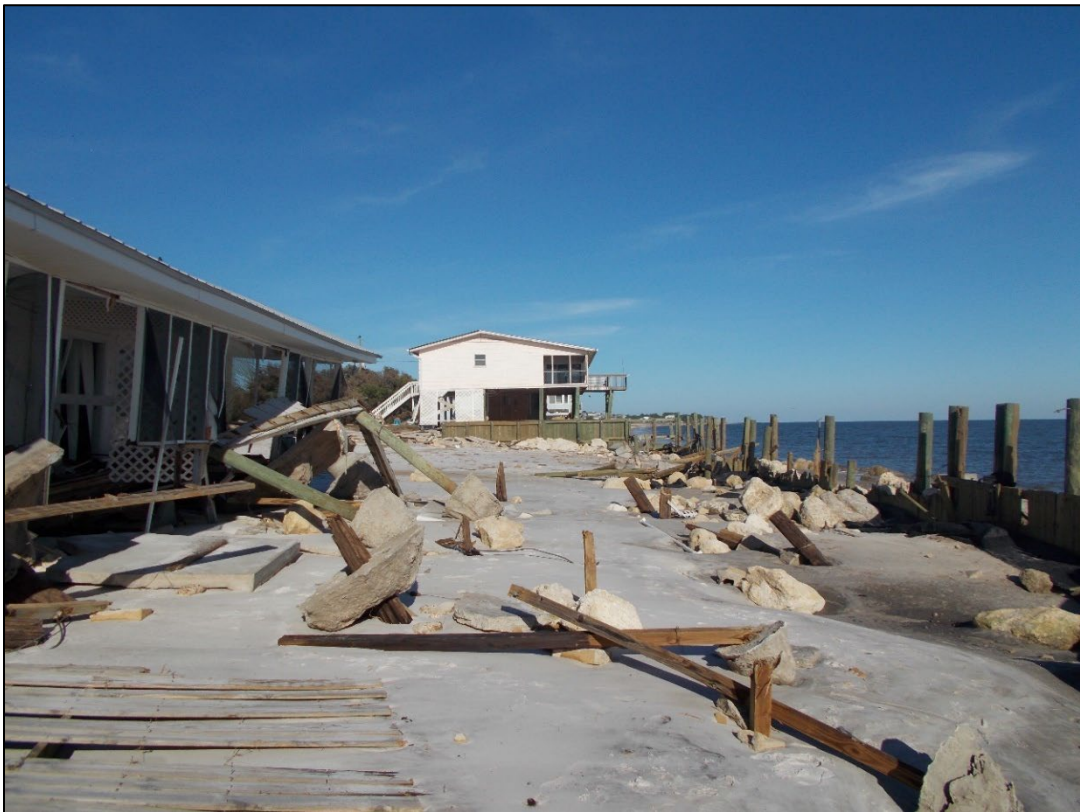
Figure 102. Dwelling and bulkhead damaged near R214.5, Southwest Cape.
