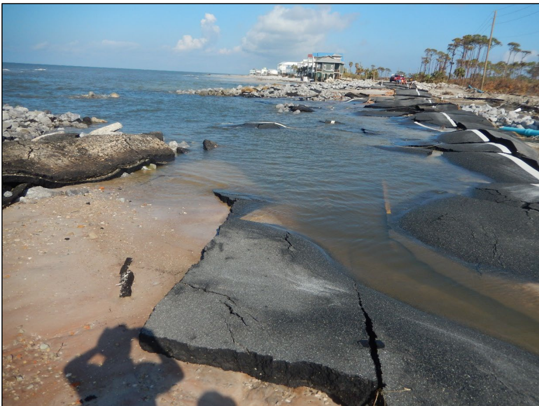
Figure 74. County Road 30E destroyed north of the Stump Hole boulder mound, R105.
