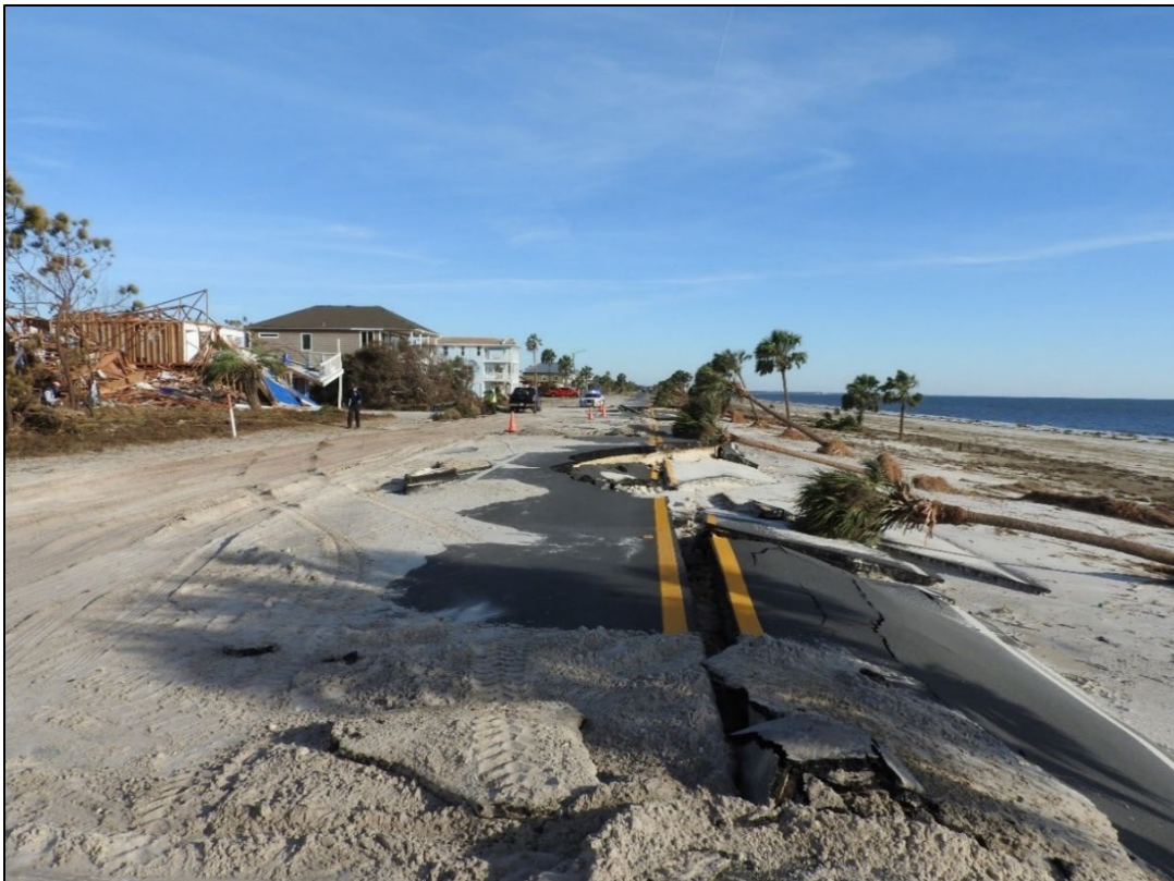
Figure 43. Segment of U.S. 98 destroyed near R139, Mexico Beach.
