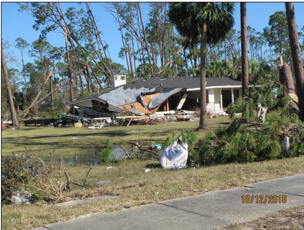
Figure 66. Dwelling destroyed by the storm surge from St. Joseph Bay, Port St. Joe.
