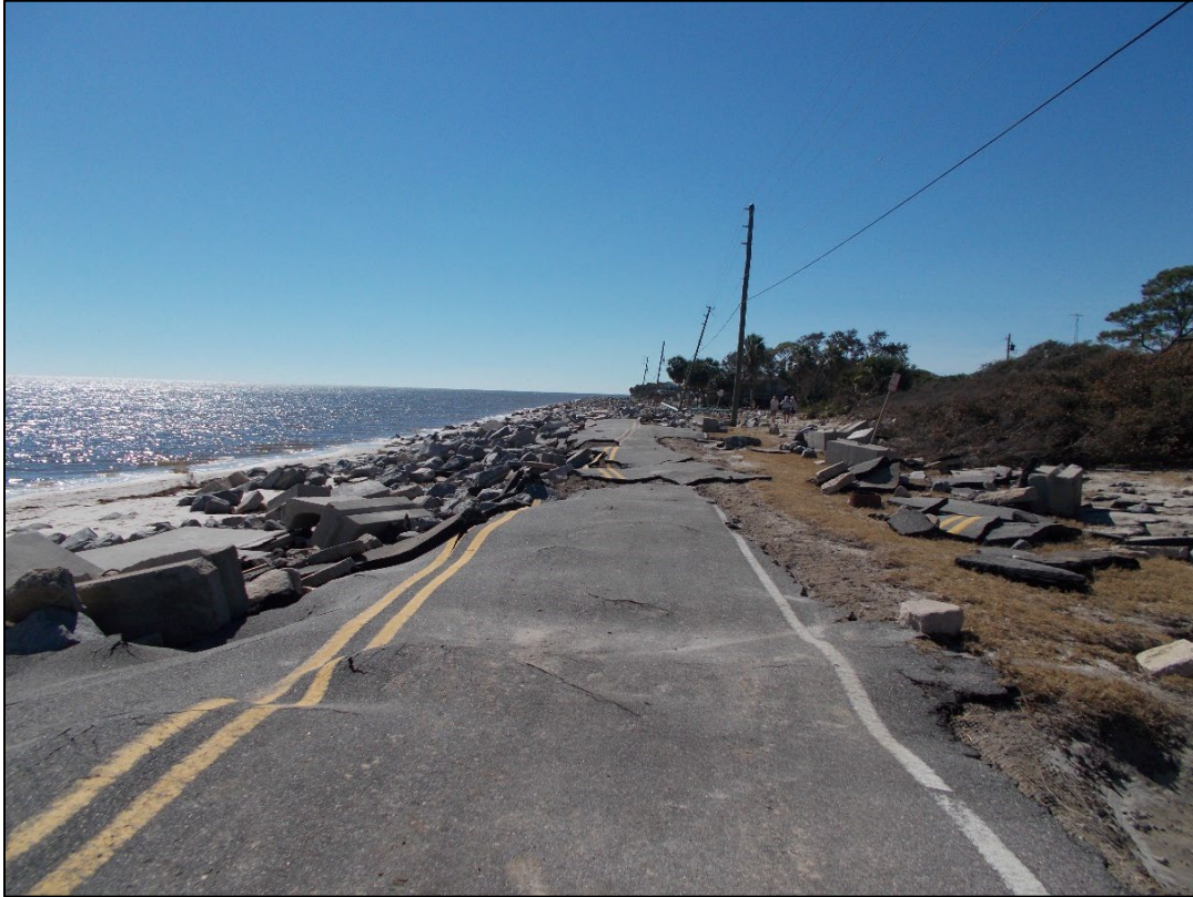
Figure 99. 3,000 feet of road and revetment destroyed between R211-R214, Southwest Cape.
