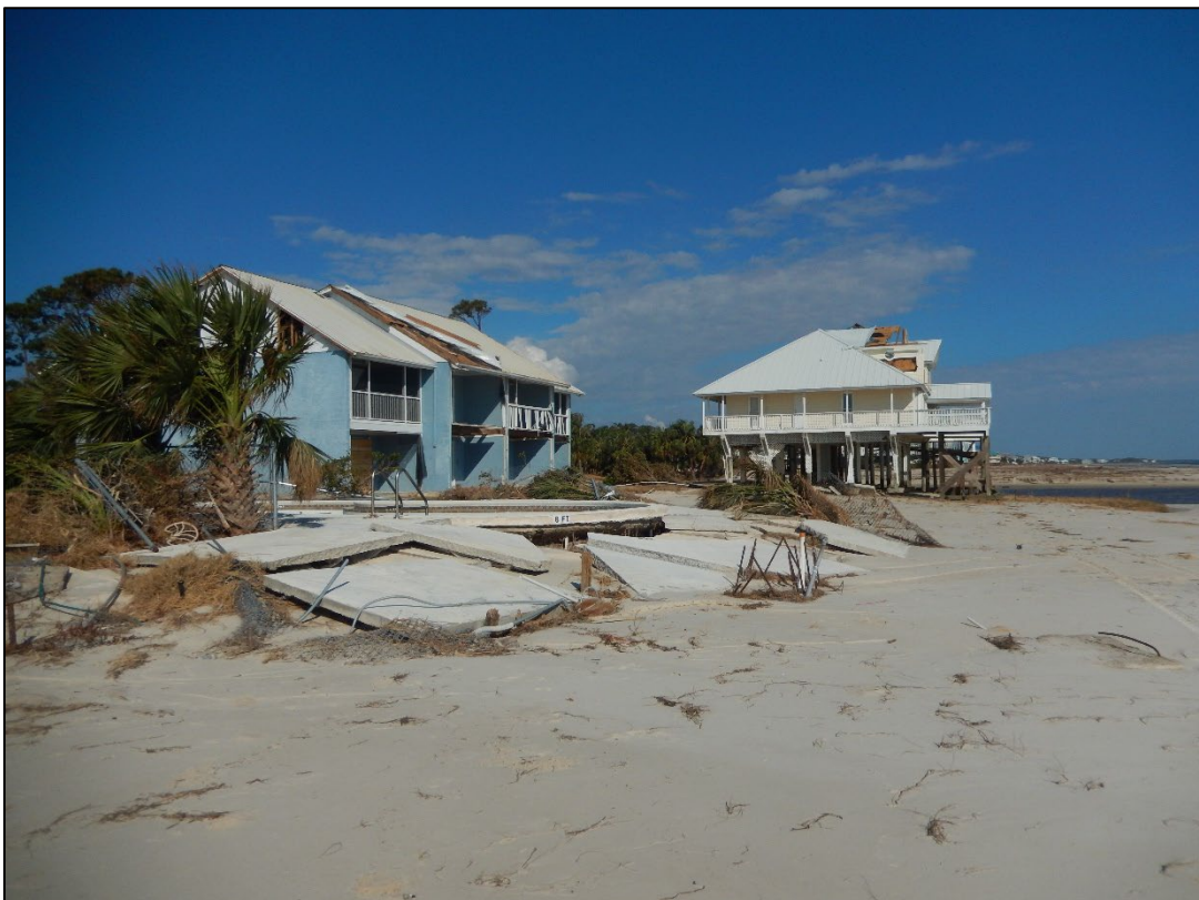
Figure 76. Storm surge damages at Money Bayou, R140.
