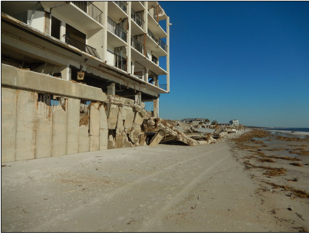
Figure 38. Over 700 feet of reinforced concrete seawall destroyed at R135, Mexico Beach.
