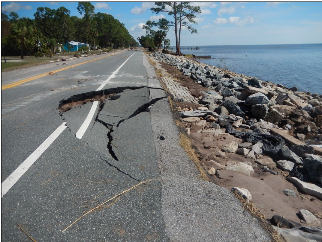
Figure 92. U.S. Highway 98 damaged near Eastpoint.
