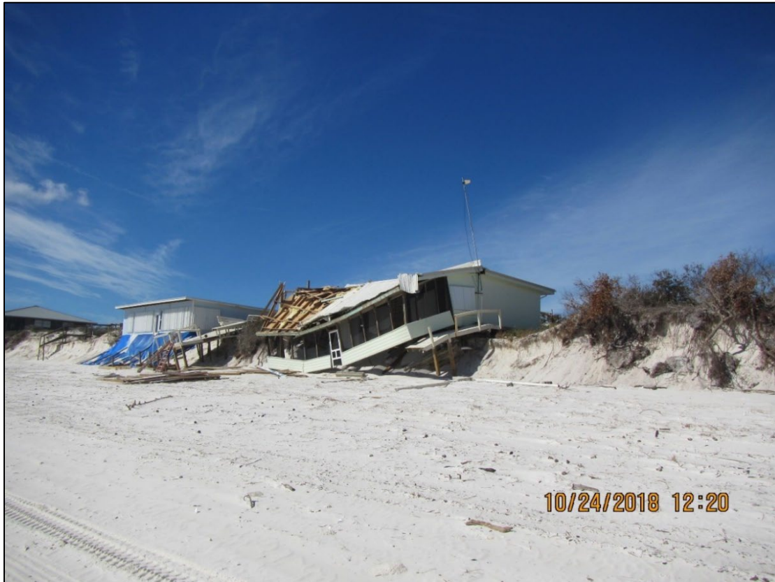
Figure 97. Dwelling destroyed near R179, Dog Island.
