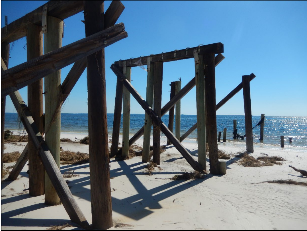
Figure 30. Mexico Beach pier destroyed near R129.
