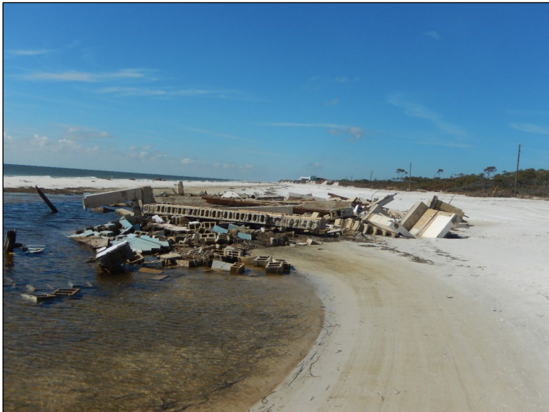
Figure 98. Pelican Inn destroyed near R183, Dog Island.
