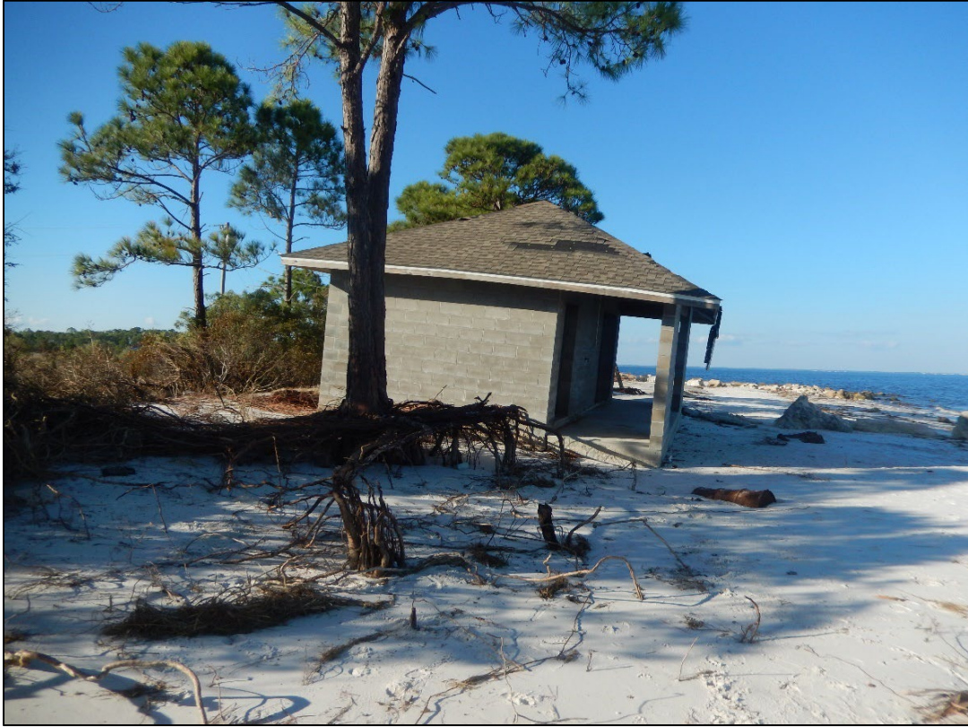
Figure 105. Bathhouse destroyed at Mashas Sands, V314.
