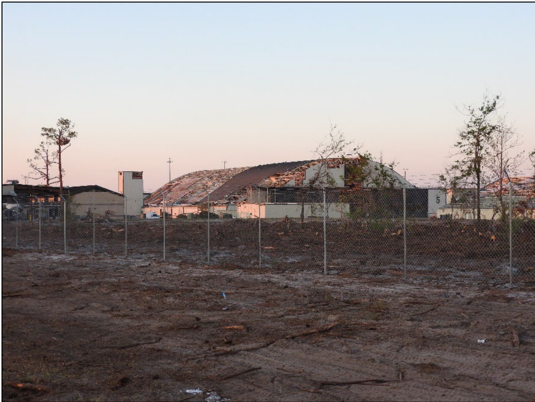
Figure 22. Tyndall Air Force Base, aircraft hangar damage.
