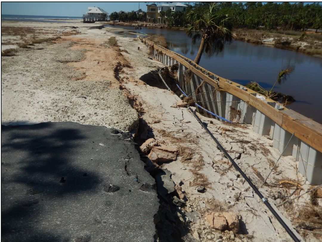
Figure 78. Bulkhead on Money Bayou damaged, R141.
