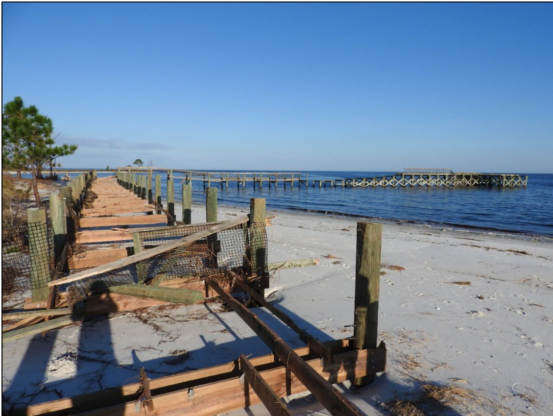
Figure 104. Fishing pier and access walkway damaged at Mashes Sands, V303.
