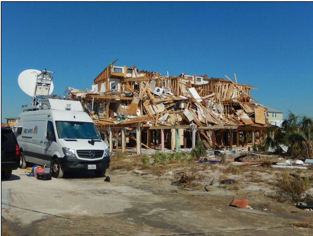
Figure 33. Pile-supported multifamily dwelling destroyed near R129, Mexico Beach.
