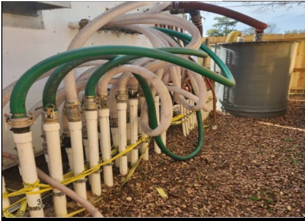
SVE System Stub Up Piping/Flex Hose Connections & Vapor Phase Carbon Vessel
