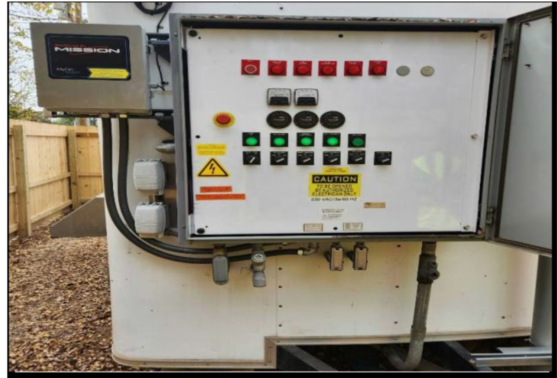
AS/SVE System Control Panel w/ Telemetry
