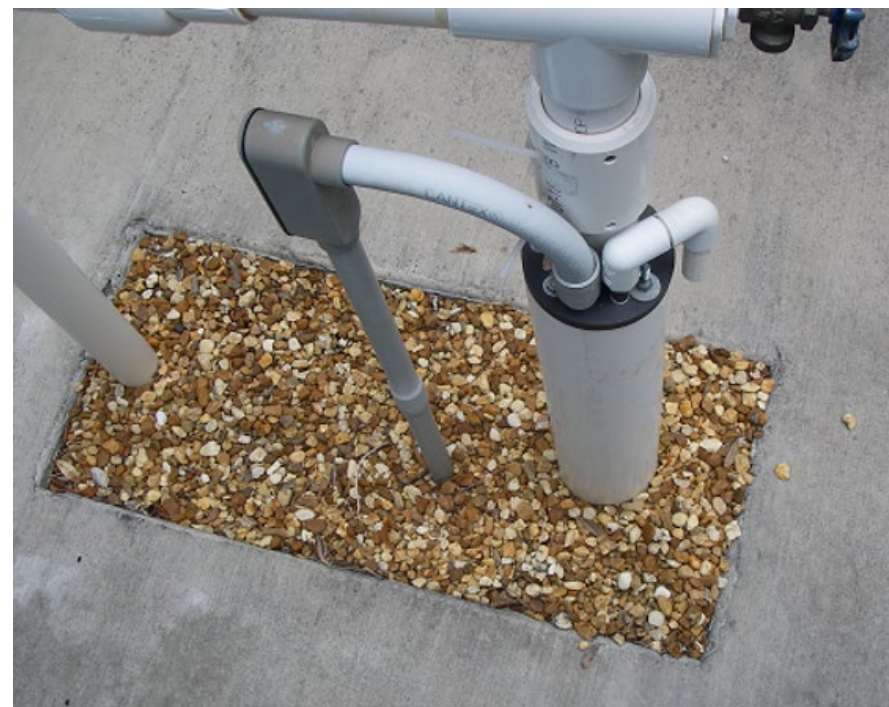
Improper well pad
