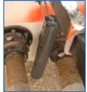
Sensor Float in Dispenser Sump
