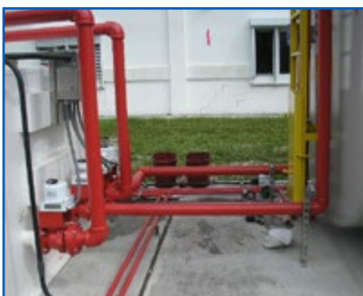
Piping for Shop Fabricated AST
