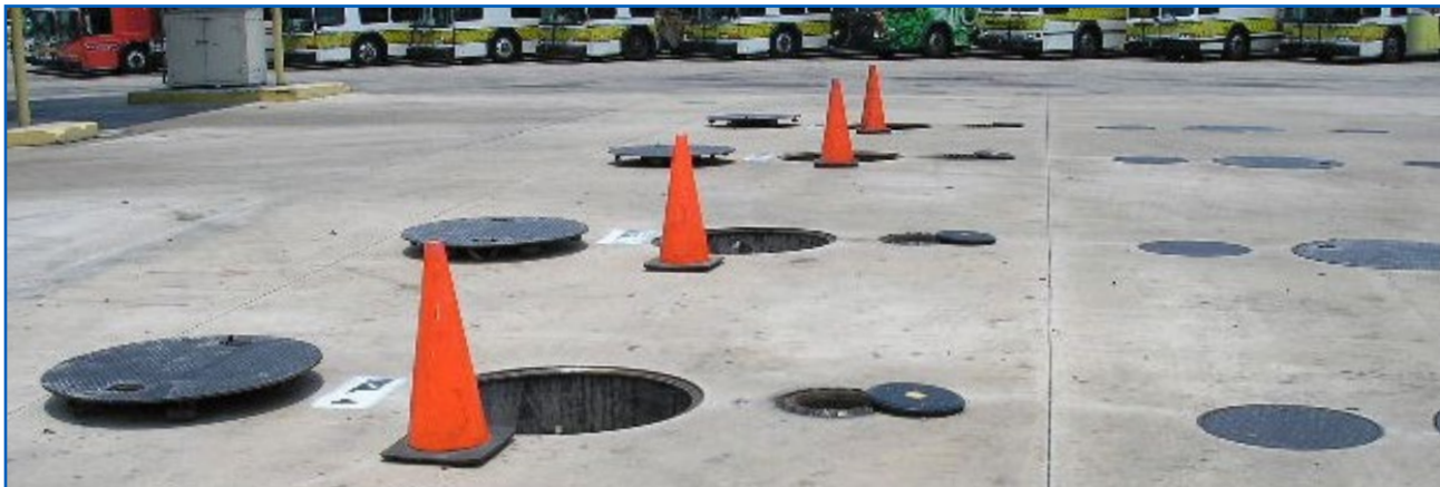
UST Systems with Sump Manway Covers Opened for Inspection
