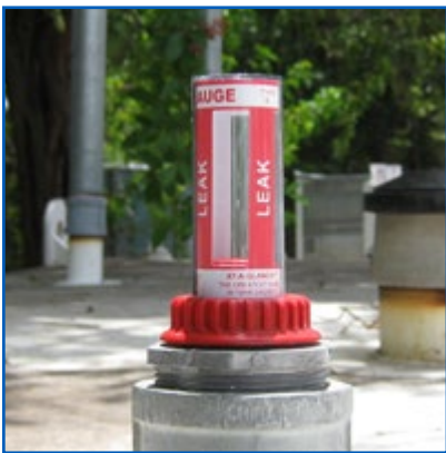
AST Float Gauge Installed
