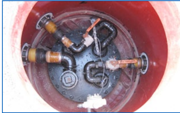
Entry/Test Port Boots Installed
