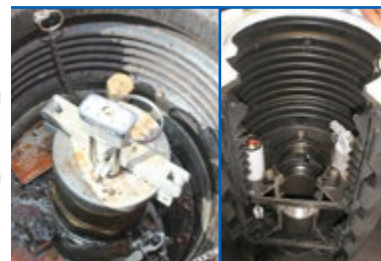
Release Valve in Spill Bucket
