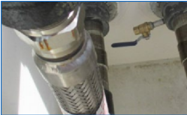
Flex Pipe Fitting in Dispenser Sump
