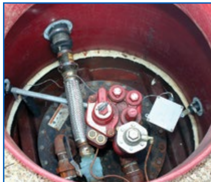
Piping, Pump and LLD inside Sump
