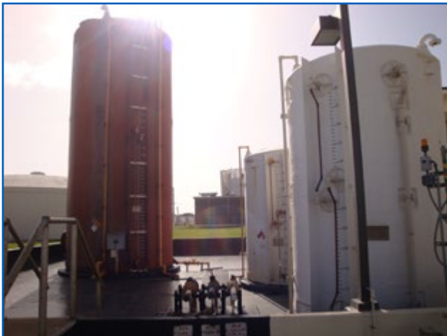
Vertical SW-AST within Secondary Containment
