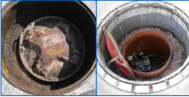
Sump Cover Closed
