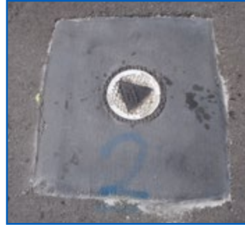
Installed MW with Color-coded Cover
