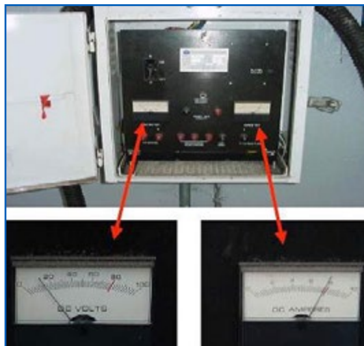
Impressed Current Rectifier with Voltmeter and Ammeter
