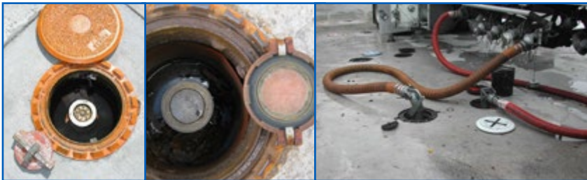
Stage I Vapor Recovery Color-coded Sump
