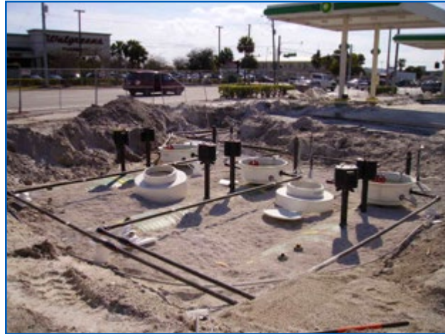
Double-walled Fiberglass Piping Layout
