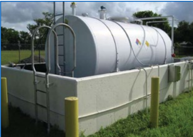
Single-walled Steel AST Inside Concrete Secondary Containment
