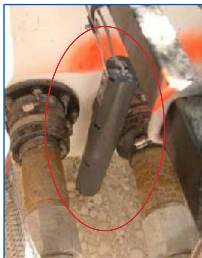
Sensor Placed Near Sump Bottom
