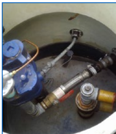
Flex Pipe Fitting in Pump/Piping Sump
