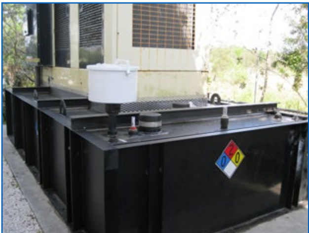
Sub-base DW-Emergency Generator AST
