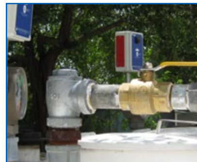
Anti-siphon with Isolation Ball Valve
