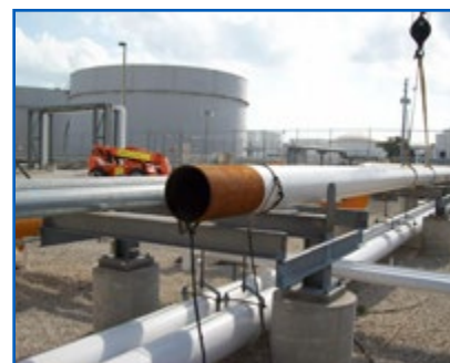
Bulk Product Piping
