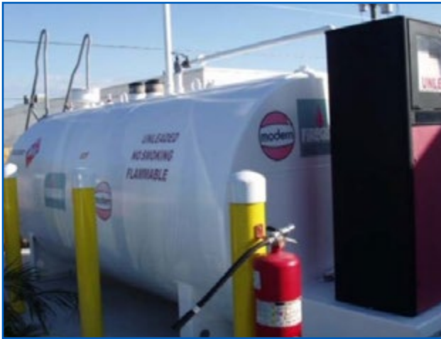
AST with Suction Pump at Dispenser
