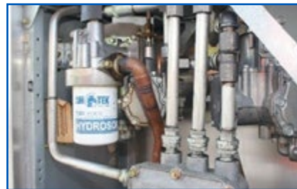
Fuel Filter, Installed in Place
