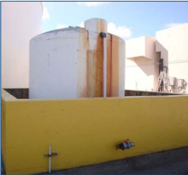
Check Drain Valves for Leaks. Ensure they are Locked when Not in Use
