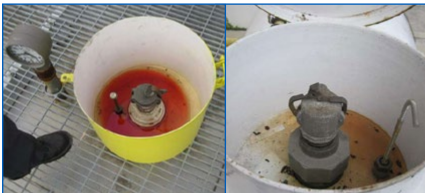
AST Spill Containment with Release Valve on Tank Top
