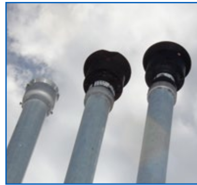
Vent Valves Extend 12 feet Above Grade
