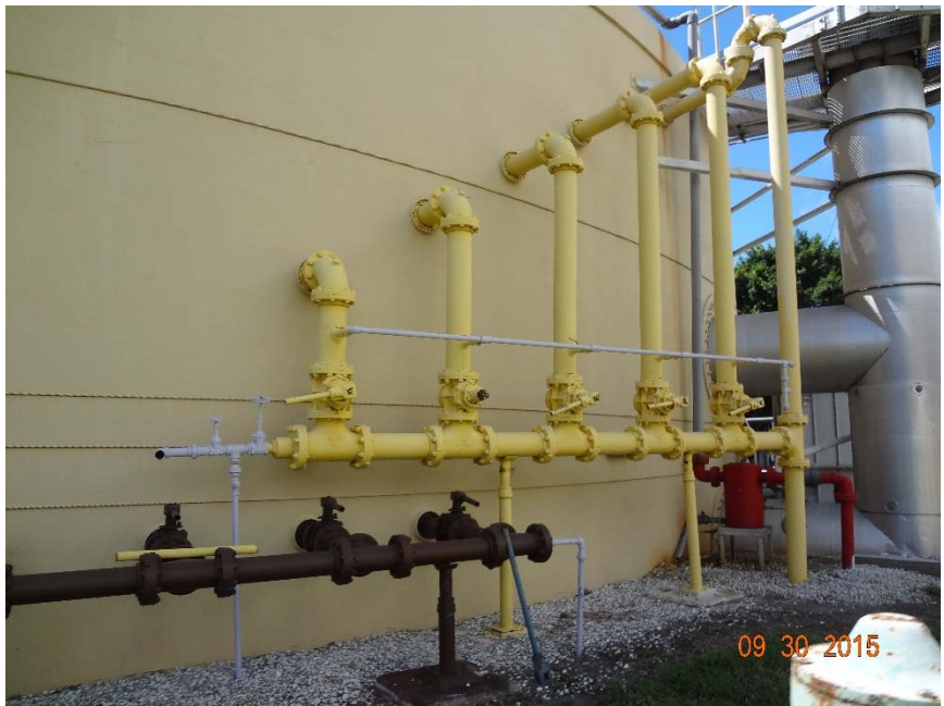
Figure SWWRF-6. Anaerobic Digester Decant No. 3 Piping and Draft Tube Mixer Southwest WRF
