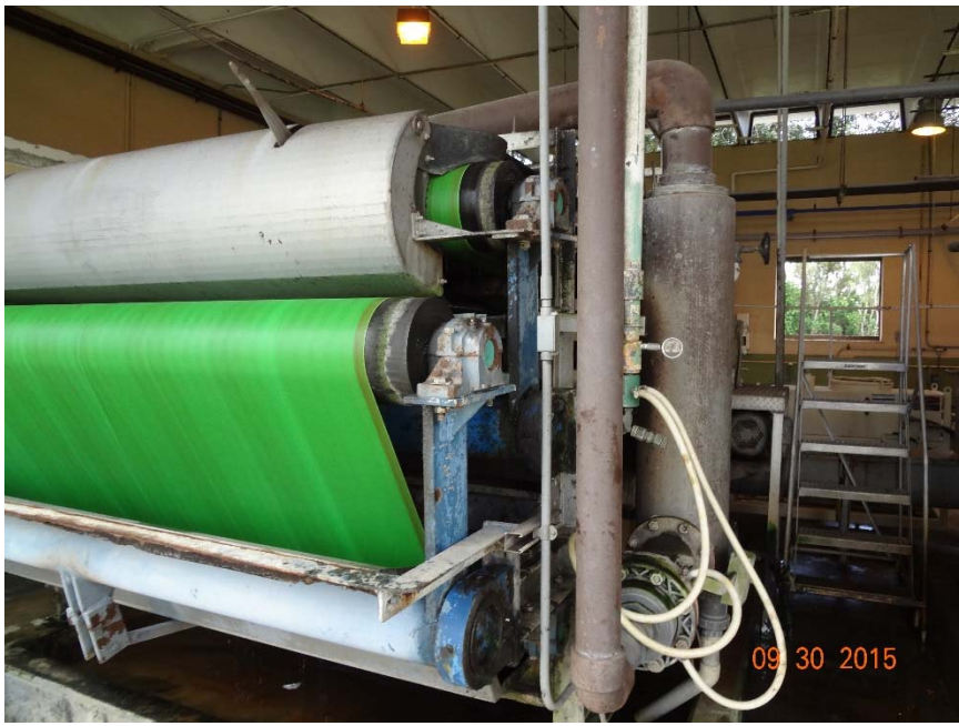
Figure SWWRF-7. Belt Filter Press Southwest WRF
