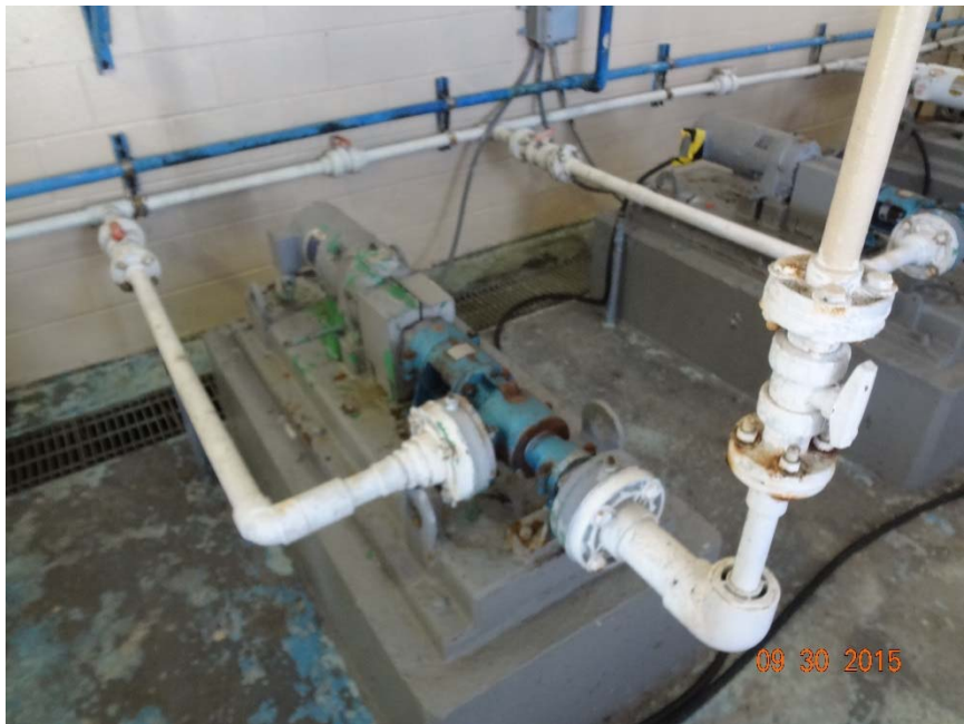
Figure NWWRF-14. Dewatering Polymer Pumping Northwest WRF
