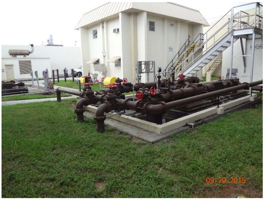
Figure NEWRF-7. Sludge Feed Pump Station Northeast WRF
