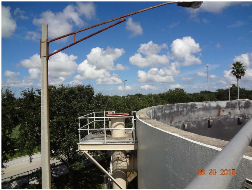
Figure NWWRF-7. Anaerobic Digester No. 4 Draft Tube Mixer Northwest WRF
