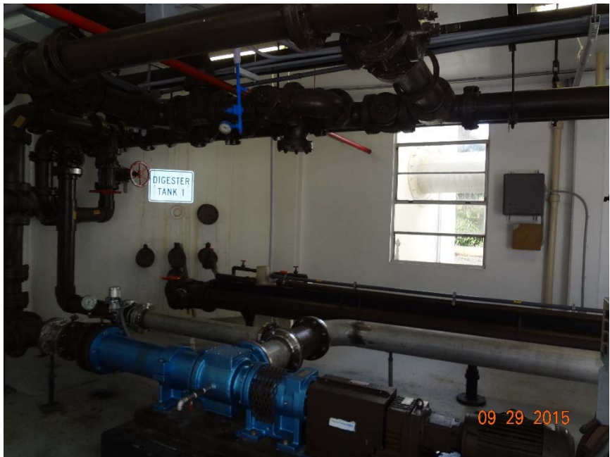
Figure NEWRF-4. Anaerobic Digesters No. 1 and No. 2 Pumping Northeast WRF
