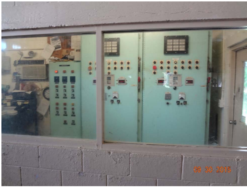
Figure NWWRF-13. Belt Filter Press Electrical Room Northwest WRF
