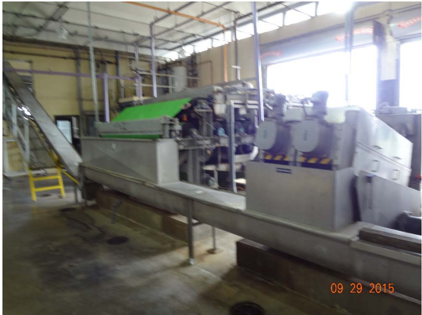
Figure NEWRF-8. Dewatering Building Northeast WRF
