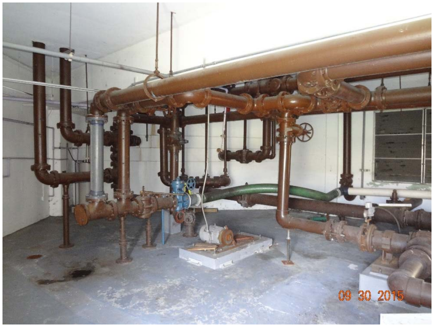
Figure SWWRF-5. Anaerobic Digester No. 1 and No. 2 Piping Southwest WRF
