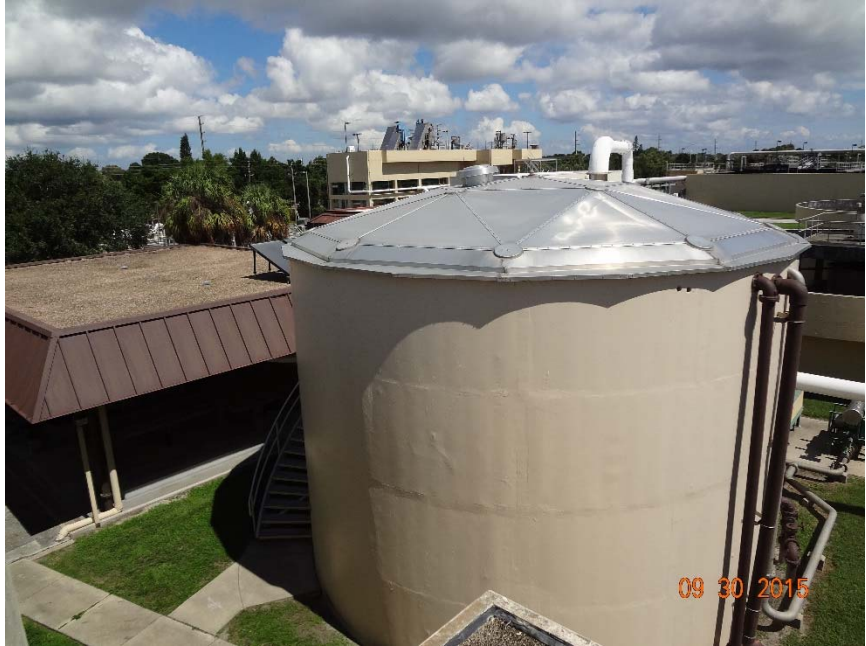
Figure SWWRF-1. Sludge Storage Tank Southwest WRF
