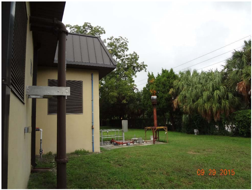
Figure NEWRF-5. Anaerobic Digester Gas Flare Northeast WRF
