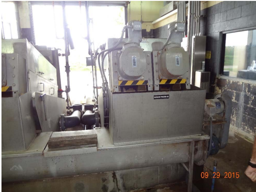
Figure NEWRF-10. Screw Presses Northeast WRF
