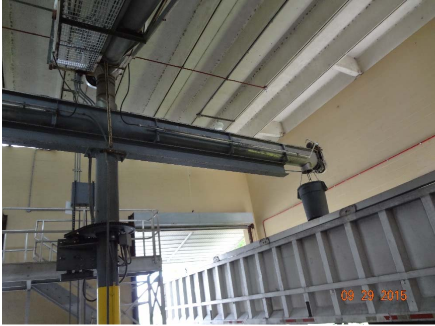
Figure NEWRF-12. Truck Loading Northeast WRF
