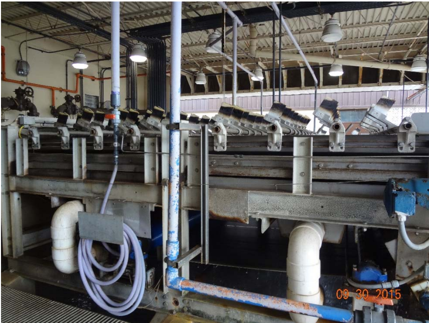
Figure NWWRF-1. Gravity Belt Thickener Northwest WRF
