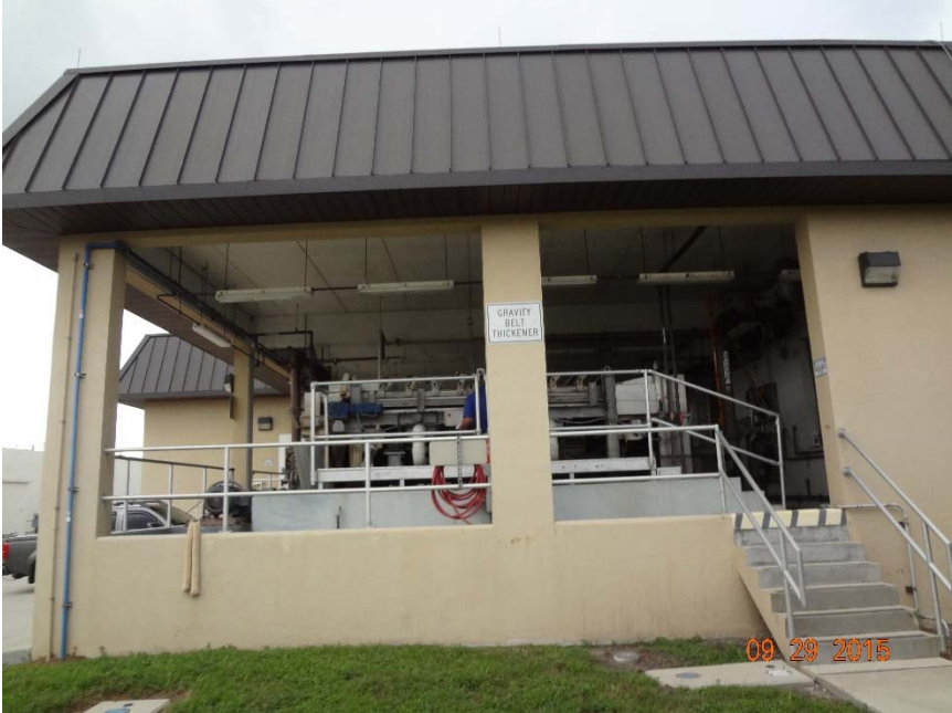
Figure NEWRF-1. Gravity Belt Thickener Northeast WRF
