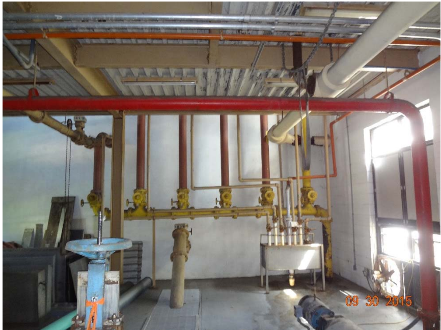
Figure NWWRF-8. Anaerobic Digesters No. 3 and No. 4 Building Second Floor Northwest WRF
