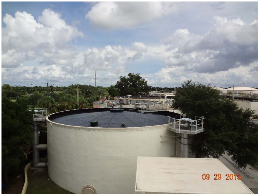
Figure NEWRF-3. Anaerobic Digester No. 1 Northeast WRF
