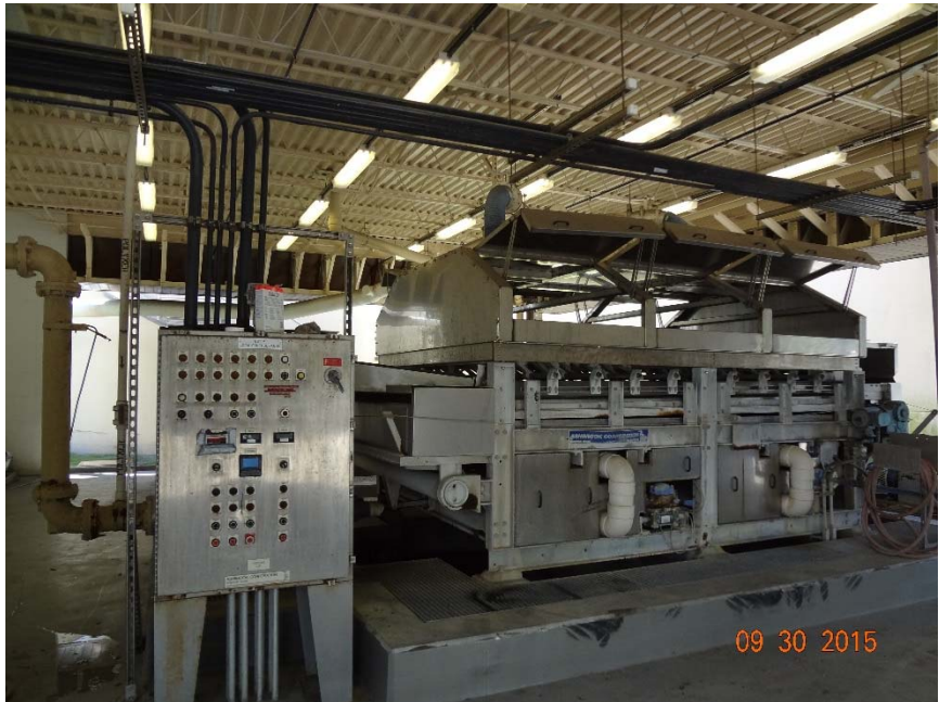
Figure SWWRF-2. Gravity Belt Thickener Southwest WRF
