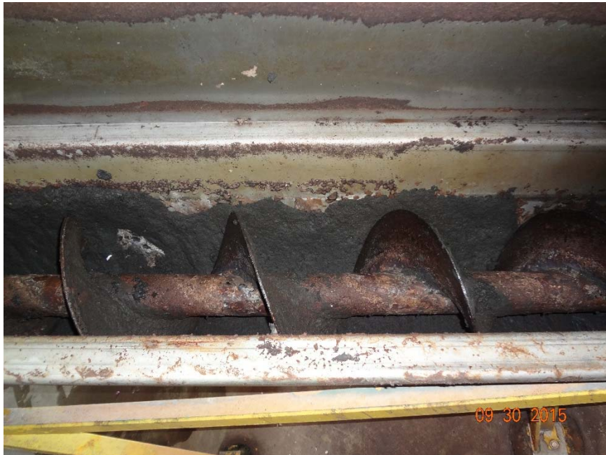
Figure NWWRF-16. Dewatered Sludge Conveyor Northwest WRF
