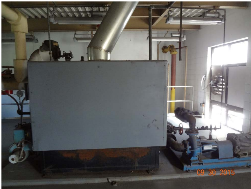
Figure NWWRF-9. Anaerobic Digesters No. 3 and No. 4 Gas-fired Heater Northwest WRF
