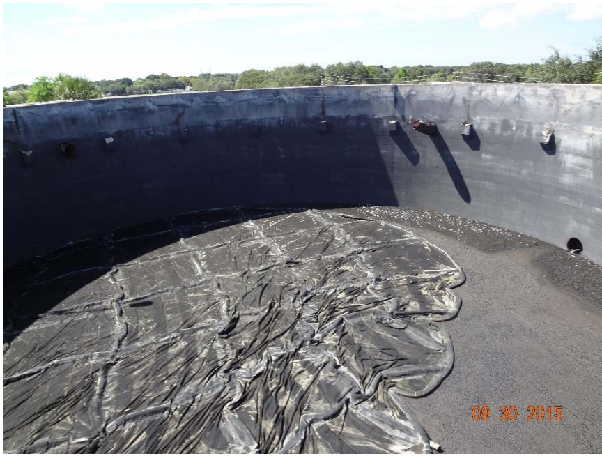
Figure NWWRF-5. Anaerobic Digester No. 3 Northwest WRF
