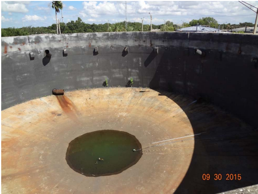
Figure NWWRF-6. Anaerobic Digester No. 4 Northwest WRF
