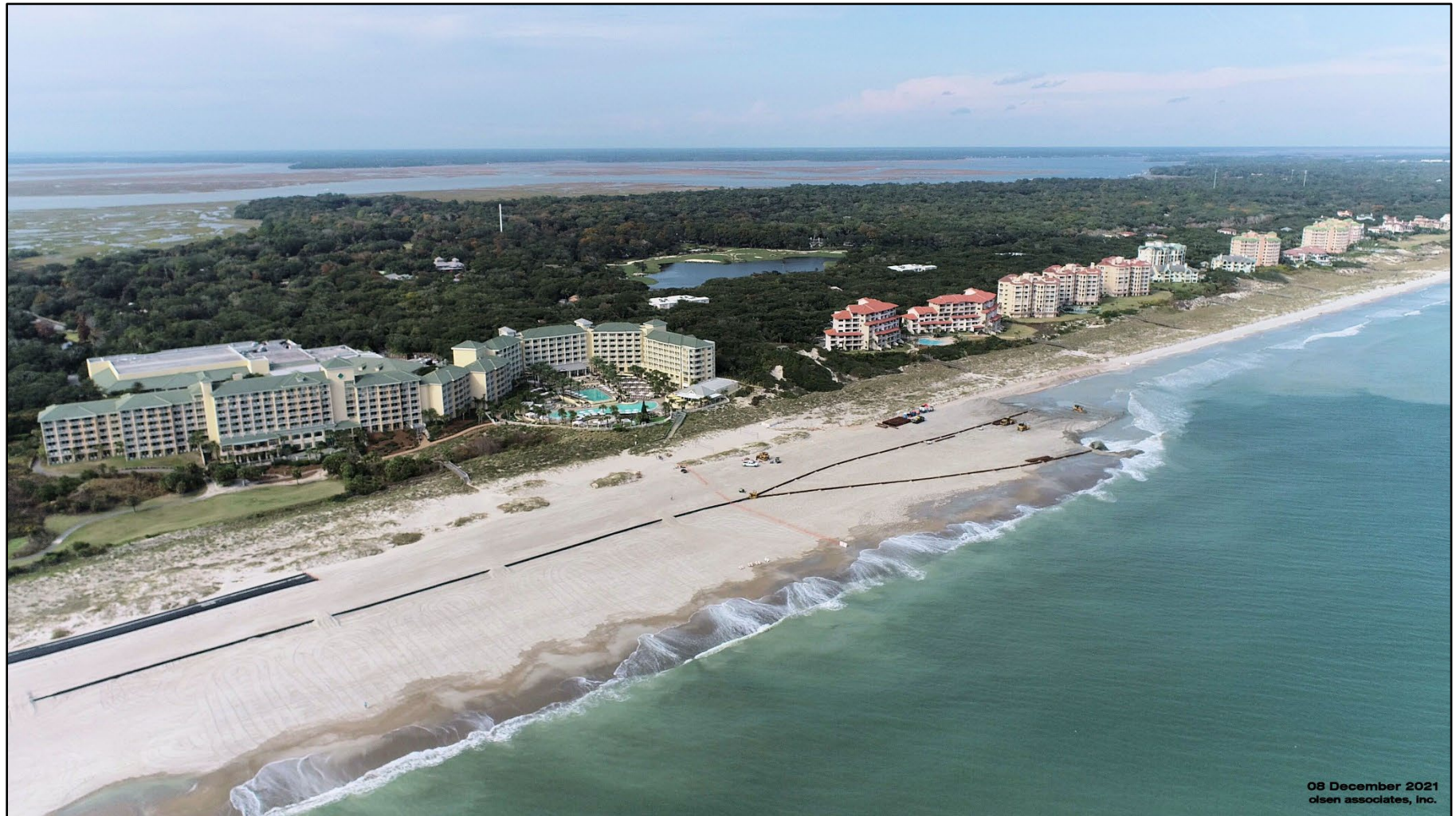
South Amelia Island Beach Nourishment Project being constructed in December 2021 and sponsored by SAISSA. Photo courtesy of Al Browder with Olsen Associates. See additional construction photos of beach nourishment projects.
