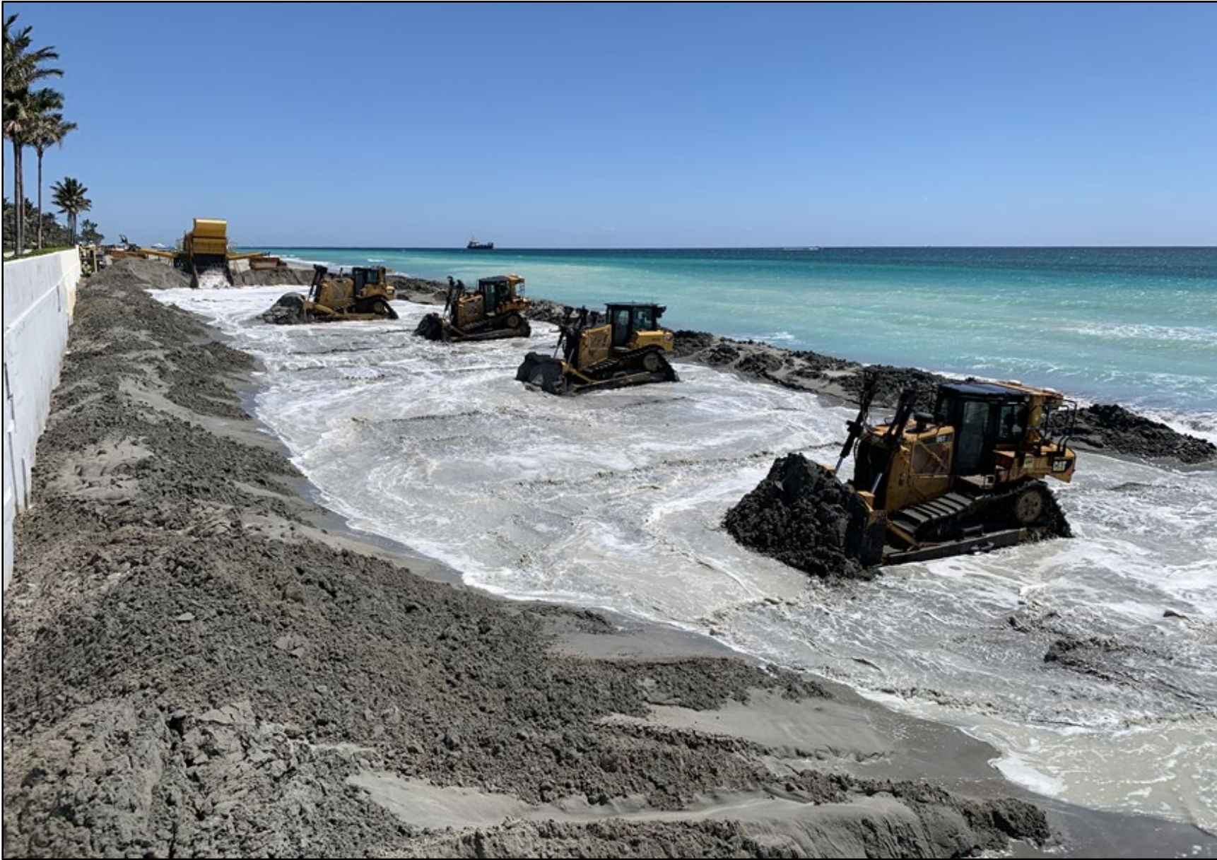
Mid-Town Beach Nourishment Project under construction in April 2020. Photo courtesy of Rob Weber, Town of Palm Beach. See additional construction photos of beach nourishment projects.
