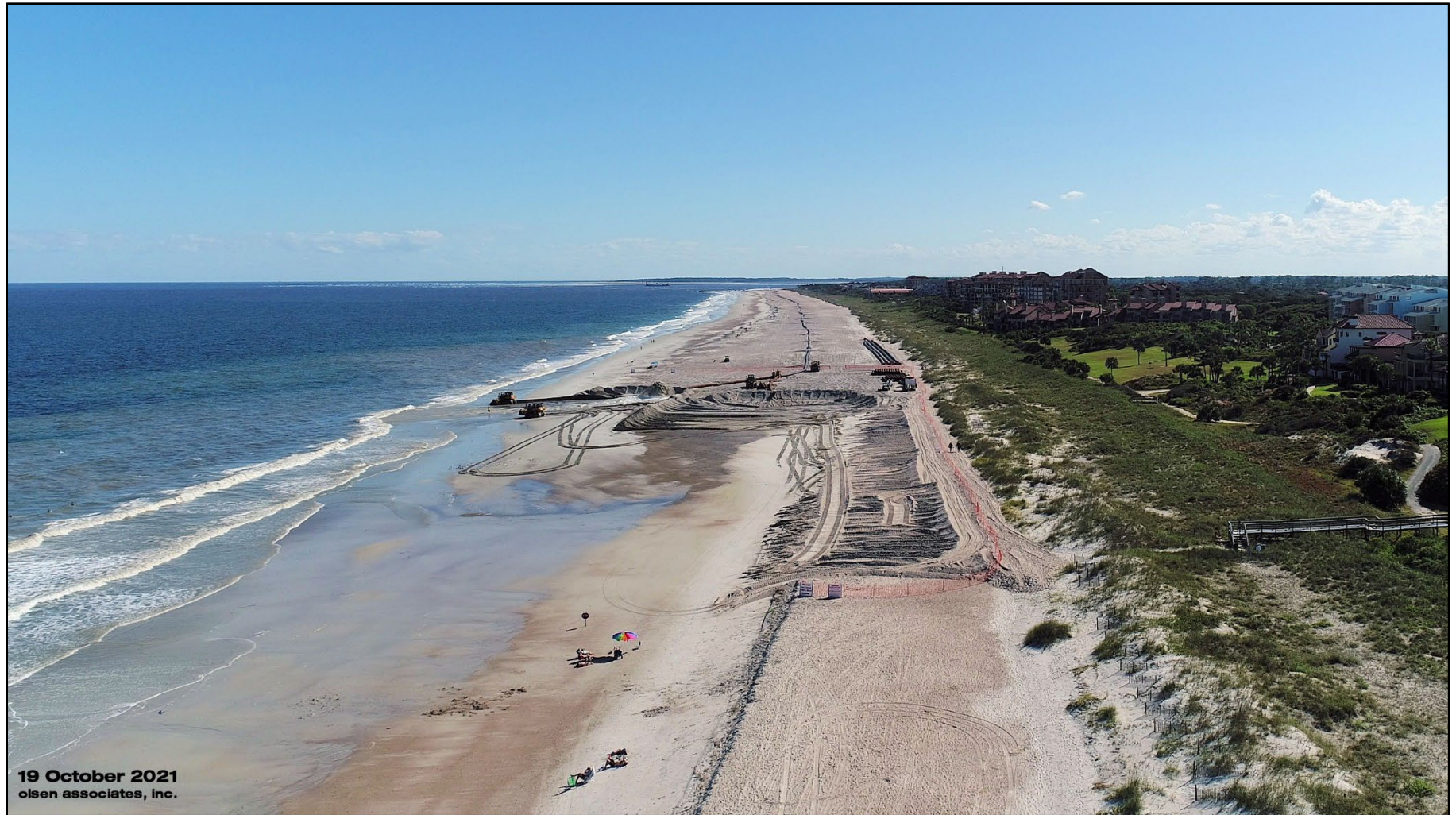
The South Amelia Island Beach Nourishment Project being constructed in October 2021 and sponsored by SAISSA. Photo courtesy of Al Browder with Olsen Associates. See additional construction photos of beach nourishment projects.
