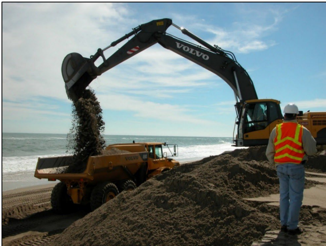
Figure 13. Wabasso Beach (Indian River County) nourishment project (Sector 3) using sand from upland sources. DEP project file photo (2010).
