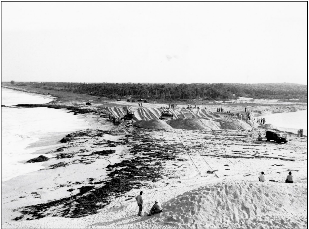
Figure 5. Work began again in 1947 using US Navy demolitions to open the Sebastian Inlet and closed again but was reopened in late 1948 and has been open ever since (Sebastian Inlet District, 2019).
