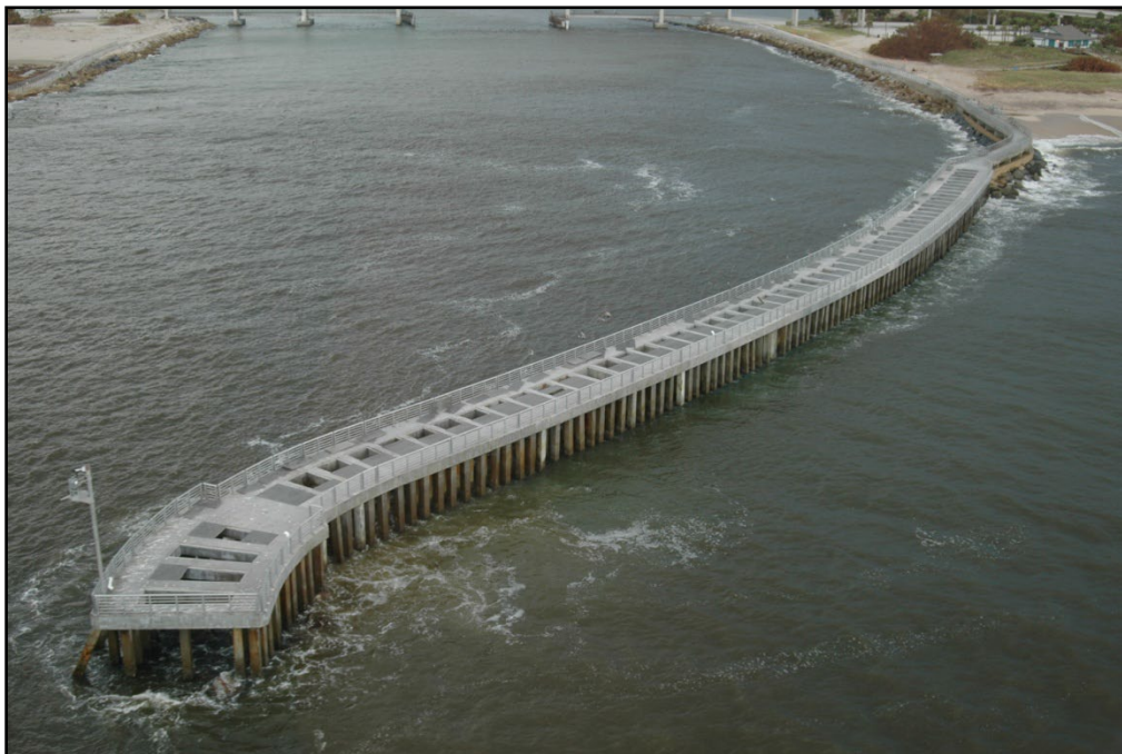
Figure 10. Sebastian Inlet North Jetty Pier lost breakaway grates during Hurricane Frances, 2004.
