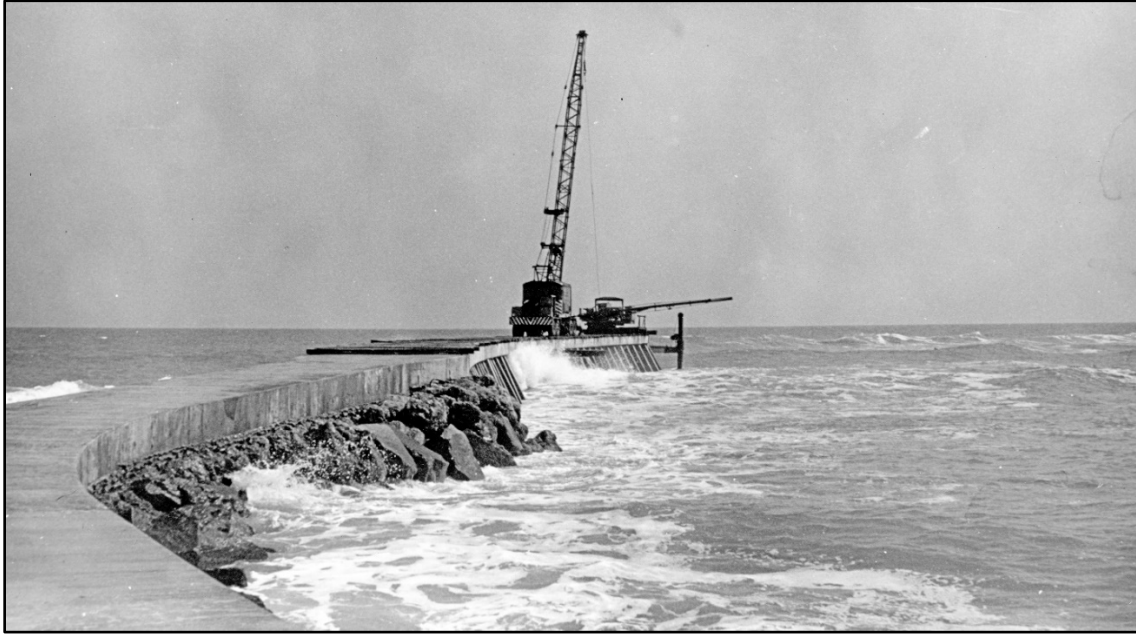
Figure 8. Construction crane working on the north jetty of Sebastian Inlet in 1969 (Sebastian Inlet District, 2019).
