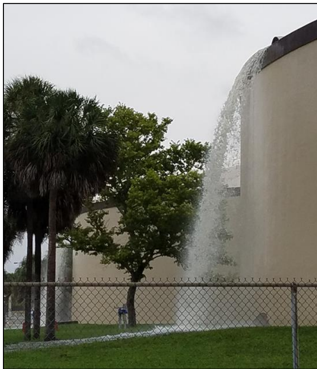
Figure 1. NWWRF reclaimed and reject water tanks overflowing
