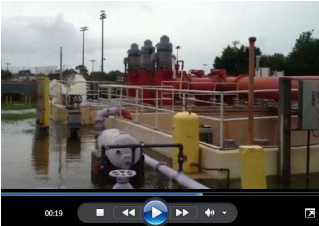
Figure 3. Video of Southwest Plant Chlorine Contact Tank overflowing during Hurricane Hermine
