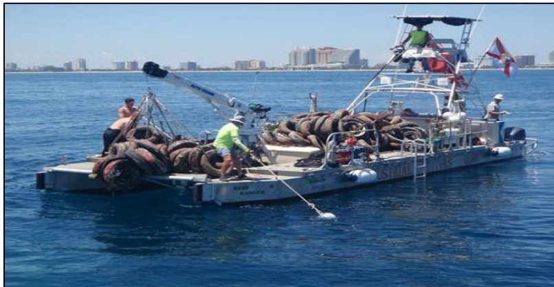
Image 10. Current commercial tire removal operation using a similar method to that used during the DoD Program. Once the support vessel is loaded with approximately 300 tires, the vessel will return to Port Everglades to offload the tires into an open-top container (Photo: IDC).
