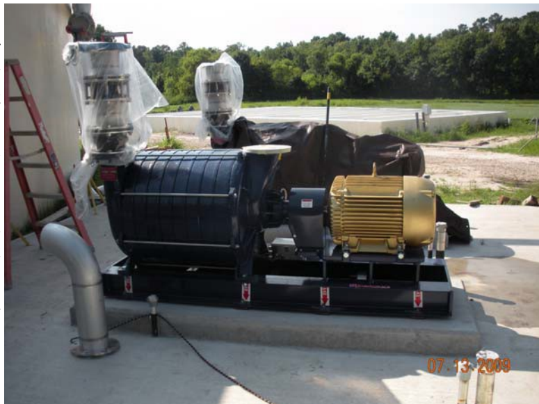
Figure 15: Spencer Multi-stage Blowers for Plant #3
