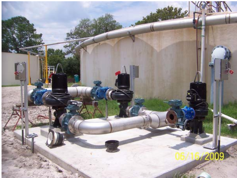
Figure 20: Plant #3 RAS/WAS Pumping station
