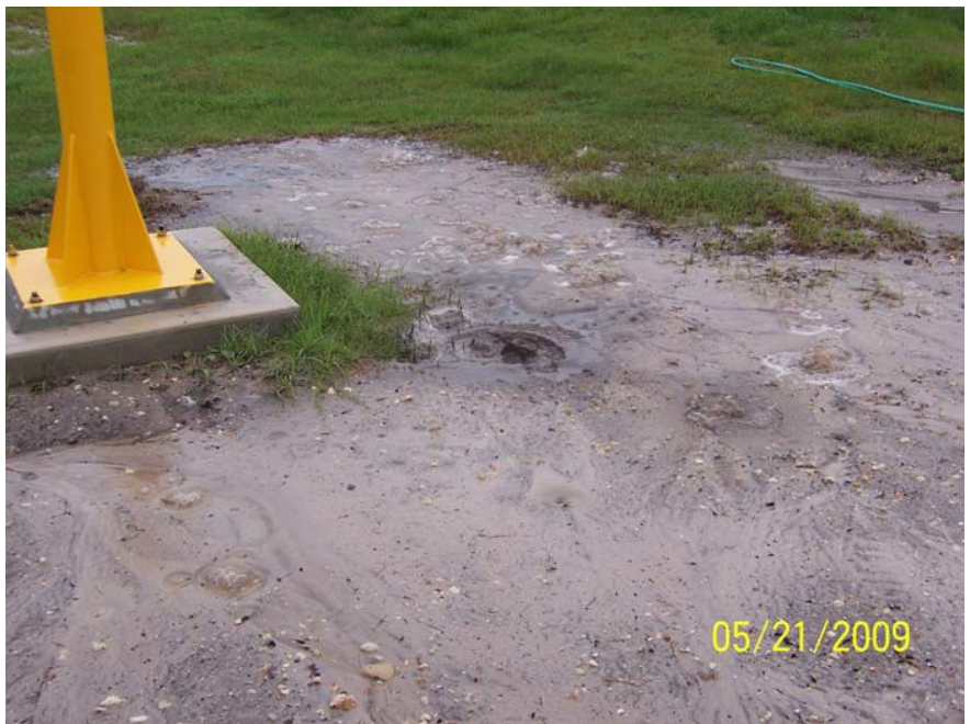
Figure 11: Air leakage from underground air piping could be detected 100 feet away from the lay of the pipe.
