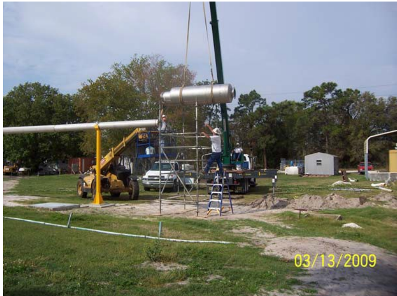
Figure 14: Installation of the inline muffler/silencer
