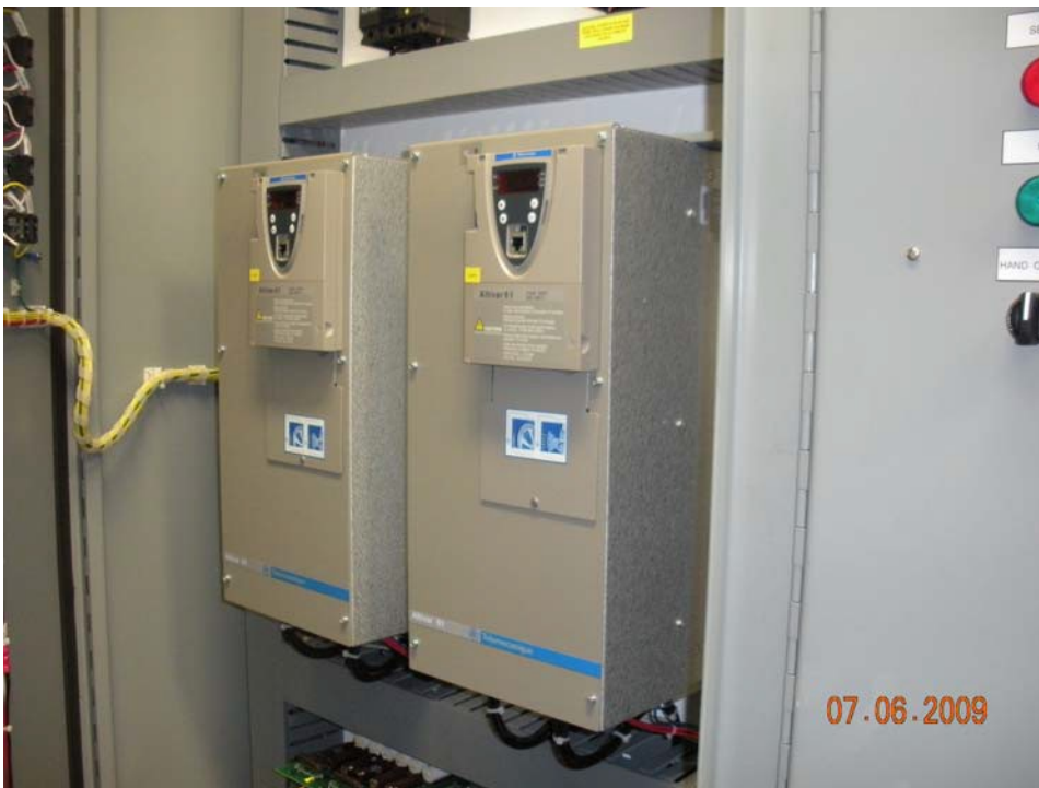
Figure 19: Variable frequency drives for Blowers #7 & 8
