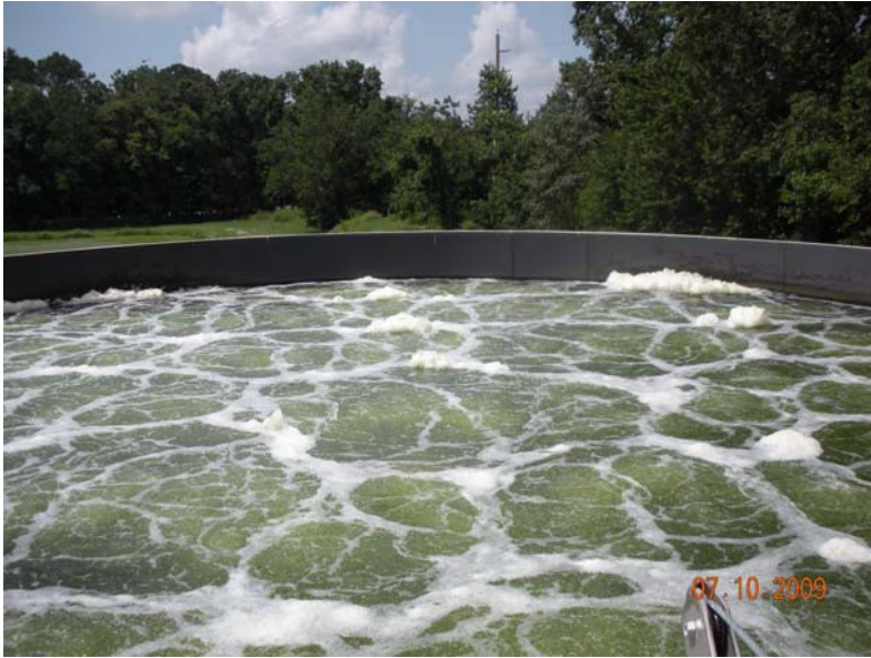
Figure 7: Coarse bubble distribution pattern in Digester #2 during leak testing
