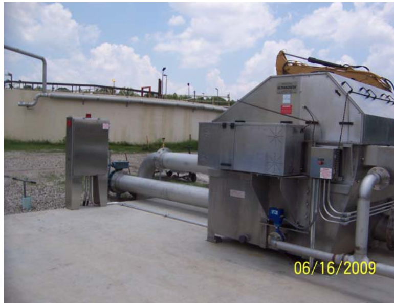
Figure 1: Nova UL1605 Tertiary Plant
