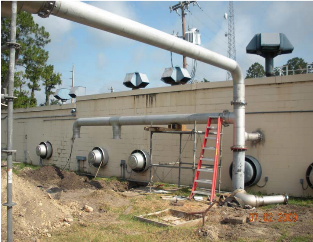
Figure 12: Overhead air header system connection to existing blowers#4, 5, & 6
