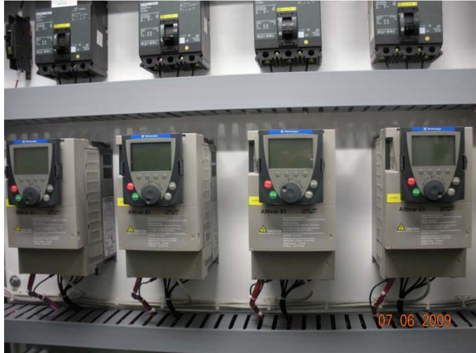
Figure 18: Variable frequency drives for RAS
