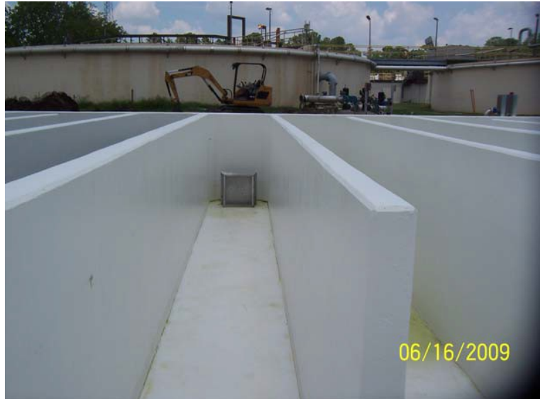
Figure 3: Chlorine contact chamber channel with stainless steel diffuser baffle at influent
