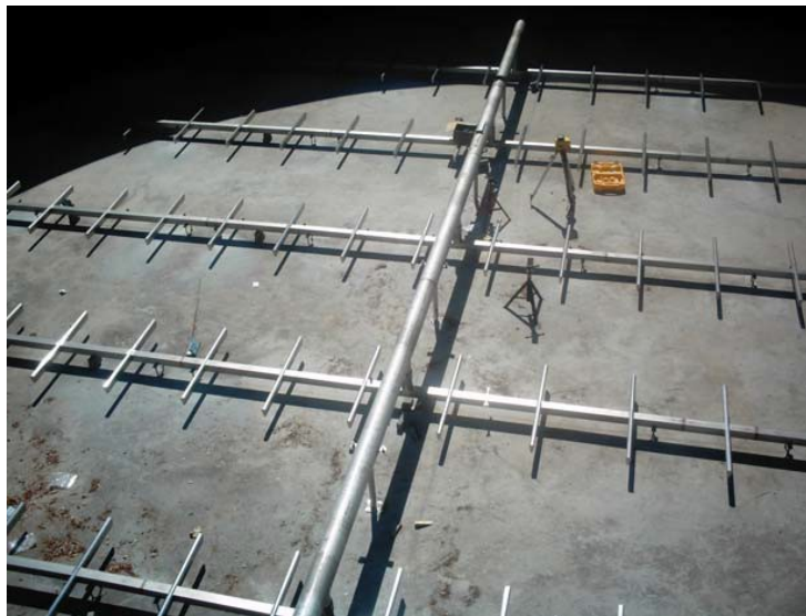
Figure 6: ICBA Coarse Bubble diffuser array in Digester #2
