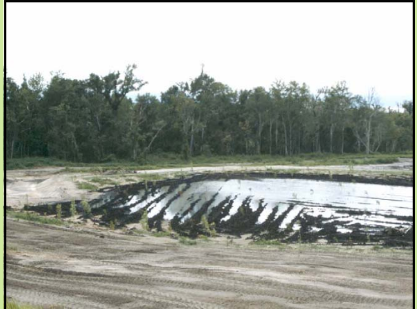
Recently constructed wetland adjacent to forested riparian wetland, showing some topographic relief resulting from dozer tracks (MTB).
