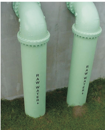
Influent lines at the Peace River Regional Water Treatment Plant in DeSoto County.
