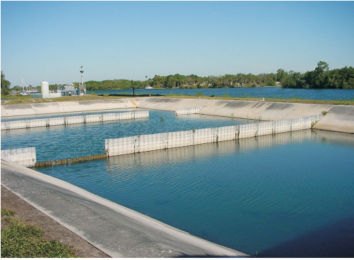
Sludge settling ponds at Lee County Utilities' Olga Water Treatment Plant. Waste streams produced during treatment are allowed to settle in these ponds. The relatively clear water overlying the settled material is returned to the head of the plant.
