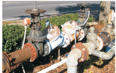
Double check valve assembly outside an office complex in Tallahassee, Leon County.
