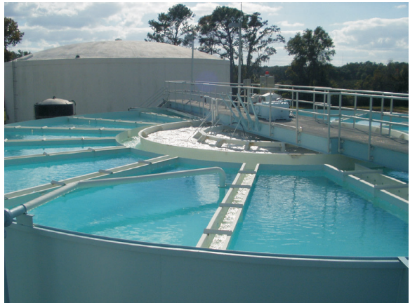
Clarifier at the City of Ocala's Water Treatment Plant in Marion County. This clarifier combines mixing, coagulation, flocculation, sedimentation, and softening in a single tank.
