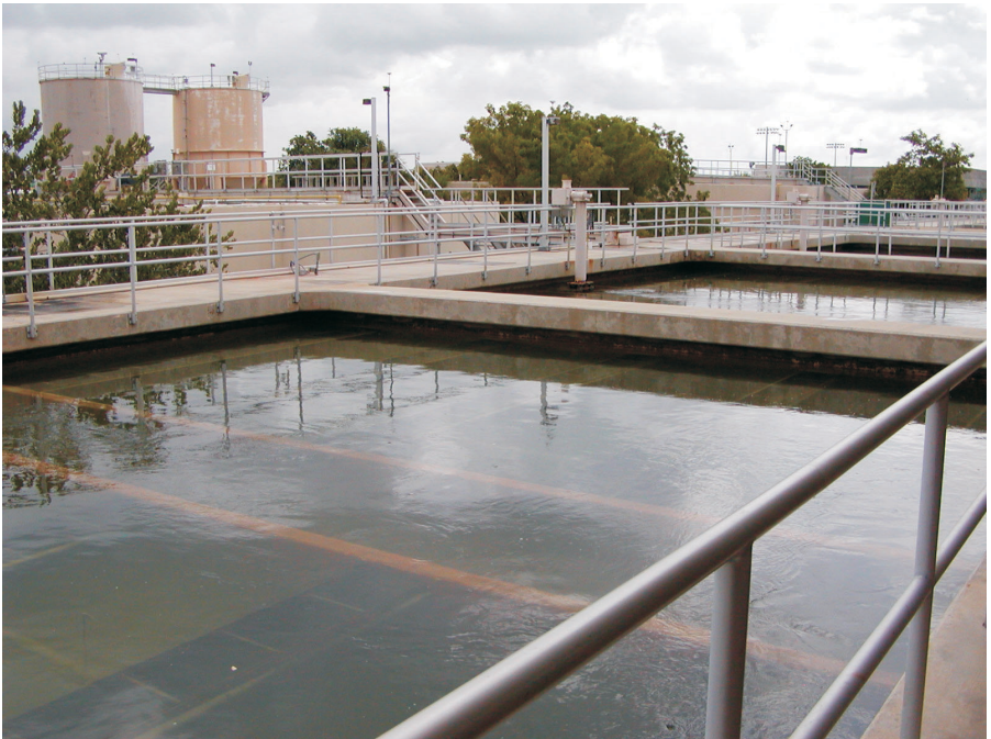
Filter at the City of Boca Raton's Water Treatment Plant in Palm Beach County.
