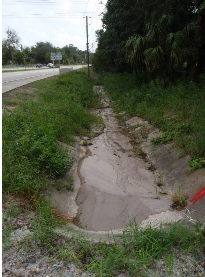
Figure 5.7. Stormwater Drain Flowing into Gee Creek at Station 21FLCEN 20010185
