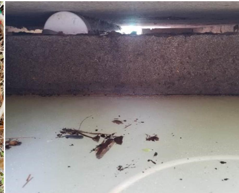
Top of distribution pipe is higher than the top of the baffle wall
