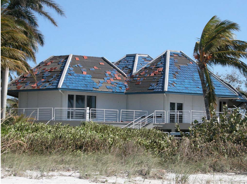
Photo 15. Roofing damage to dwelling, Hideaway Beach (V14.7).
