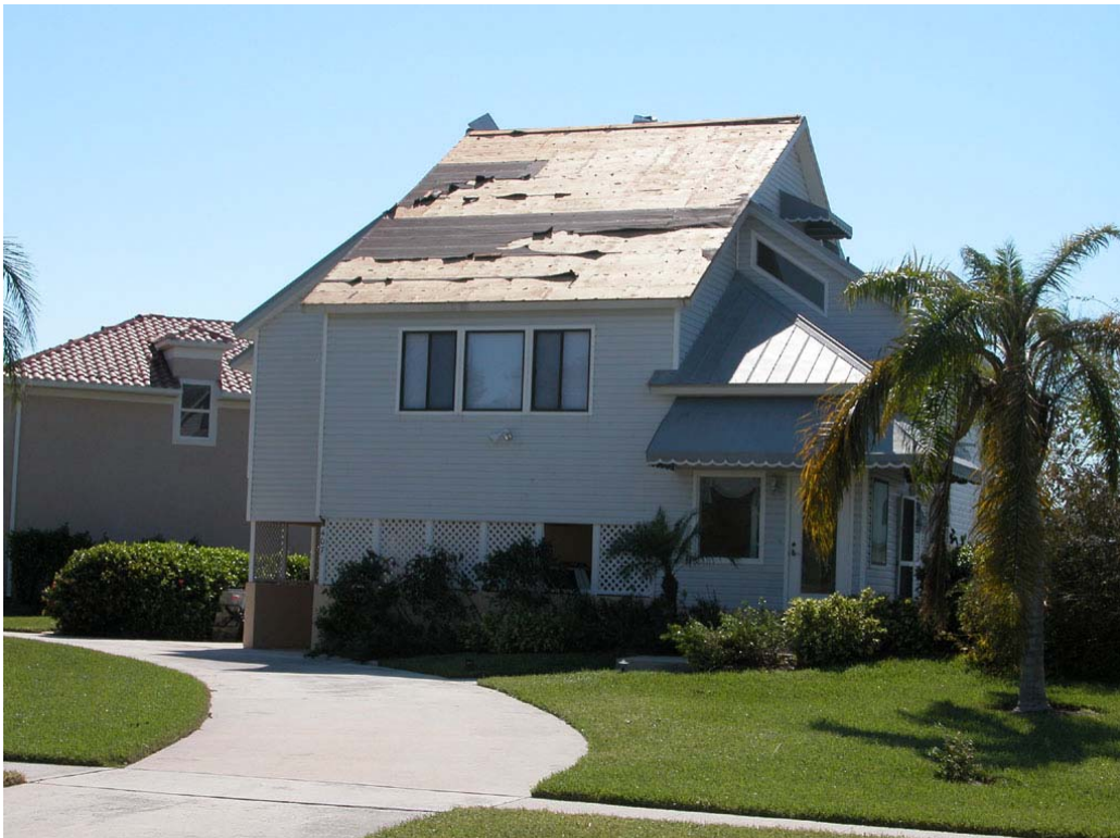
Photo 16. Extensive roofing damage, Tiger Tail Beach (R132.3).
