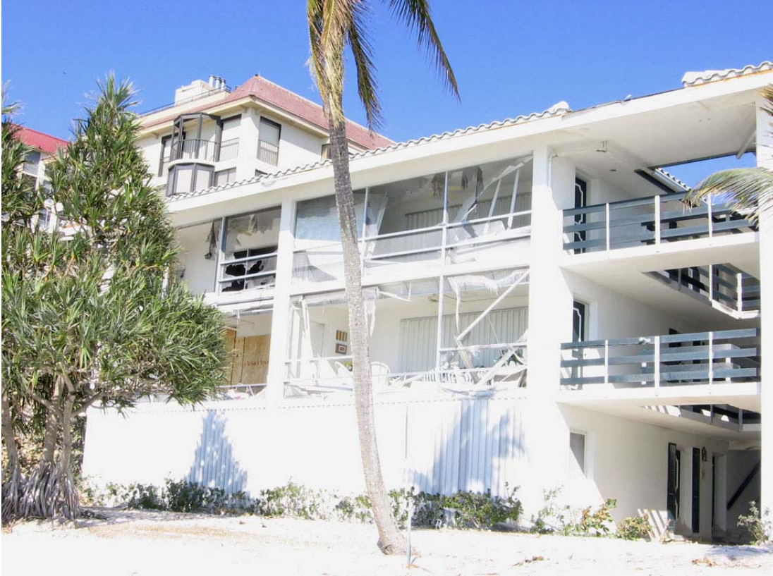
Photo 11. Wind damage to dwelling, Vanderbilt Beach (R24.1).
