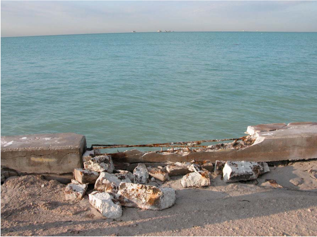
Photo 62. Concrete cap damage, Cape Florida State Park.
