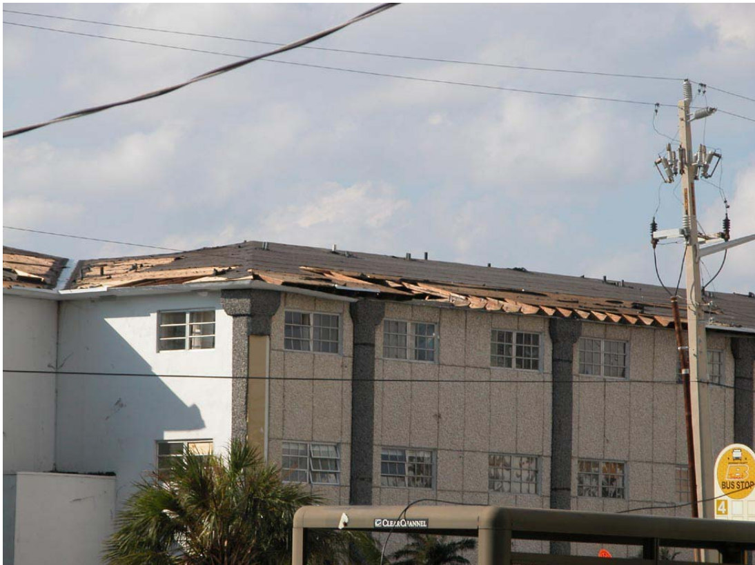
Photo 70. Major roofing damage, Hollywood (R119.8).
