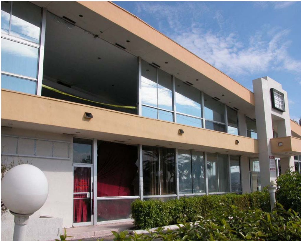
Photo 61. Broken windows, Golden Nugget Motel, Sunny Isles Beach.
