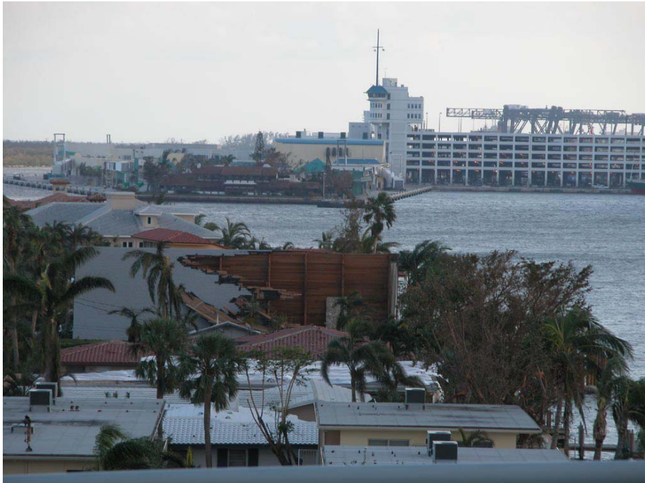
Photo 65. Major roofing damage. Fort Lauderdale.
