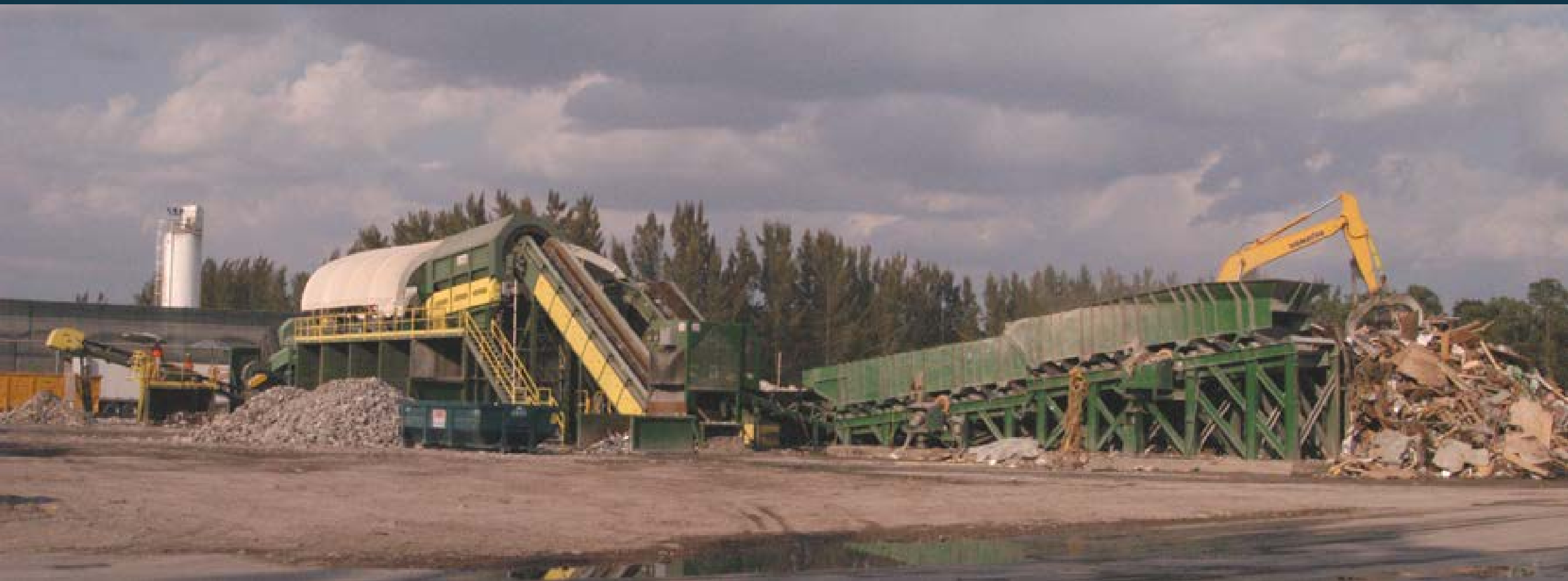
Mixed C&D Processing Facility
