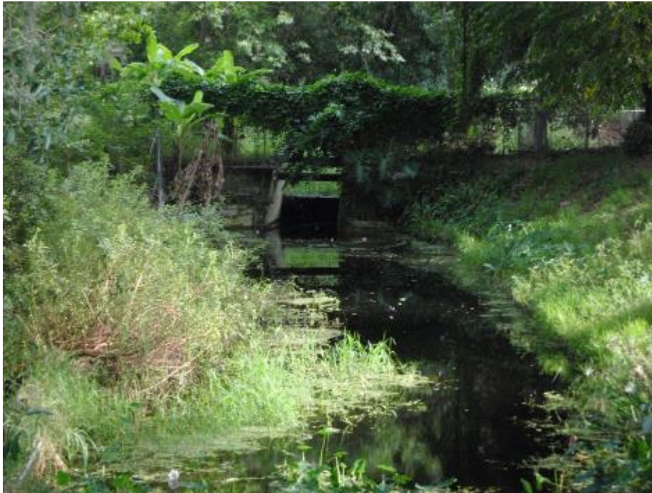
Figure 5.4 Control Structure on Mud Lake Inlet Channel.
